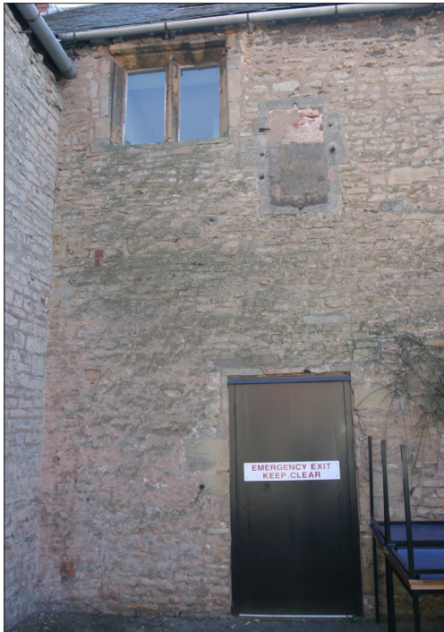
Figure 9. North side of south range, showing early 17th-century window on upper floor. Linda Monckton 04/06
