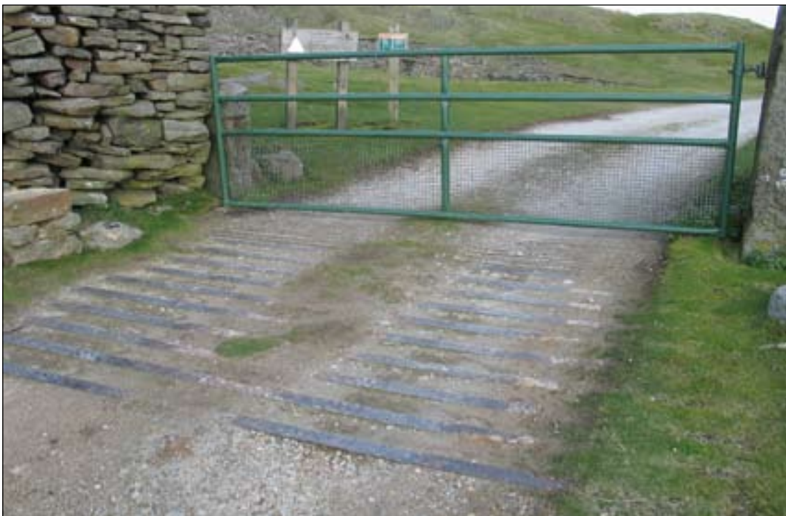
Figure 34: Example of Category 3g: miscellaneous. Cattle-grid (257) sunk into Road 1.
