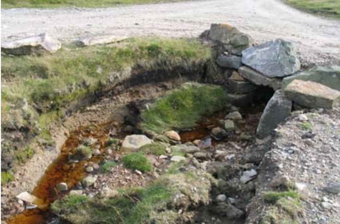
Figure 16: Example of Category 1f: culvert (170). An attempt has been made to arrest erosion by placement of boulders and stones around the historic culvert.
