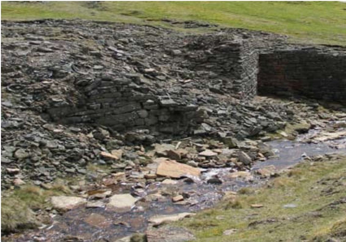
Figure 36 Example of Category 3i: collapse. Erosion along the Coalgrove Beck is causing collapse of structures (95) close to the site of the late 17th-century High Smelt Mill site.
