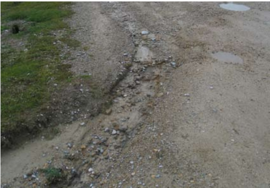
Figure 46: Gully erosion along Road 1 (8). The presence of pot-holes here may be contributing to the problem.
