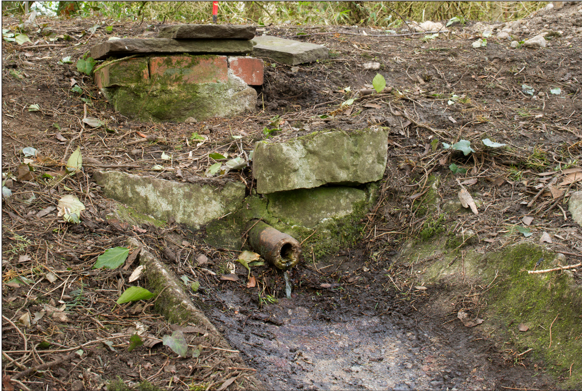
Figure 17: The brick manhole, iron pipe and concrete channel at the 'source' of the waterfall. DP168982 © Historic England/Alun Bull, 28th April 2015.
