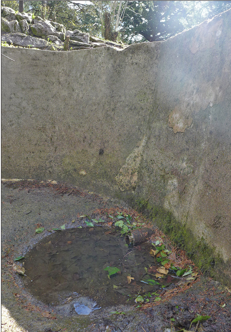
Figure 28: The dip in the top lip of the pond wall (top centre) and the inserted drainage pipe and hollow at the base of the south end of the pond (foreground), looking south-east. © Historic England/ Rebecca Pullen, 29th April 2015.
