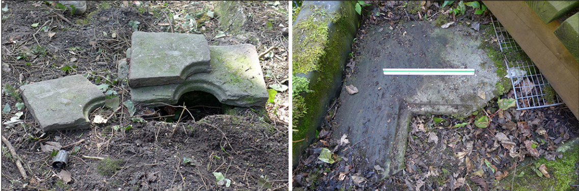
Figure 18: Surviving stone drain caps found in the garden: (left) found close to the manhole at the top of the waterfall, and (right) found close to the manhole at the end of the pond outlet. © Historic England/Rebecca Pullen, (left) 29th April 2015 and (right) 10th June 2015.
