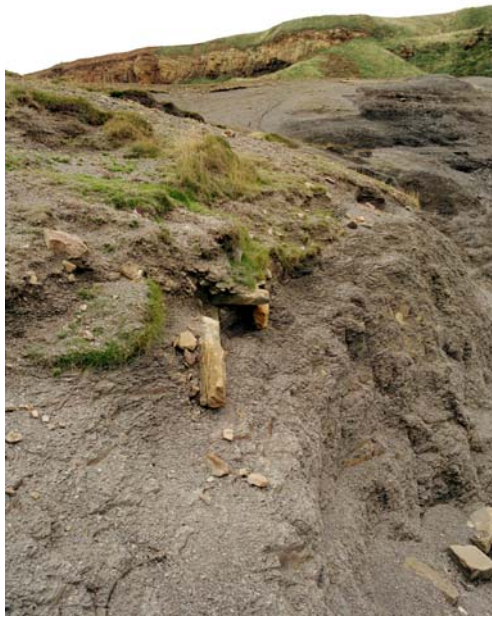
Figure 35. Detail of conduit 1 above the north-east corner of the alum- house shelf. Displaced stones overlie the scree below. (NMR AA040230)
