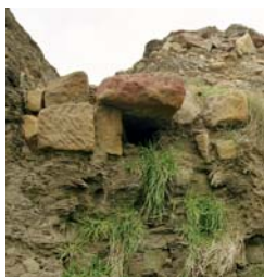
Figure 36. Conduit 2 exposed in the face of the collapsed ledge. (NMR AA040228)
