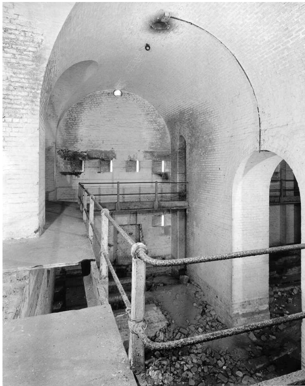
Figure 22 The interior of no 3 caponier, showing vaulting and first floor walkway (NMR: BB99/15904)
