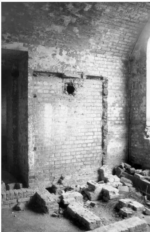
Figure 31 Remains of the stove and hot air cupboard in the Guard Room (NMR: MF99/01348/16)
