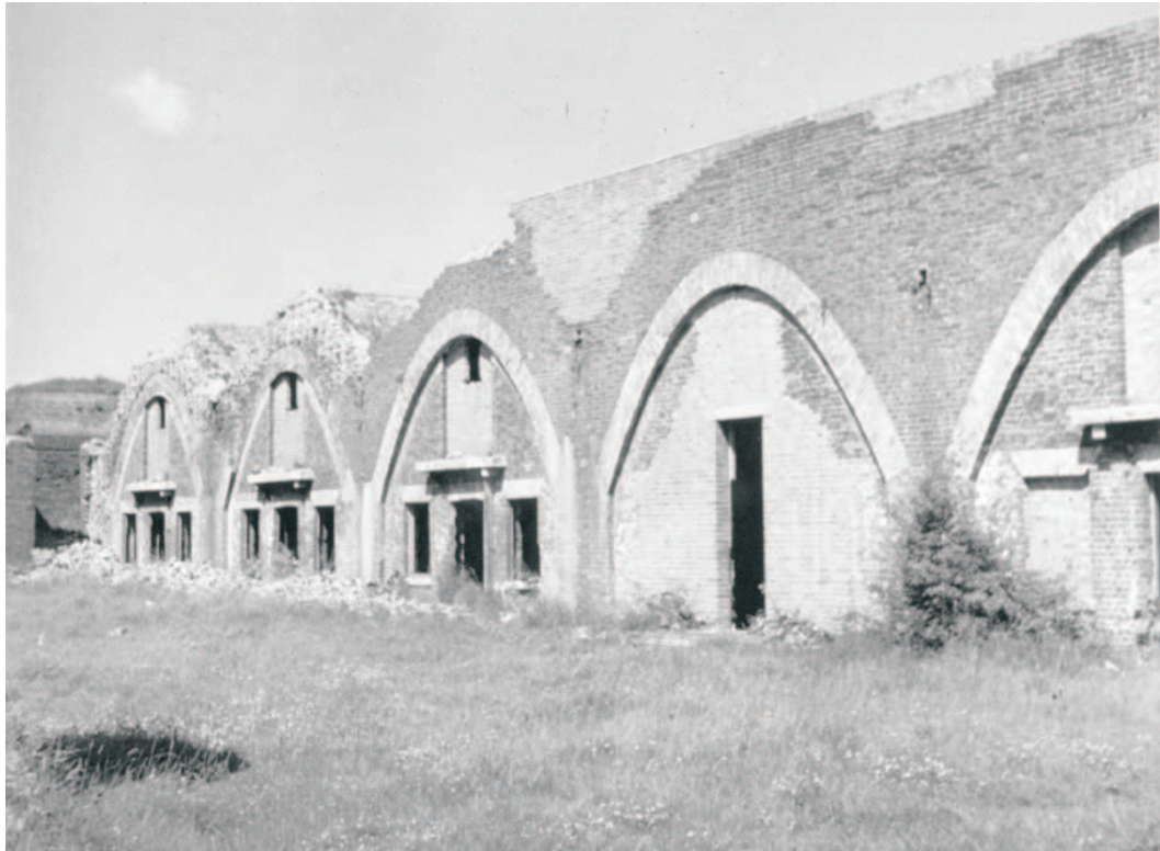
Figure 39 The Soldiers' Quarters prior to removal of the south elevation detail (Dover Museum: D07905; reproduced by kind permission of Dover Museum)
