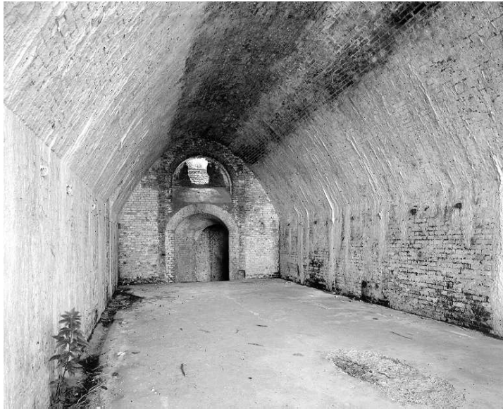
Figure 40 The Soldiers' Quarters: interior detail of casemate 4 showing parabolic vault and entrance to gallery leading to no 3 caponier (NMR: BB99/15931)
