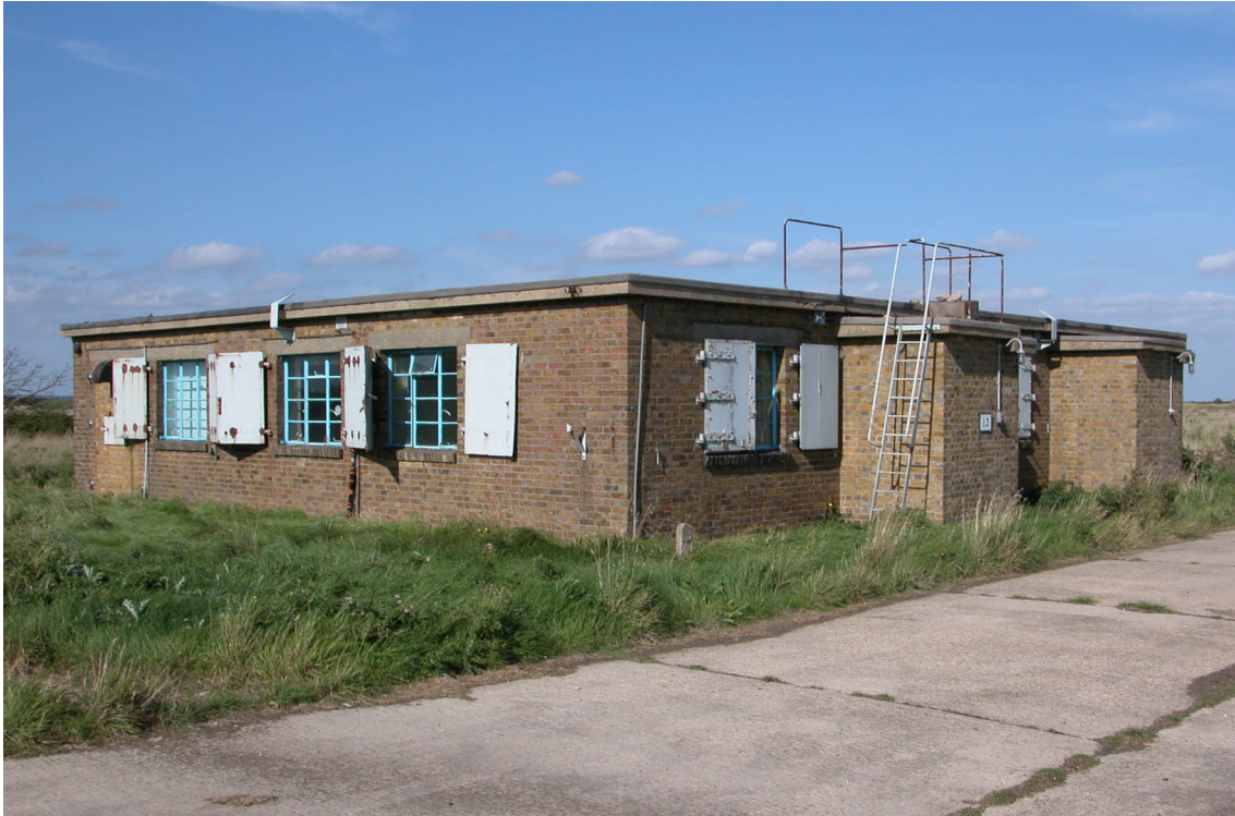
Figure 17: Office and Laboratory I3, this building is typical of the late 1940s and early 1950s range control buildings with brick walls, a flat concrete roof and steel Crittall windows protected by hinged steel shutters. (c) English Heritage
