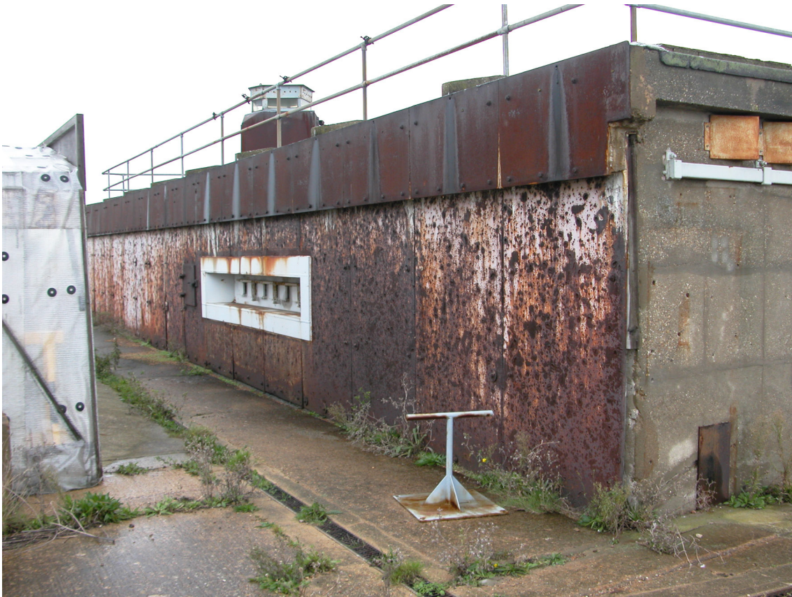
Figure 13: Fire Control Building and Instrumentation F4, showing the heavily pitted armoured steel wall facing the range, armoured observation apertures and roof turret. (c) English Heritage
