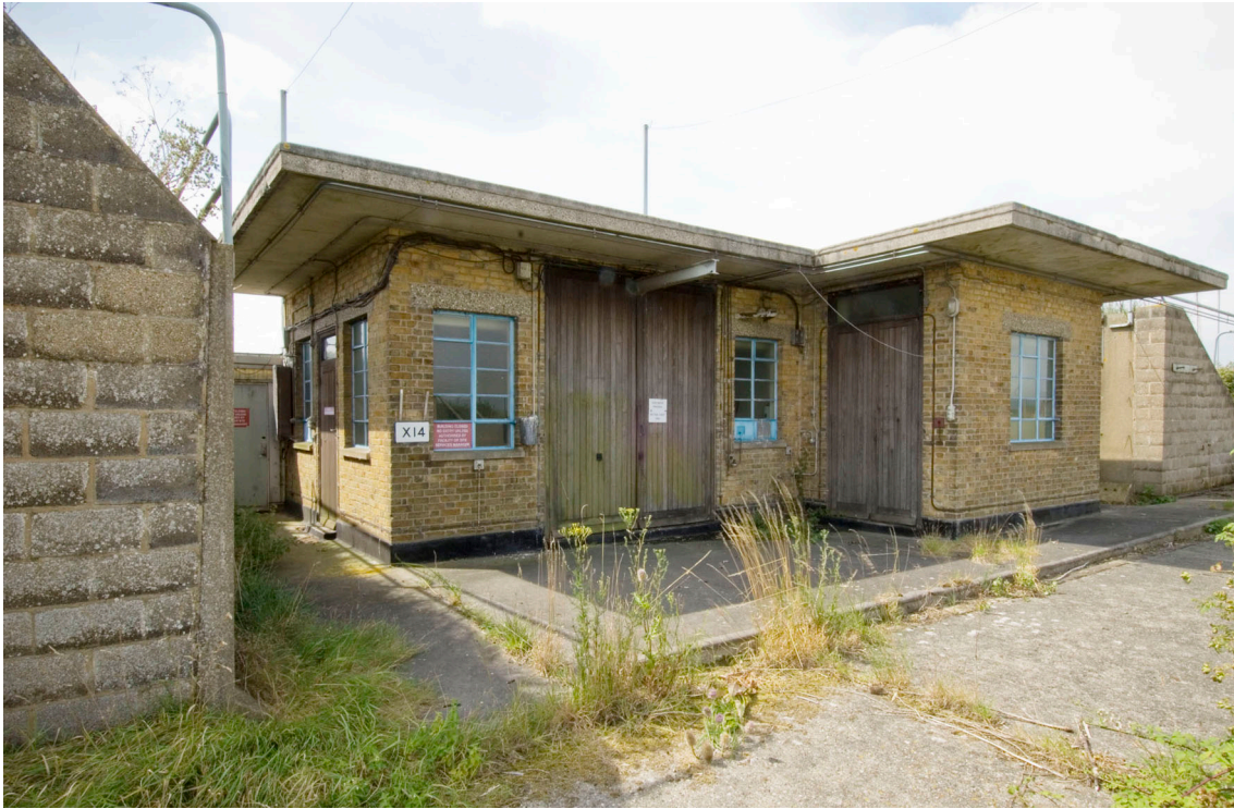
Figure 42: Explosives Machining shop X13 built about 1955, this group of buildings were distinguished by well-finished brickwork, gravel washed lintels and sills, and teak doors. To either side are later breeze block and earthwork traverses. (c) English Heritage DP035934
