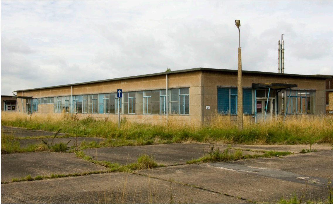
Figure 8: Laboratory LI was built in 1955 and illustrates many of the features typical of the mid-1950s pre-fabricated structures, including block panel wall construction, metal framed windows, and porch roofs supported by tubular steel arms. (c) English Heritage DP035968
