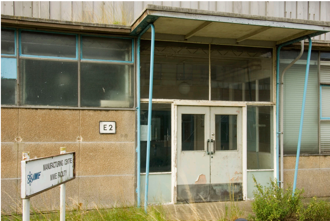
Figure 49: Main Mechanical Workshop E2, this building exhibits many features typical of the mid-1950s structures, including the hung concrete wall panels, Crittall windows, pressed aluminium sheet cladding and a porch canopy supported by a tubular steel framework. (c) English Heritage DP035959
