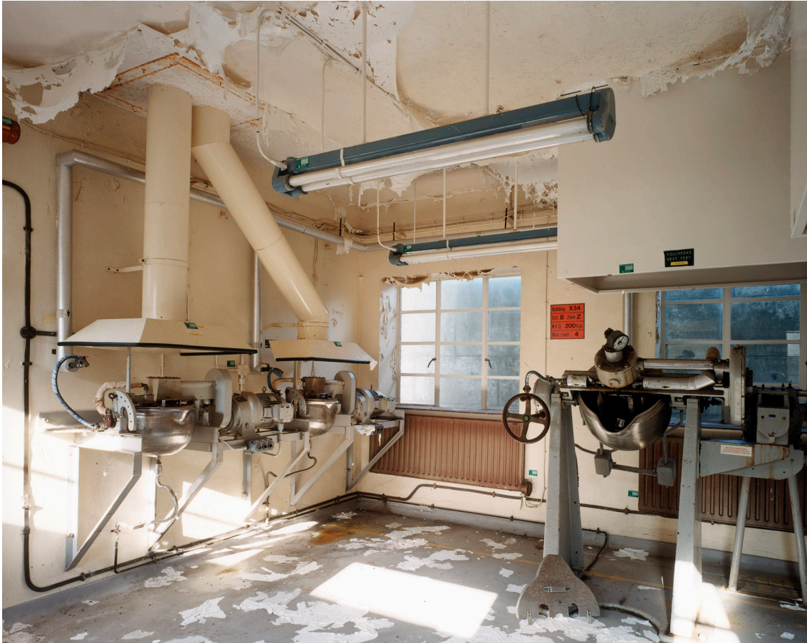
Figure 41: Casting Shop X10, was 56, showing the steam heated jacketed mixing bowls used to melt and cast high explosives. (c) English Heritage BB99/15981
