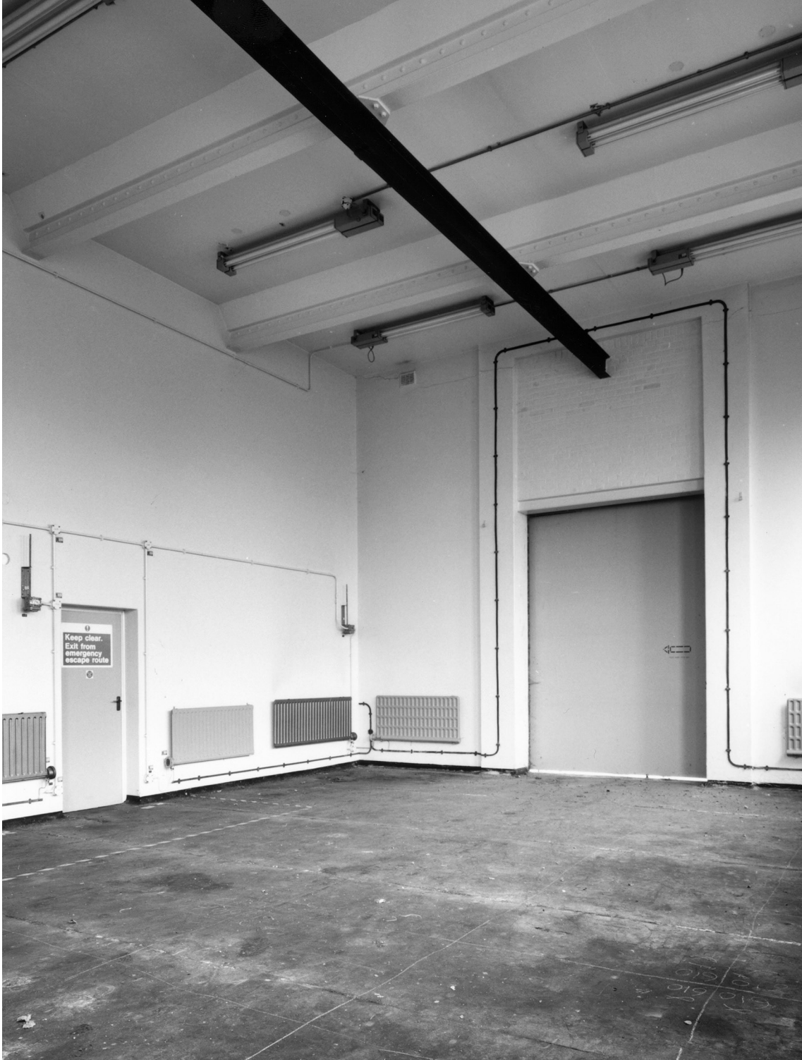
Figure 37: Building X6 was 23, Explosives Preparation Laboratories, interior of Laboratory 1 showing the main entrance door and over head lifting beam. (c) English Heritage AA99/09785
