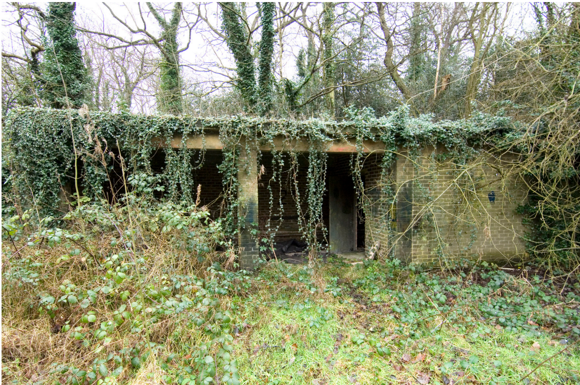
Figure 31: The rifle-range building viewed from the west. Photograph: Derek Kendall DP049806 © English Heritage
