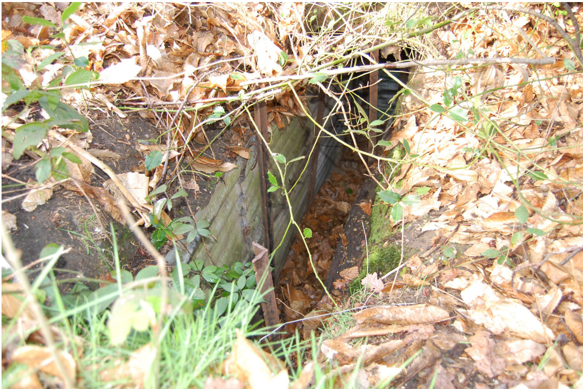
Figure 33: The entrance to the narrow buried trench which probably dates to the Second World War. Photograph: Sarah Newsome 2008 © English Heritage
