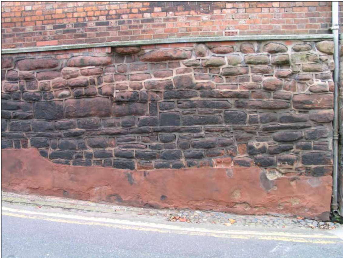
Figure 44: Early masonry underlying range along Souter's Lane (© Historic England, photograph: Adam Menuge).
