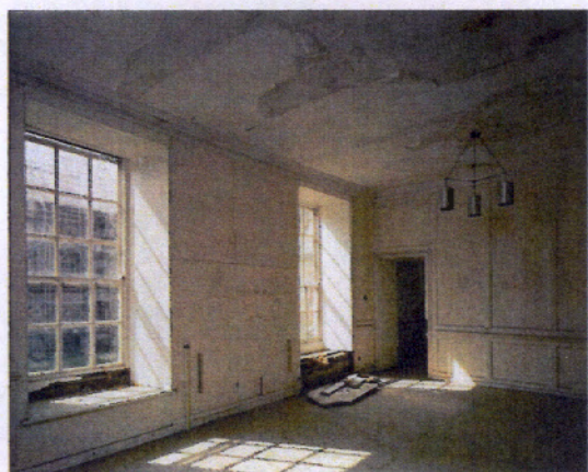
Figure 7.42 The eastern panelled room in the North Lodging Block. © English Heritage BB039799
