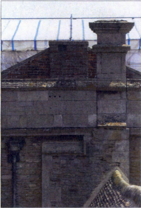
Figure 7.31 The altered chimney stack on the west side of the Gate Tower. Pete Smith 2006
