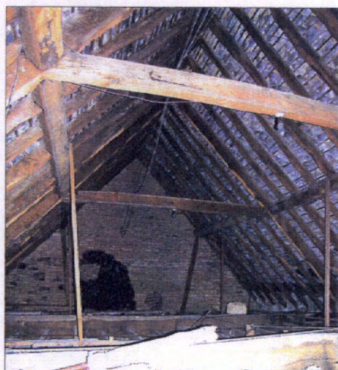
Figure 7.17 The Kitchen roof showing the smoke-blackened scar of the former chimney stack.
