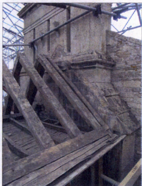
Figure 7.30 The altered Long Gallery roof showing how it abuts the chimney stack to the east of the Devil's Stair.
