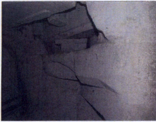
Figure 7.5 The missing step on the spiral staircase in the Gate Tower.
