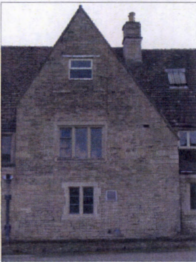
Figure 7.21 The single gabled projection on the north front of the Service Block.
