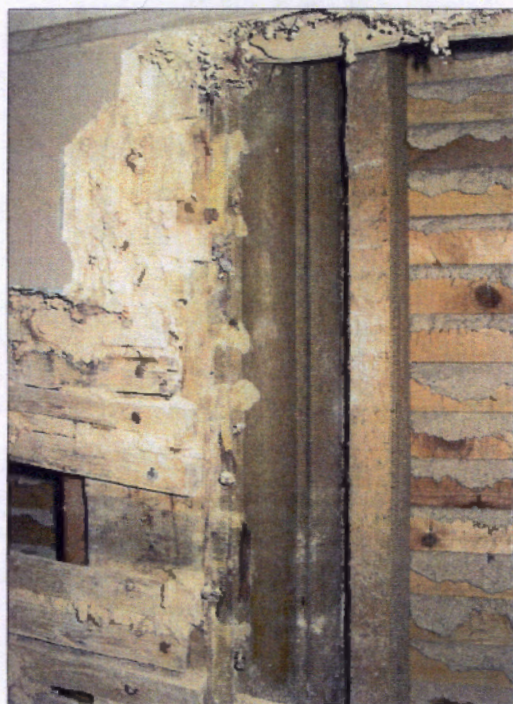
Figure 10.11 Recently uncovered jamb of doorway leading from the Duke's Closet to King's Chamber. Kathryn Morrison 2006
