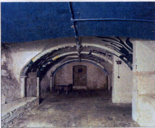
Figure 10.8 Cellar under south end of east range, looking south towards blocked doorway. © English Heritage BB039787
