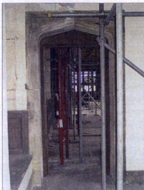
Figure 10.19 Original doorway to Long Gallery, from south, showing scaffolding in place in 2005-2006 to protect the ceiling. Kathryn Morrison 2006
