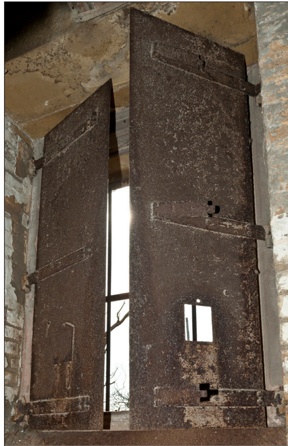
Figure 25: The iron loopholed shutters in one of the barrack rooms [46]. Note the hinged cover over the loophole at the bottom of the left-hand shutter and the locking hasp on the centre hinge of the right-hand shutter. (DP 097506)
