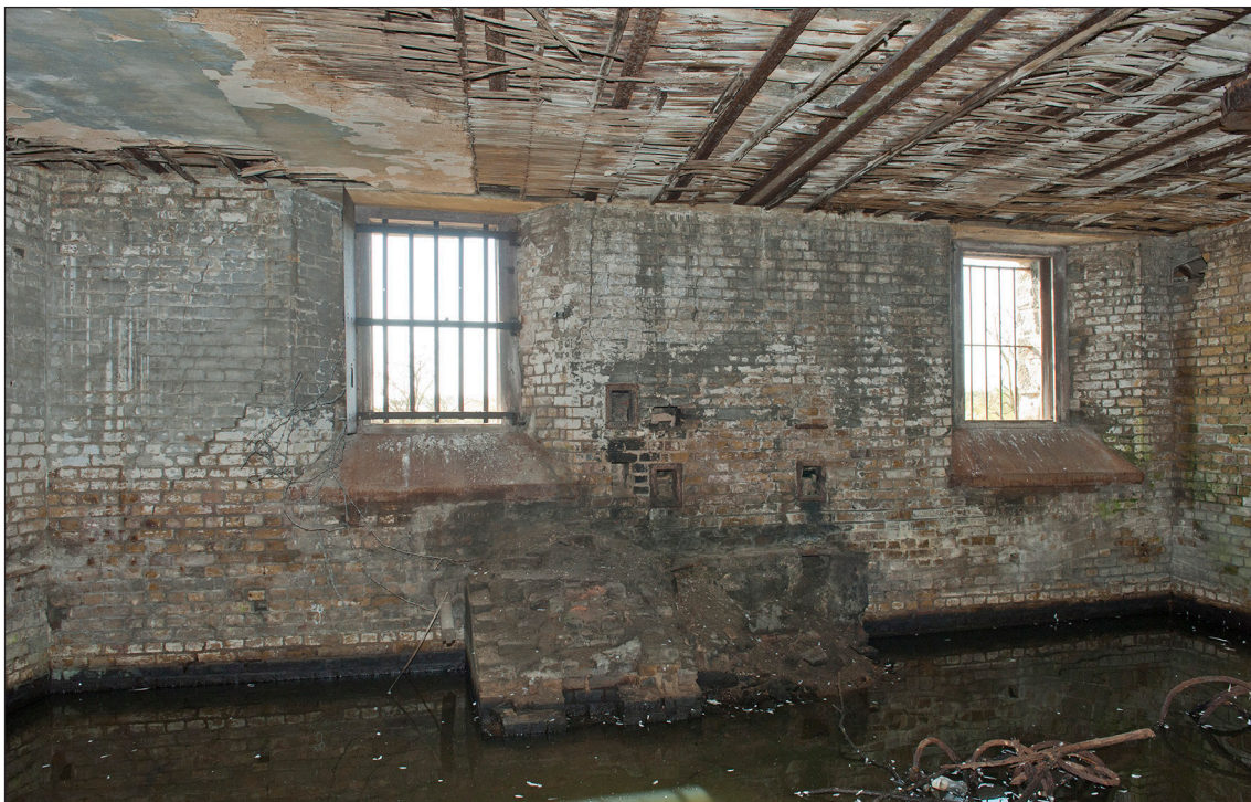
Figure 37: The brick bases for the washing coppers on the south wall of the Wash House and Laundry. (DP097511)
