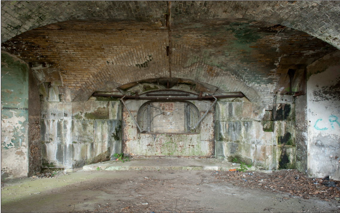
Figure 18: Interior of Casemate 4 looking towards the shield and embrasure. Note the two cheek pieces to the shield face, two sets of mantlet bars and the granite base at the foot of the shield. Just visible flanking the casemate are the edges of the later concrete traverses filling the gun positions of casemates 3 and 5. (DP097600)
