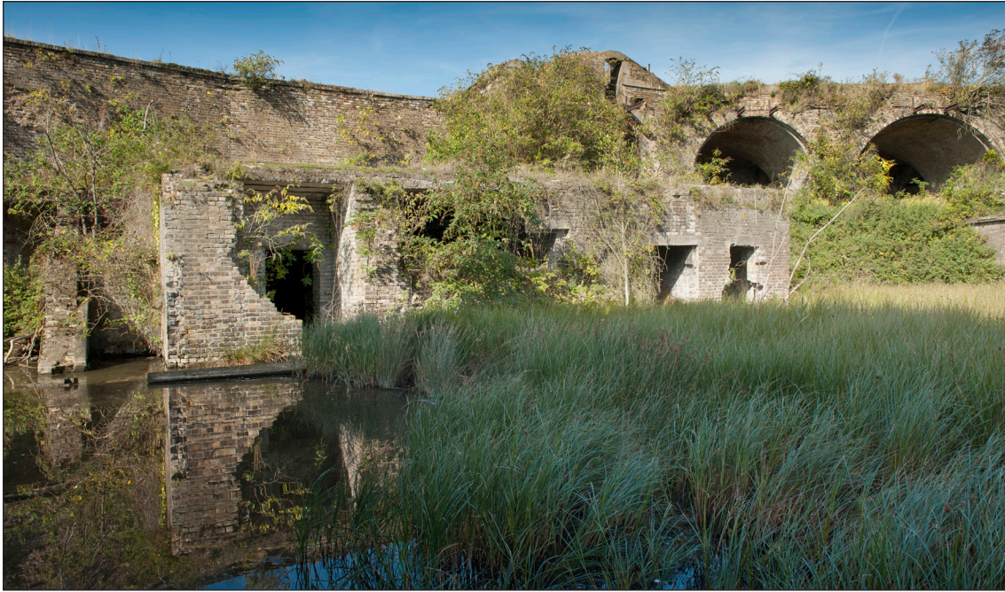
Figure 15: The former Laboratory [61], later converted to the entrance and stores for the Brennan installation. Above and behind is the traverse at the rear of the open battery. Casemate 15 is to the right with the back of the Brennan observation post above it. (DP097566)
