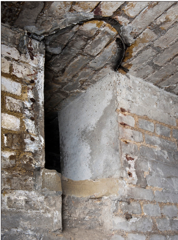
Figure 14: Inserted opening for No 16 light box at the springing of the shifting passage vault. The witness marks shows the position of the cover. The glass pane was set in the foot of the opening below the sandstone sill. (DP097437)
