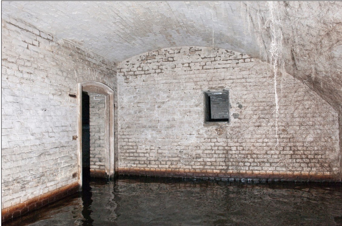
Figure 10: Interior of No 5 Spare Shell Store [92] which retains the plan and appearance of the ammunition stores as built. Note the light box in the rear wall and the sturdy timber door-frame with pegged joints and retained by noggins set in the brickwork. (DP097445)
