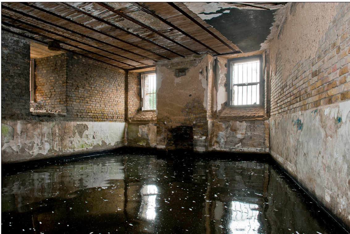
Figure 29: The interior of the Officers' Mess Room [37]. The remains of decorative plasterwork can be seen on each corner of the chimney breast and on the lower portion of each wall. Patches of ceiling plaster still adhere to the laths infilling the Fox and Barratt type roof. The iron shutters and their sills have been removed from each window opening. (DP 097470)
