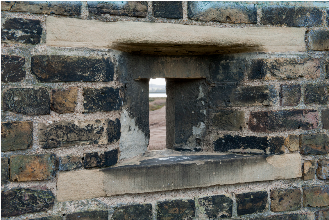
Figure 24: The interior of a loophole in the southern face wall of the fort. (DP 097575)
