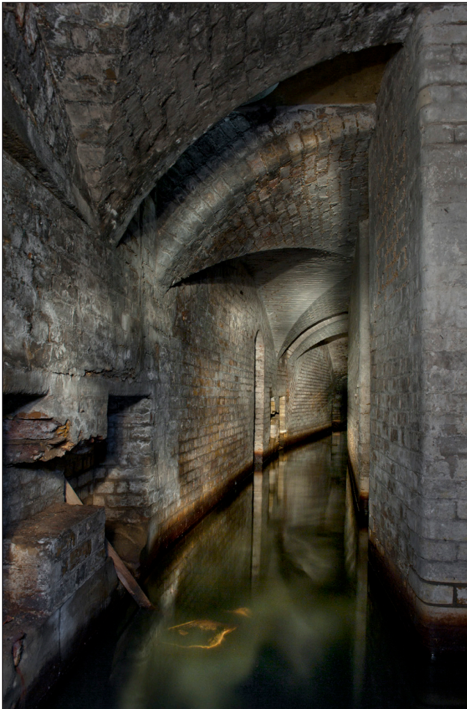
Figure 8: The shifting passage looking north-east. At the base of the wall on the left side of the picture are the recesses for the ammunition lift winches. Located out of shot to the right are the end walls of the ammunition stores. A shaft for the ammunition lift rises from the recess at the top of the vault. The arched headed opening in the middle distance is the blocked entrance to the demolished caponier. (DP097444)
