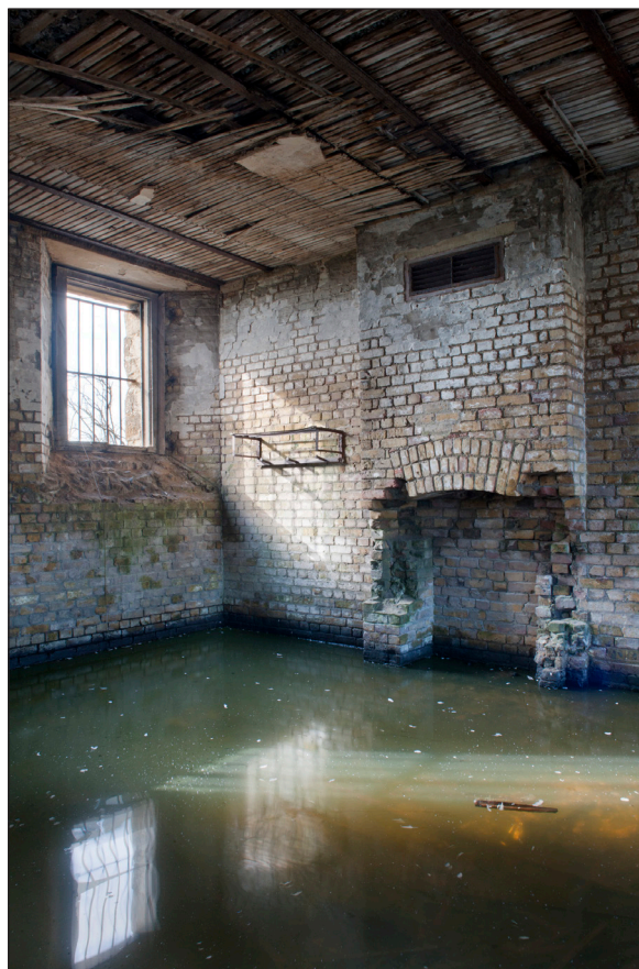
Figure 34: The interior of a Barrack Room intended for nine men [45]. The vent above the fireplace and the equipment rack set midway up the wall to the left of the chimney breast are visible. The iron shutters and the accompanying sill have been removed from the window. (DP 097489)
