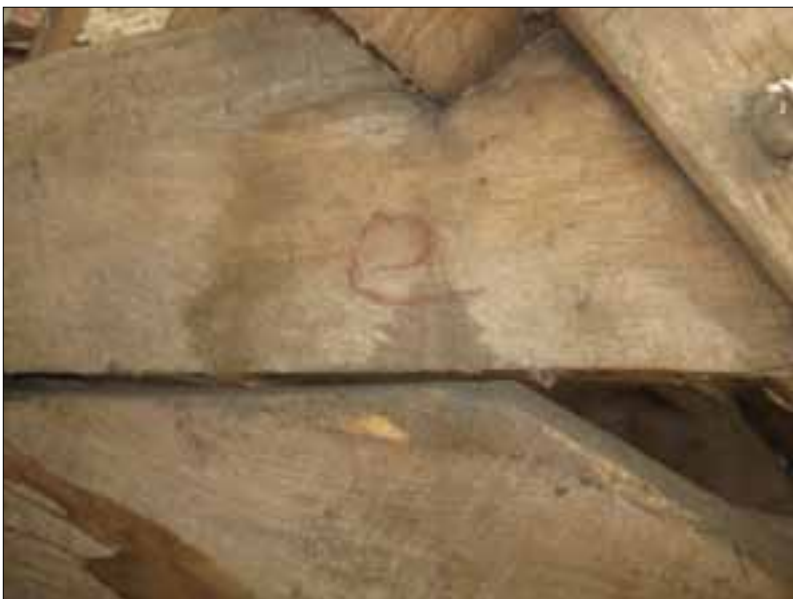
Fig 2.3 Close-up of red carpenter's mark to roof over H2.10/2.12.
