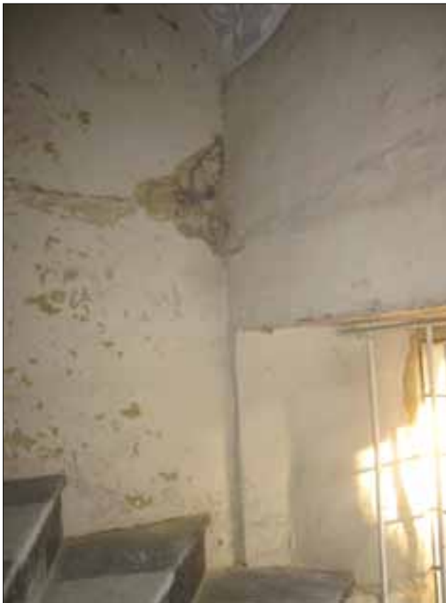
Fig 9.3 Junction of south and east walls to S3.04 – stair at second floor.
