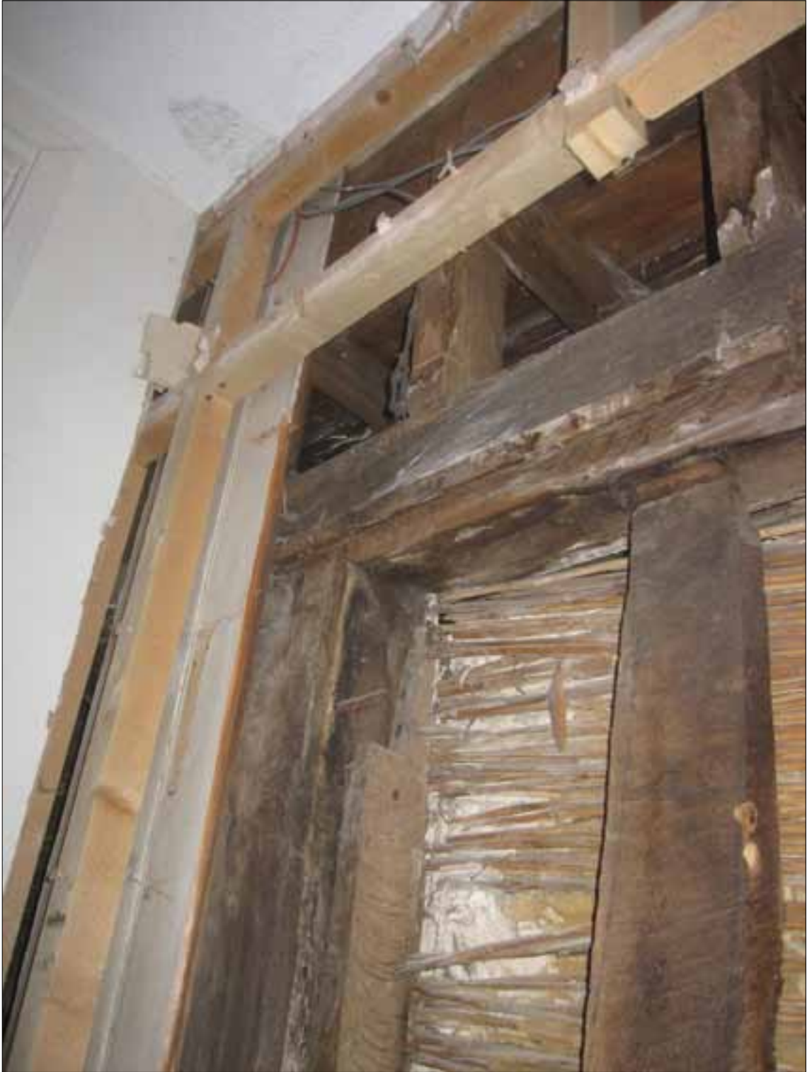
Fig 8.5 West wall of H2.16, central post, with stud set back from face.
