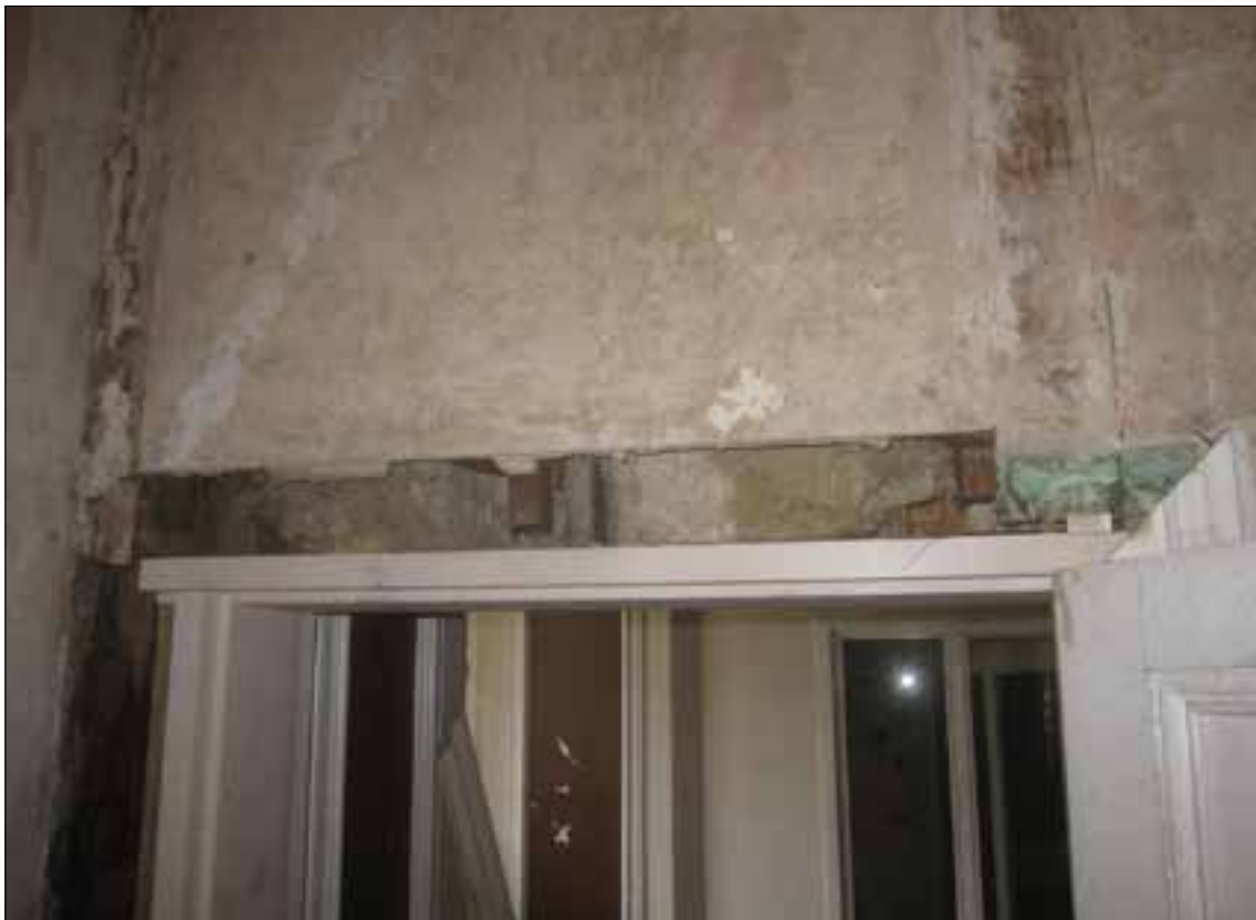
Fig 3.4 Partition over the head of the doorway, with oak studs and mud infill panels.
