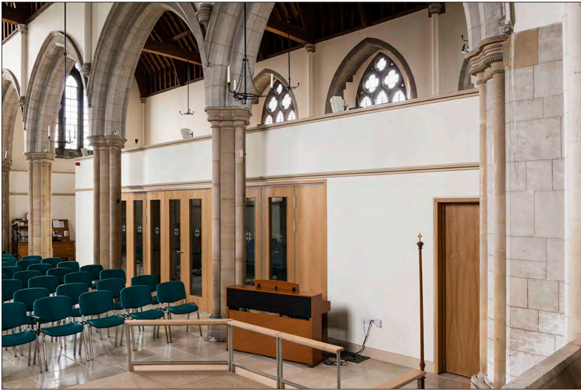
Figure 42: The transformed north aisle at the Church of All Saints, Highcliffe (DP172530 © Historic England, photograph: James O Davies)
