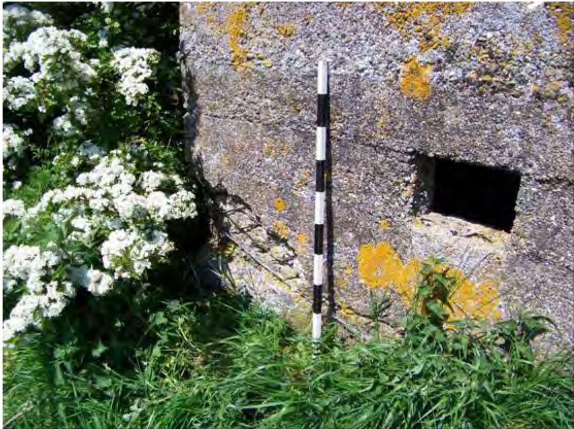
Plate 59 Detail of SK50, showing exposed reinforcement in wall and at base of embrasure (1m scale)
