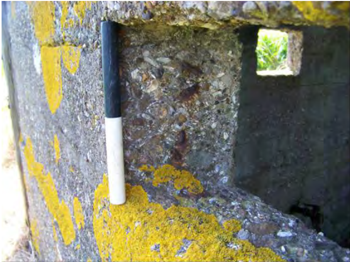
Plate 31 Detail of embrasure, BA30, showing bent ends of reinforcing mesh (0.2m scale)
