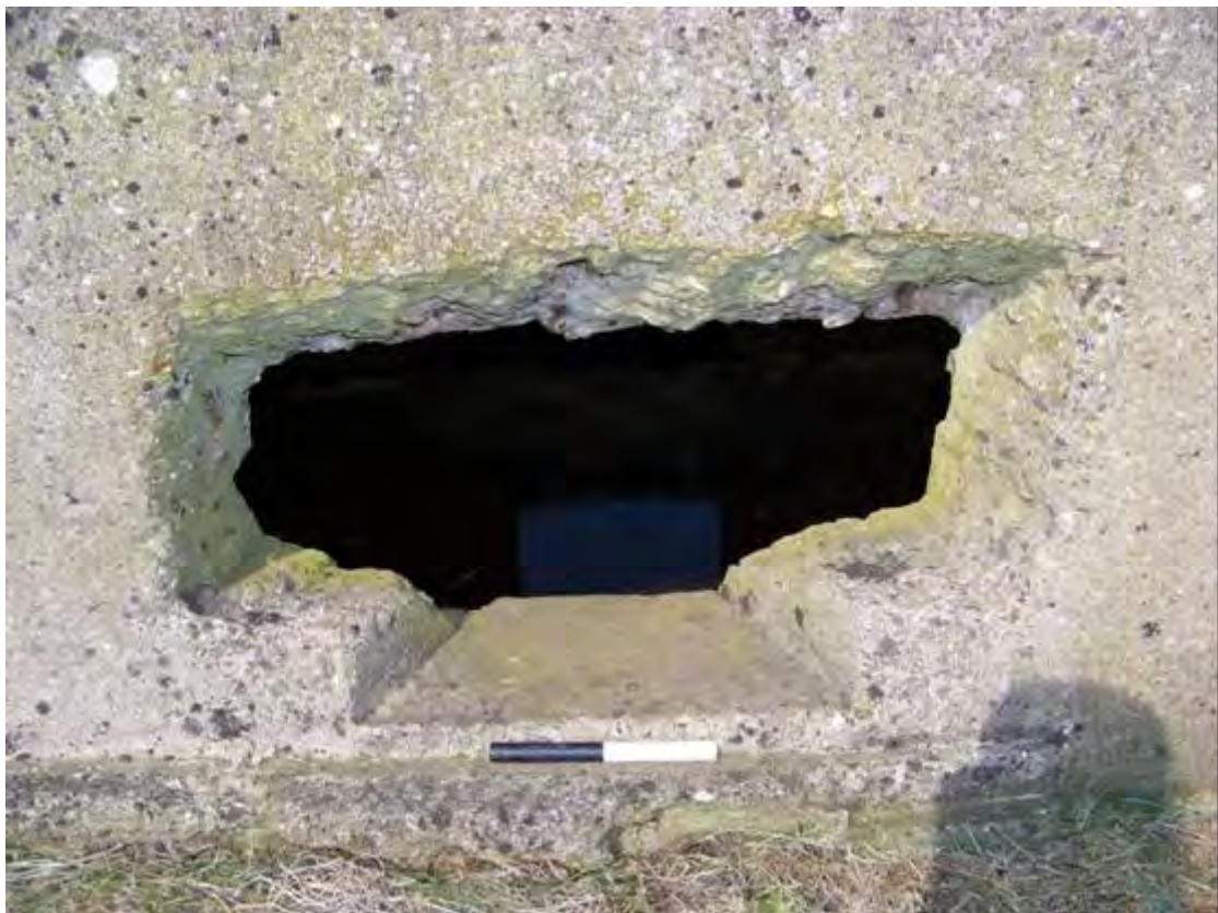
Plate 8 Detail of central Second World War embrasure of BA10, enlarging original splayed loophole. Traces of reinforcing bars visible at top of opening (0.2m scale)
