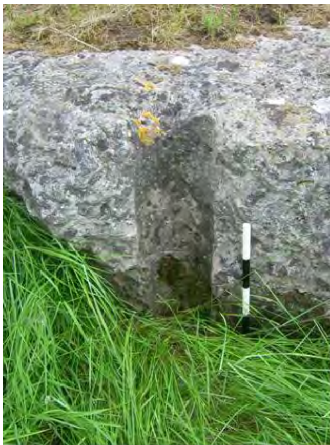
Plate 76 Detail of vent pipe through fracture of NS74 roof slab (0.5m scale)
