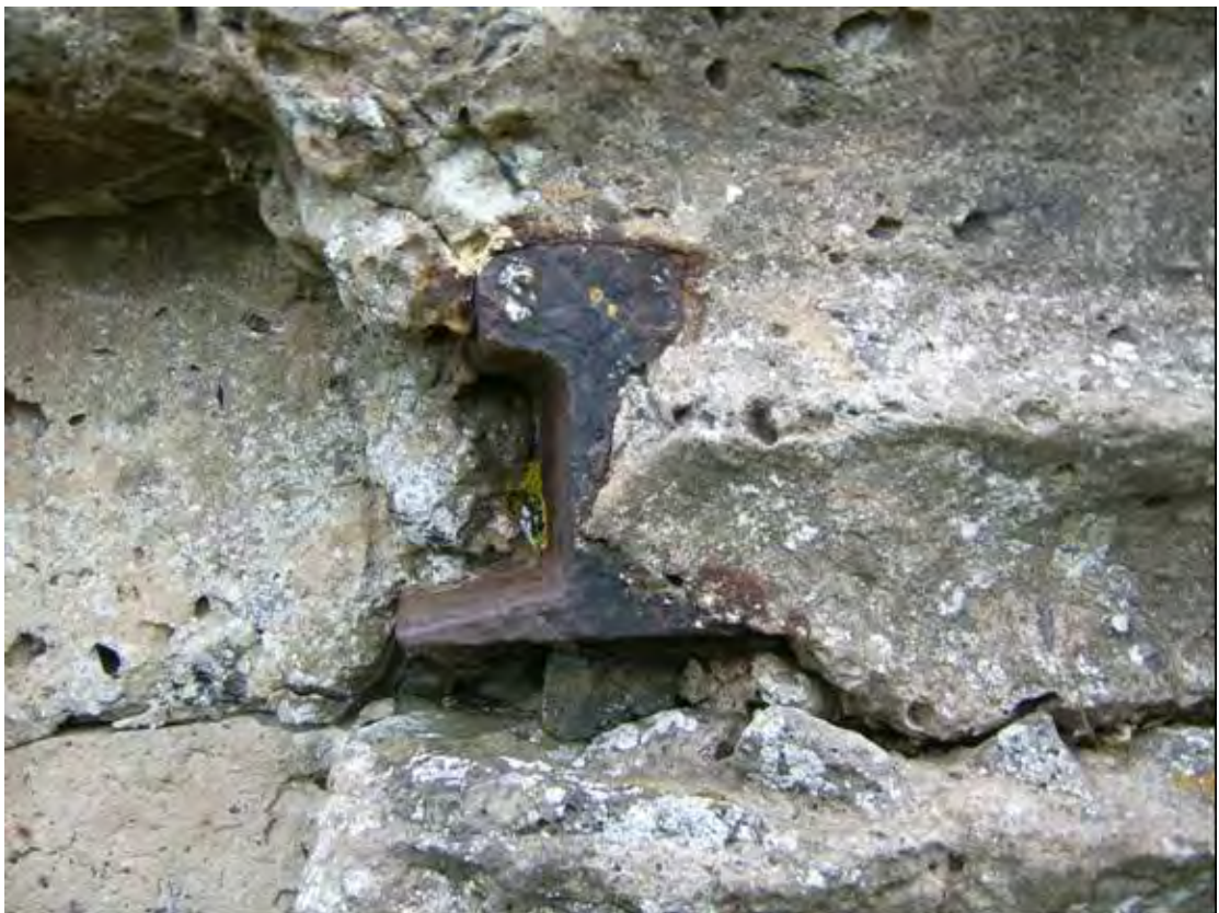
Plate 84 SH1, detail of exposed end of steel reinforcement beam
