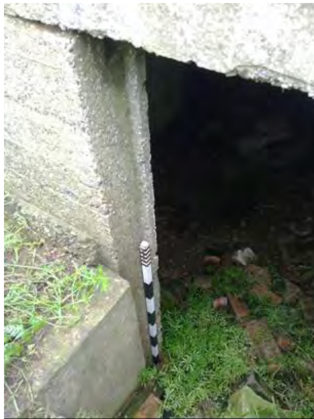
Plate 66 Sunken entrance to AT24, showing rebated doorway and sidewalls of entrance passage (1m scale)
