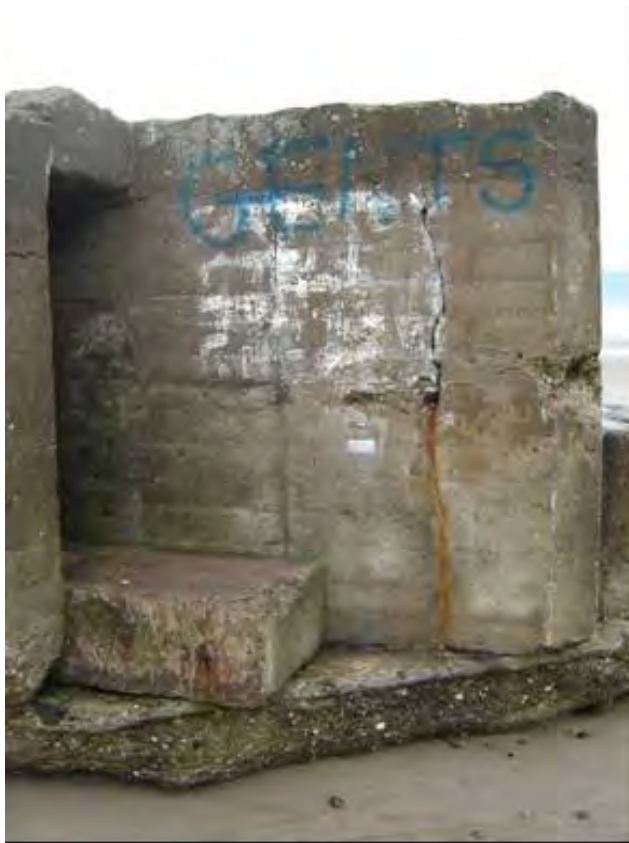
Plate 131 Second World War eared pillbox CY5 showing condition of eastern side in 2008, with blast wall still in situ
