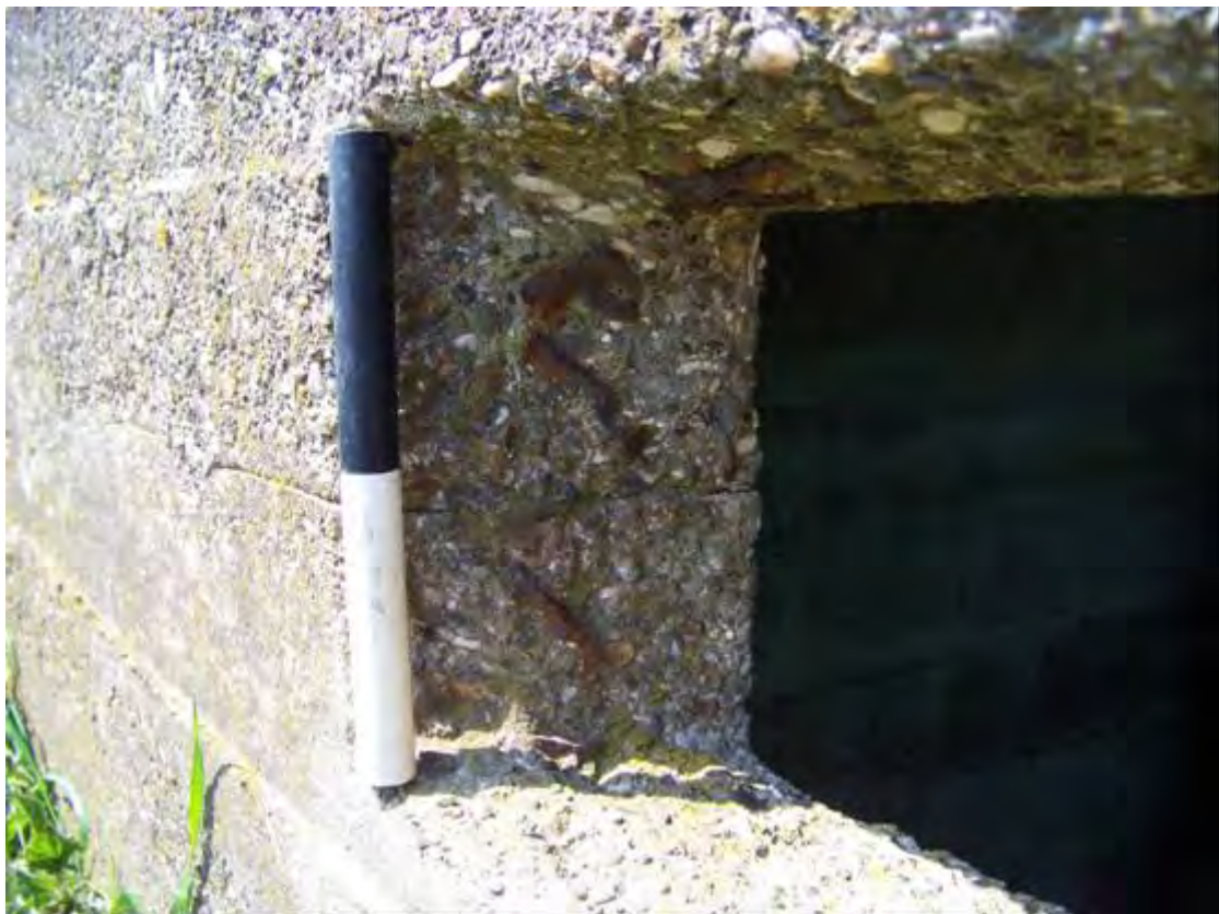
Plate 32 Detail of embrasure, BA30, showing exposed reinforcing mesh and distinct division between concrete pours (0.2m scale)
