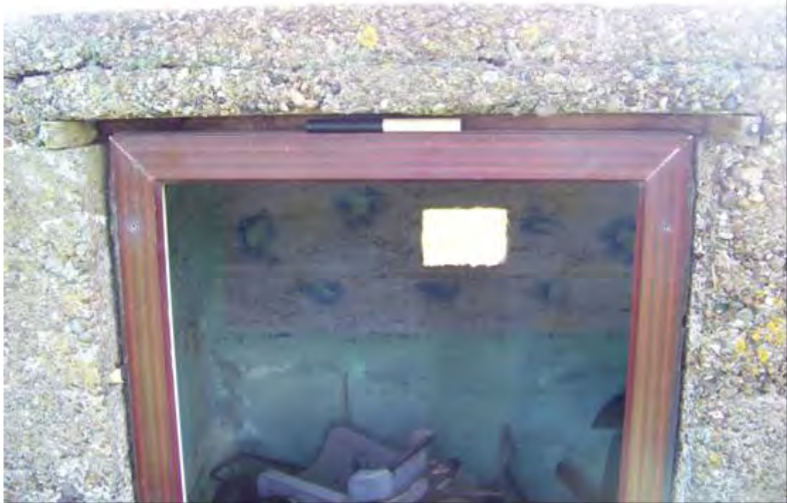
Plate 29 Detail of modern frame inserted in doorway of southern pillbox, BA30, showing slot for original wooden lintel (.2m scale)
