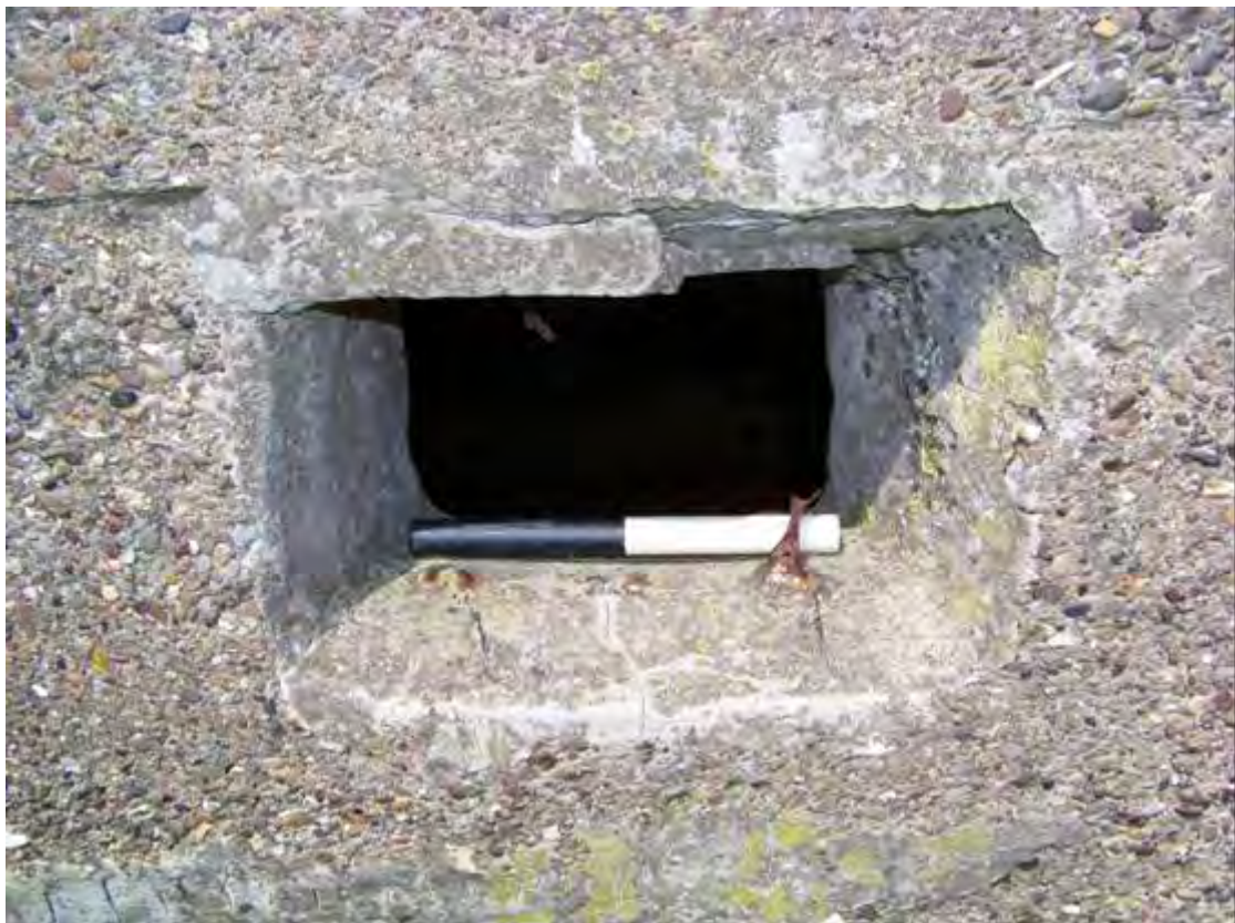
Plate 16 Detail of embrasure cut through wall of BA19 and mesh reinforcement after casting, cement smoothing around opening has partly fallen away (0.2m scale)
