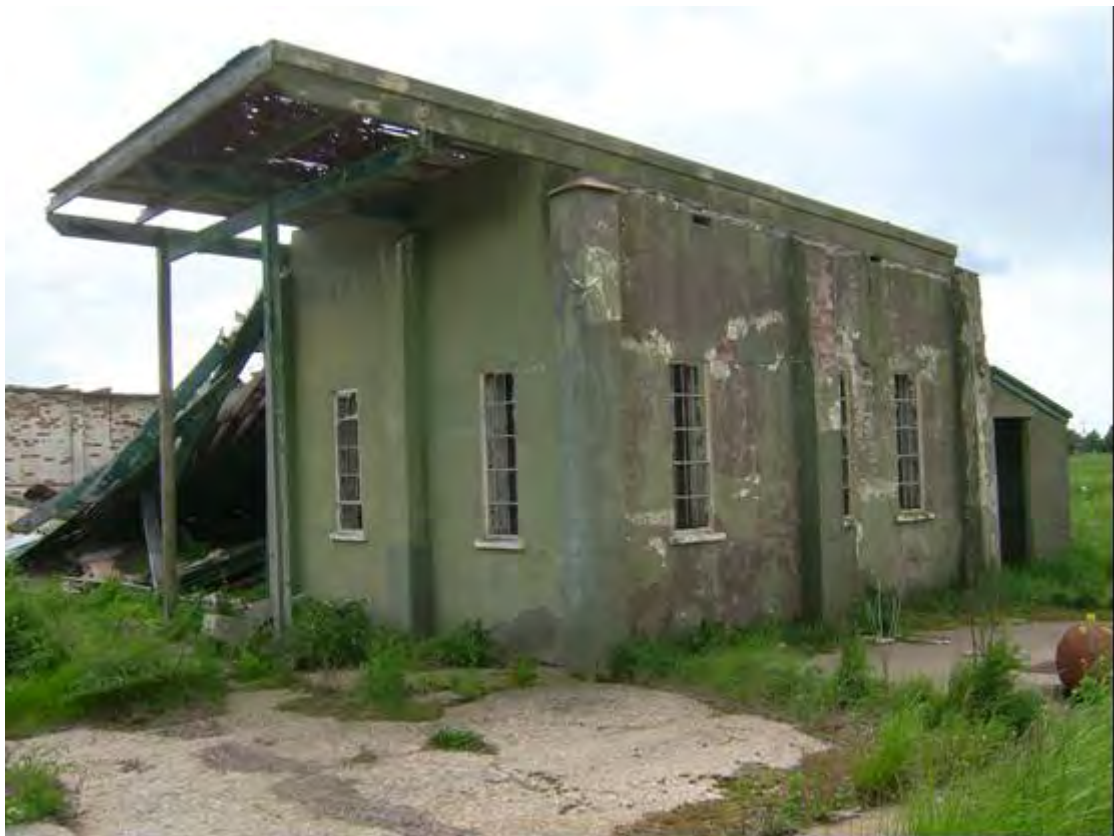
Plate 194 RAF Theddlethorpe, north end block of turret maintenance building, looking south-west, showing collapsed verandah (left) and lean-to (right)
