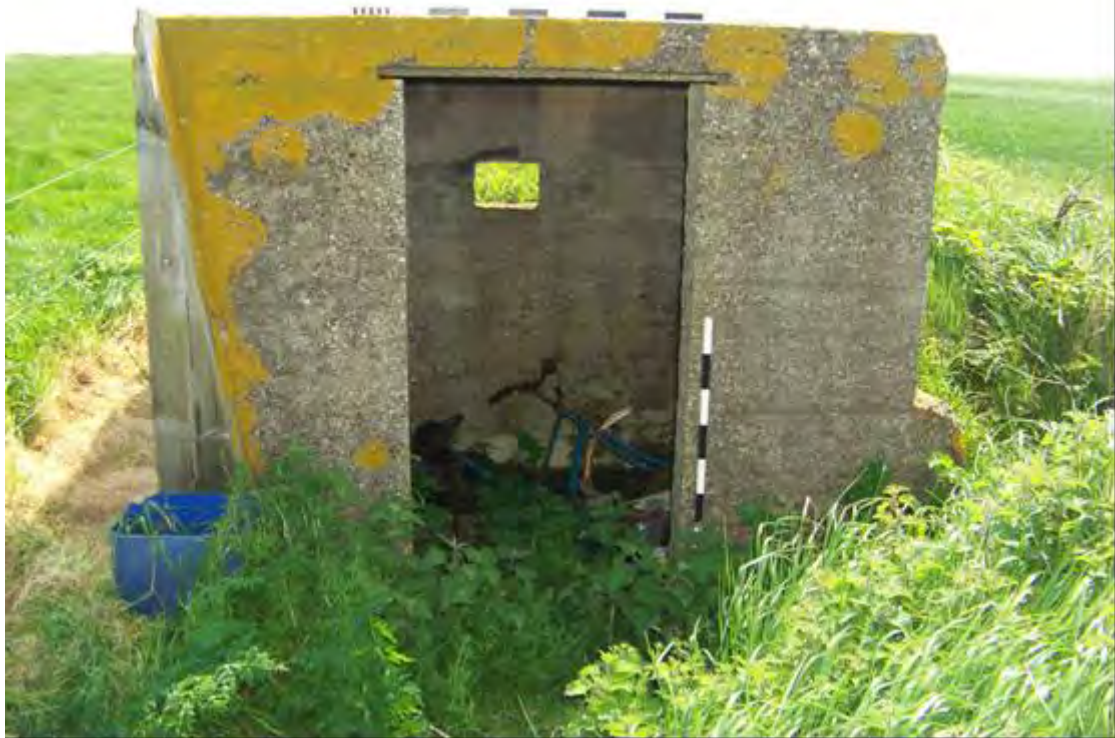
Plate 27 Detail of west wall of northern pillbox, BA30, showing wooden lintel and thickness of roof slab (2 x 1m scales)
