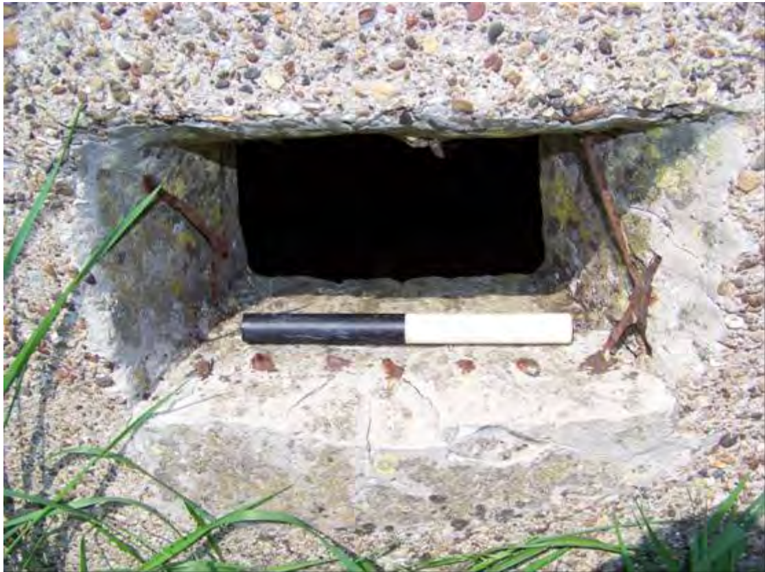
Plate 15 Detail of embrasure cut through wall of BA19 and mesh reinforcement after casting, clearly showing cement smoothing around opening (0.2m scale)
