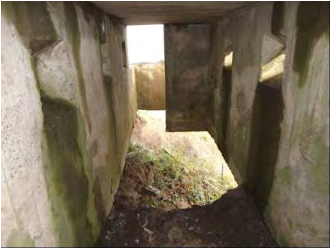
Plate 105 Second World War section post FD60, missing floor at the seaward (NE) end of the post
