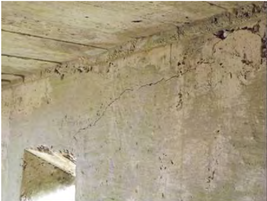
Plate 106 Second World War section post FD60, Hairline crack leading from the gun loop to the angle of the ceiling
