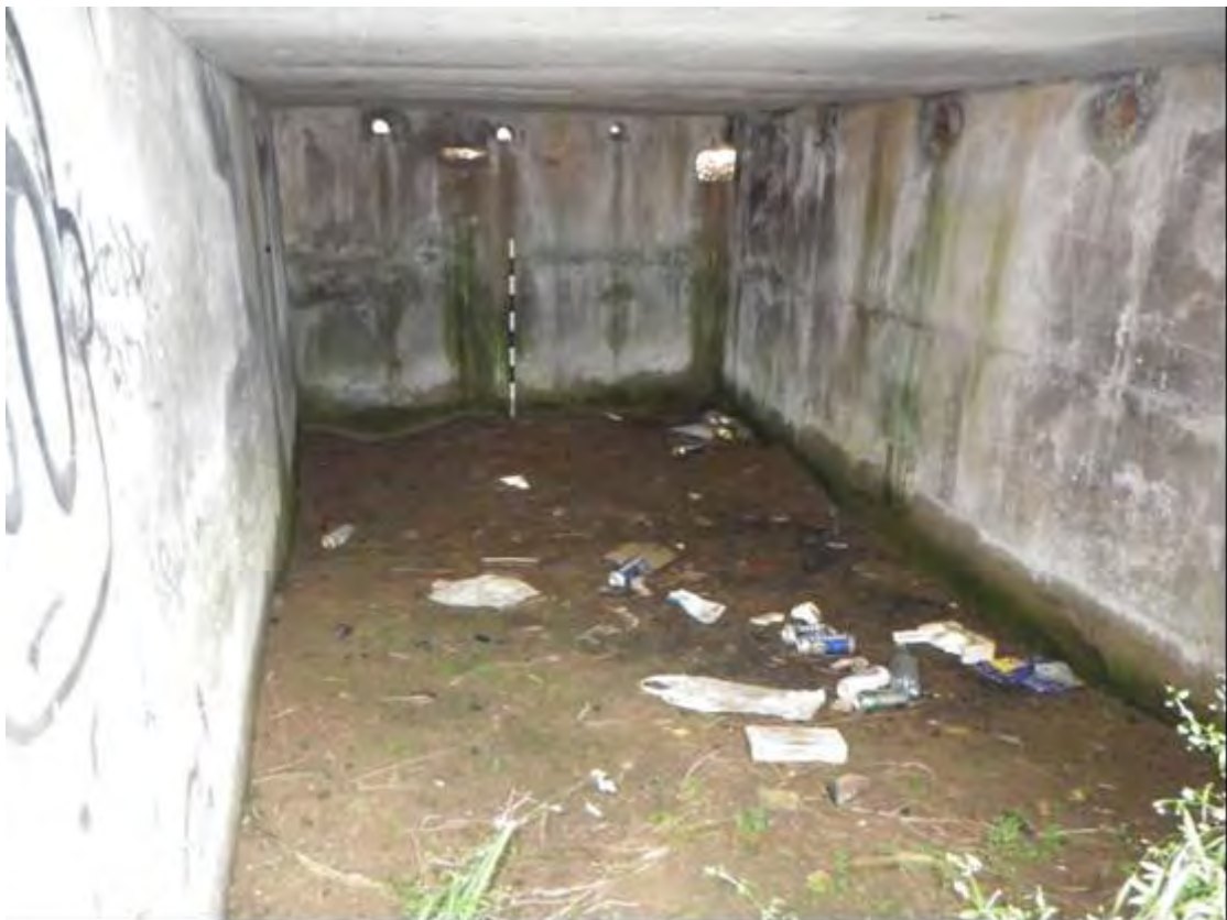
Plate 168 AT58, interior of southern room, showing wall vents and small later openings cut through upper east wall
