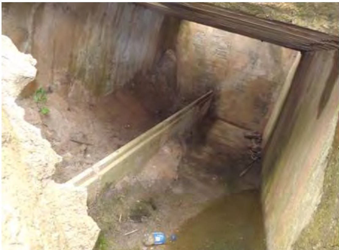
Plate 123 Second World War section post CY9, reinforced concrete shelf running along the inner face of the forward wall, looking west with the light shining down the access stairs to the upper side of the image
