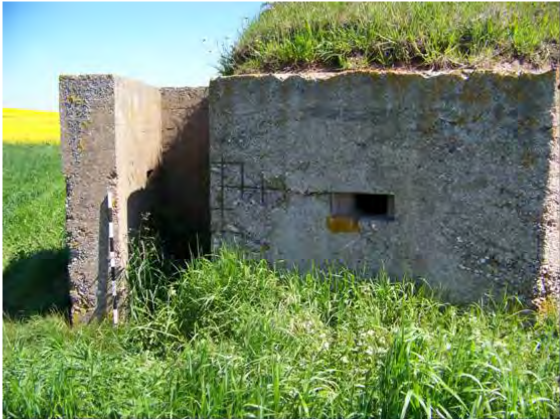
Plate 137 Second World War lozenge pillbox BA104, showing details of blast wall with embrasure protecting rear entrance, and exposed reinforcing mesh (1m scale)
