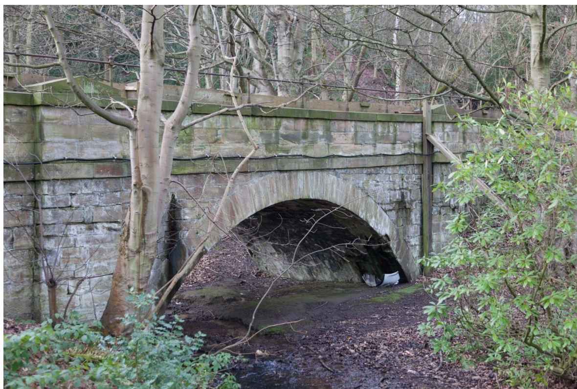
Figure 4.2: Listed bridge in poor condition
