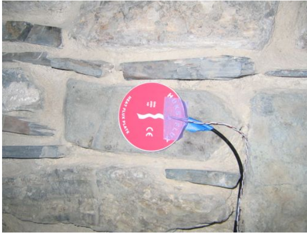
Figure 1. Heat Flux Sensor and surface temperature thermocouple.
