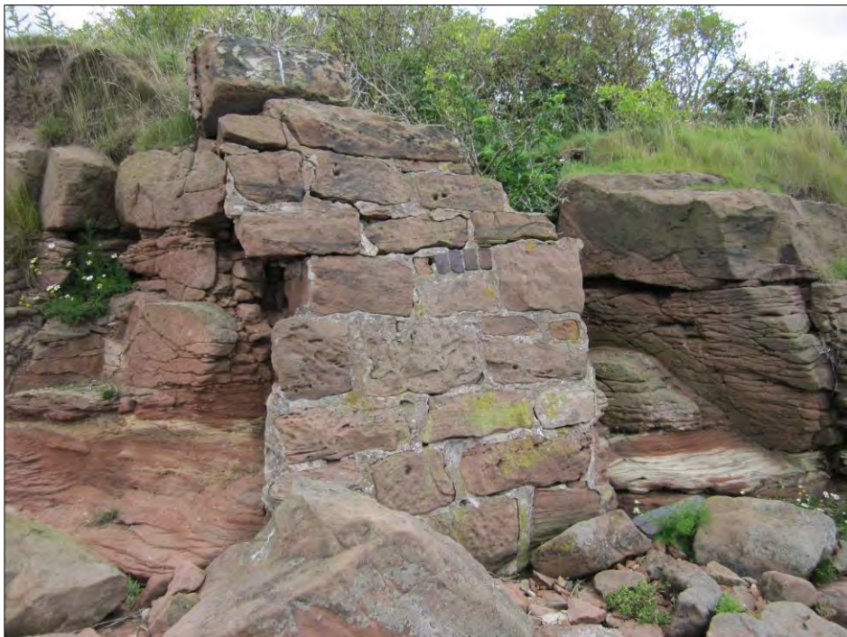
Figure 2.19 Failing Victorian defences on the north and north-west end of Stanlow Point (© Robert Edwards, Cheshire West and Cheshire Council)
