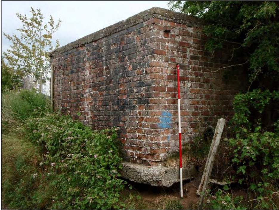
Figure 2.7 Bombing decoy control building on the edge of Burton Marsh. Note ground erosion at the base that may lead to subsidence (scale = 2m).
