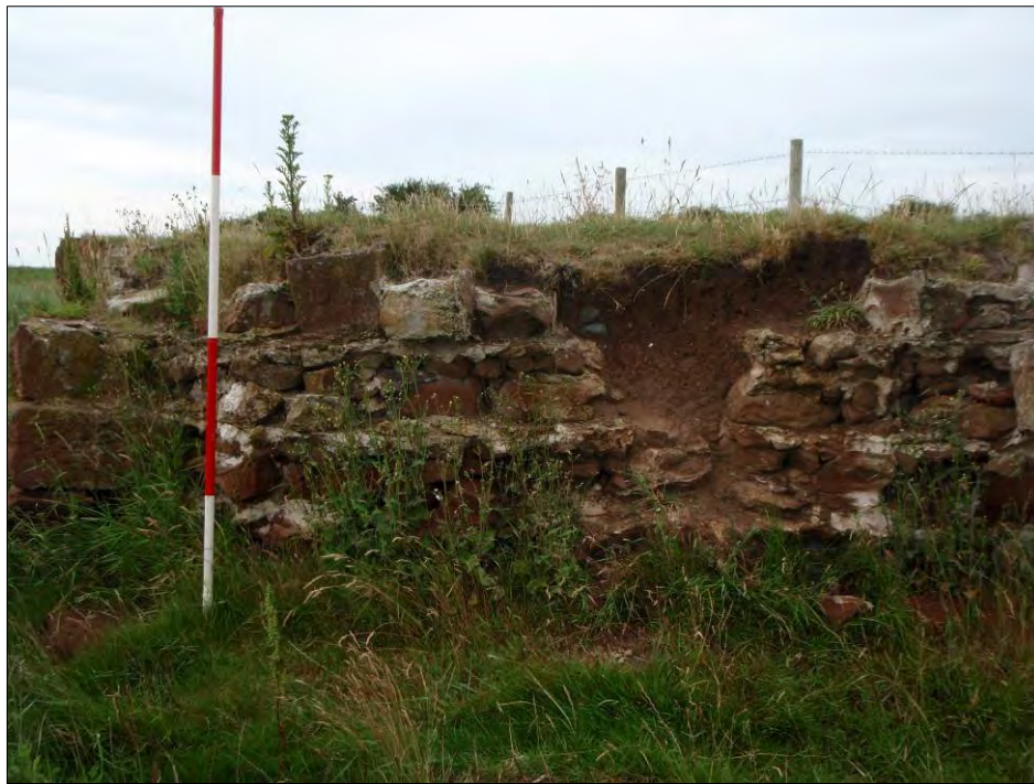
Figure 2.11 Erosion/stone robbing at Neston Old Quay (scale = 2m).
