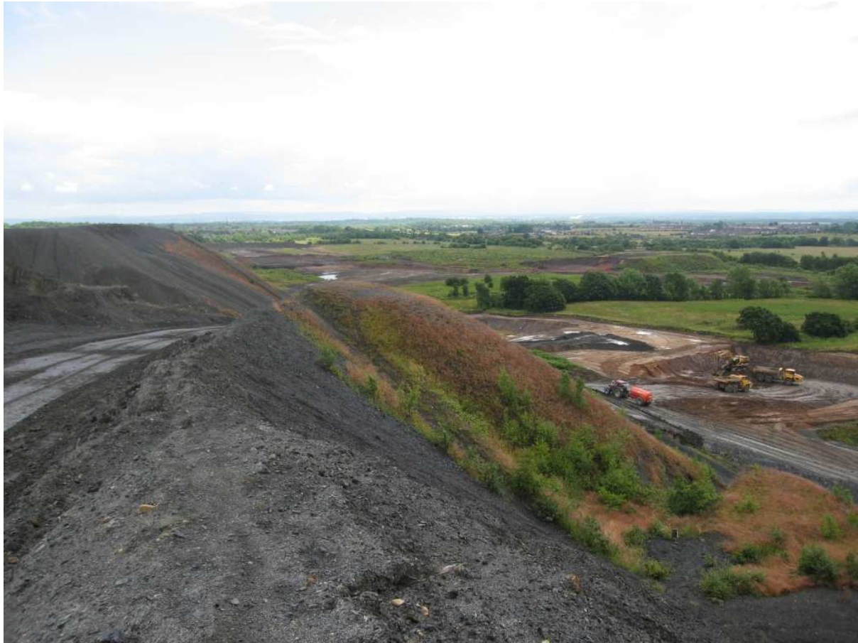
Figure 11e Cutacre opencast coal workings, straddling the border of Salford, Bolton and Wigan districts
