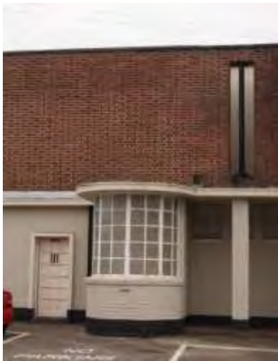
The remains of the 'Off Licence' at the Merchants Arms, Bell Hill, Stapleton. Architects: R. C. James and H. E. Meredith for The Bristol Brewery Georges and Company, Limited. Fiona Fisher and Rebecca Preston, 2014
