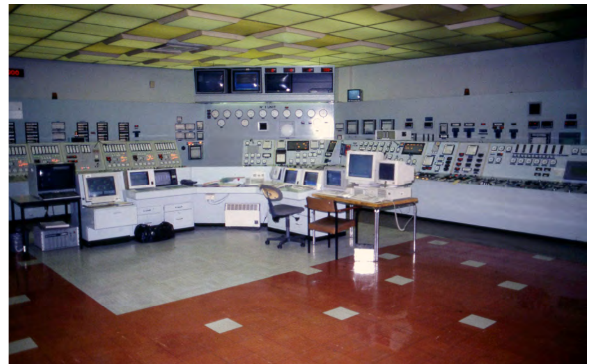
Below: The control room at Ironbridge in 1995 © Wayne Cocroft
