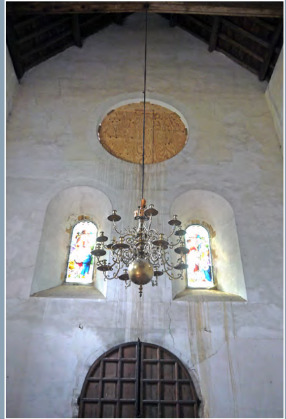
Water ingress and the damaged stained glass window
