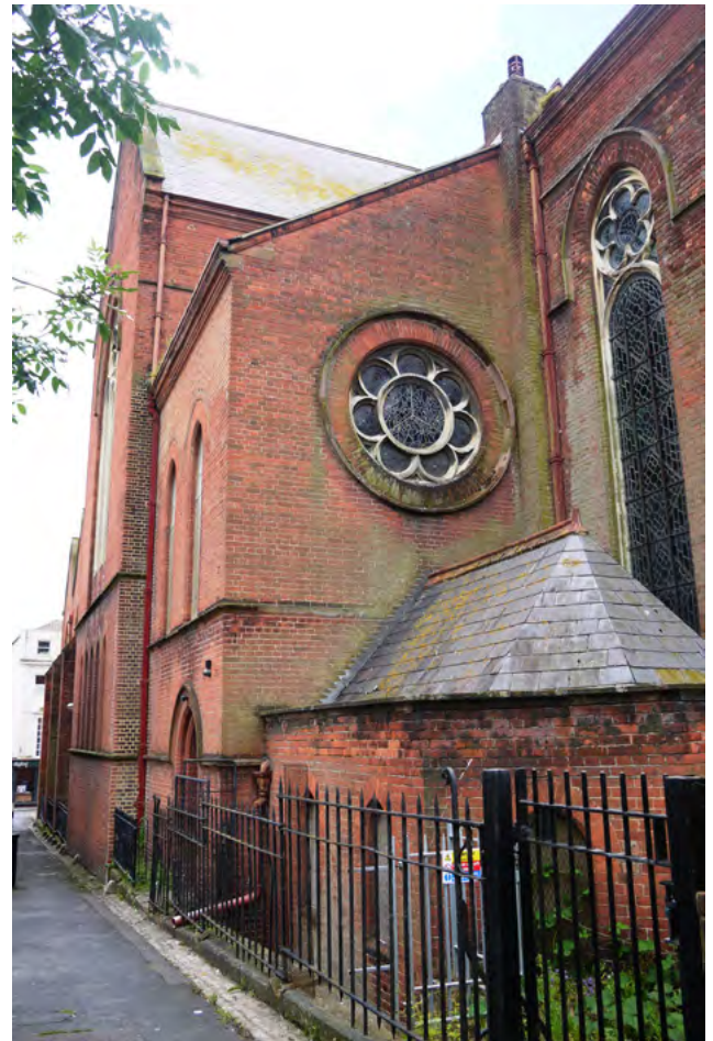
Poor condition of the external brickwork
