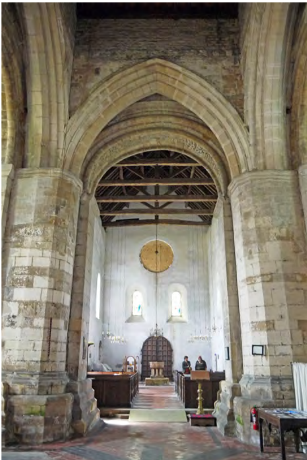
View west towards the nave (the west window blew out in a storm)
