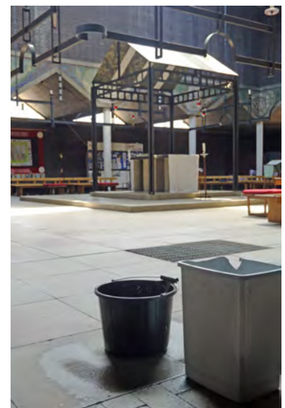
Minor leaks in the roof affecting the interior of the church
