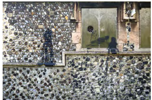
Vandalism to the rear of the Minster and intrusive anti-vandalism measures over windows at ground level
