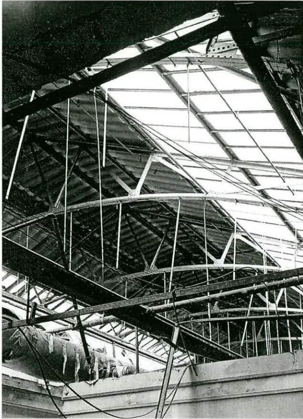
Fig 7 - Trussed roof principals of the former 'Liberal Arts Palace', glimpsed through suspended ceiling of the 1970s.
