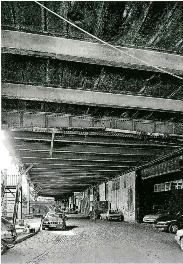
Fig 11 - Underneath the former 'Social Economy (Sports and Physical Culture) Hall', showing the cast- in-situ concrete floor.
