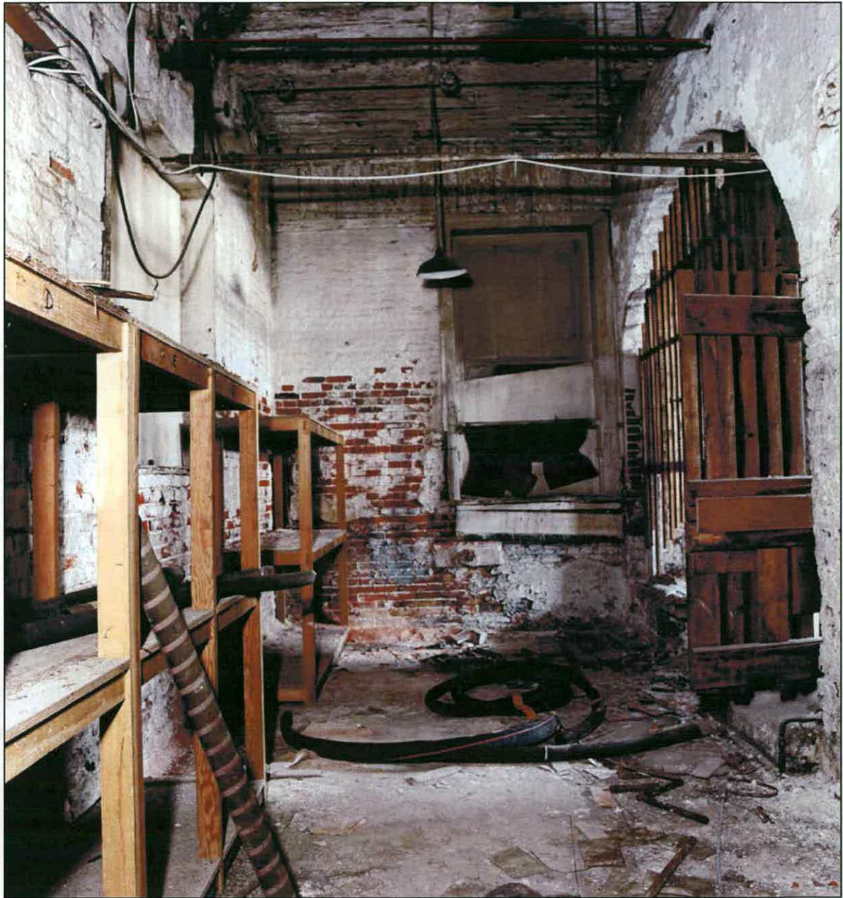
Figure 5. Inside the former engine house built for the Sadler engine in 1798 and subsequently modified. A photograph taken in 2003. [AA042399]
