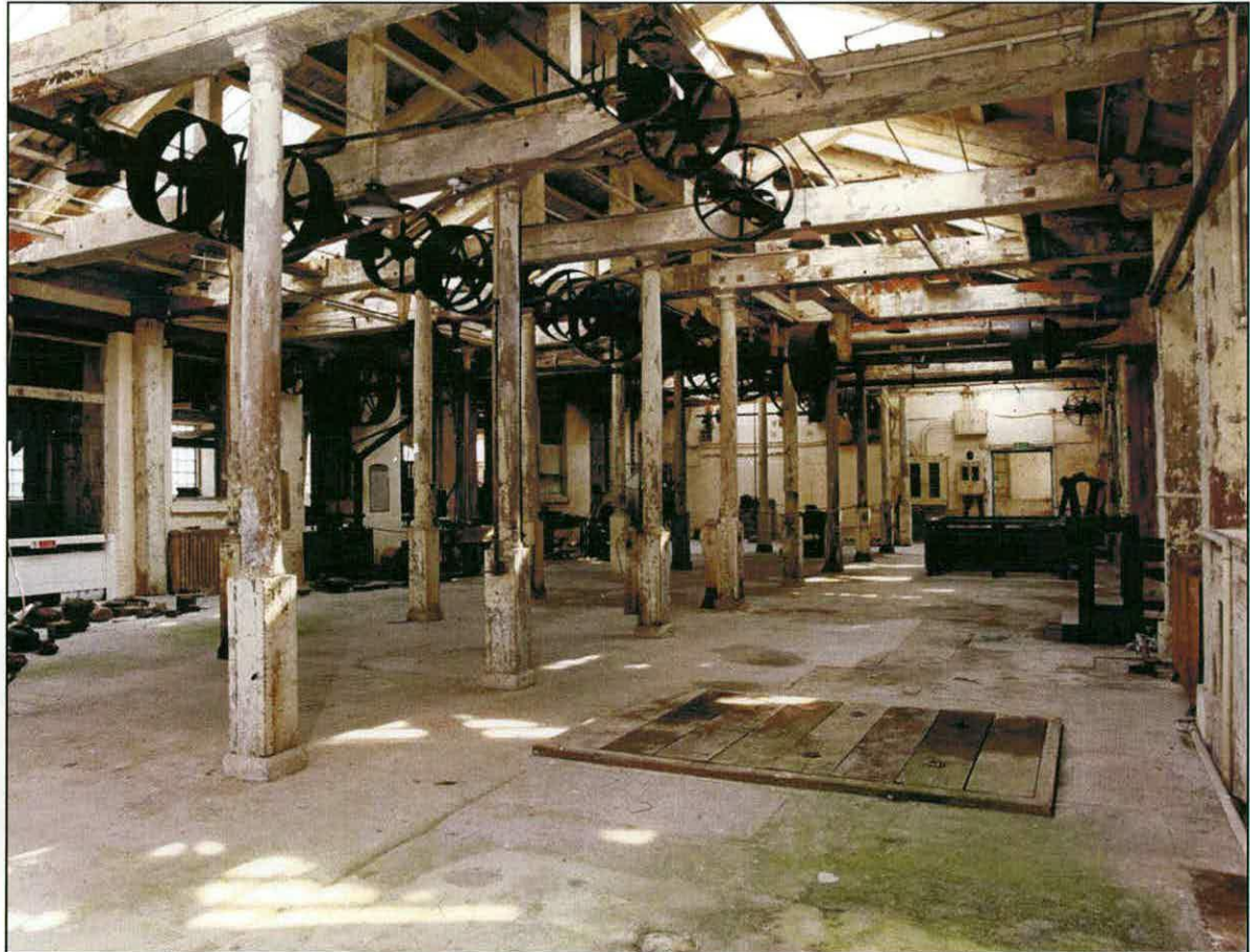
Figure 2. The interior of the Block Mills in 2003 showing the early overhead power transmission system and the turned wooden columns. [AA042405]
