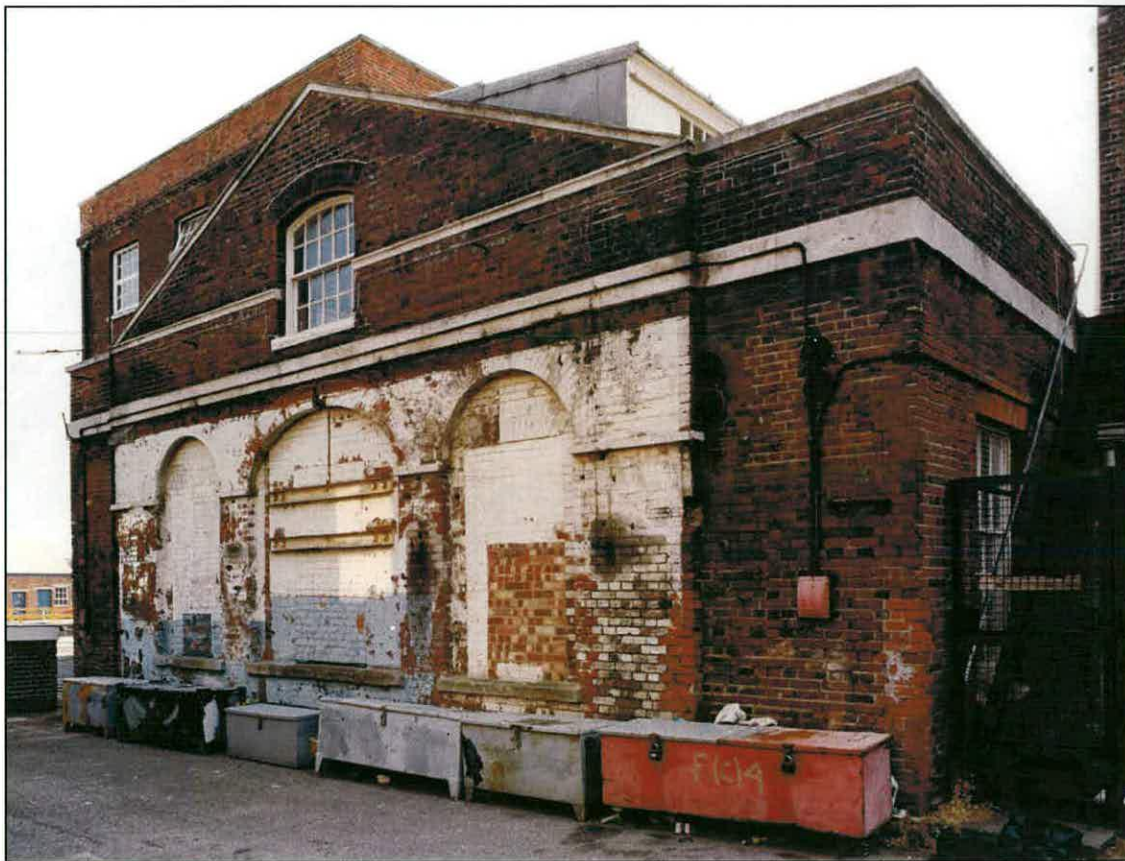
Figure 11. The workshop added to the eastern end of the Block Mills. Its original equipment was to include a small forge and bellows, an anvil, vice and a 'good foot lathe with drills and chucks and a variety of hand tools'. [AA042457]
