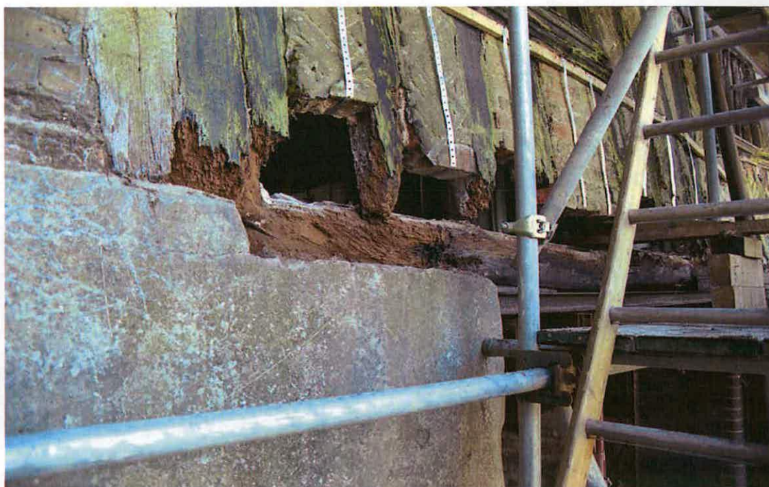
Figure 27 Detail of north wall of the Crossway, showing decayed feet of timbers at first floor level
