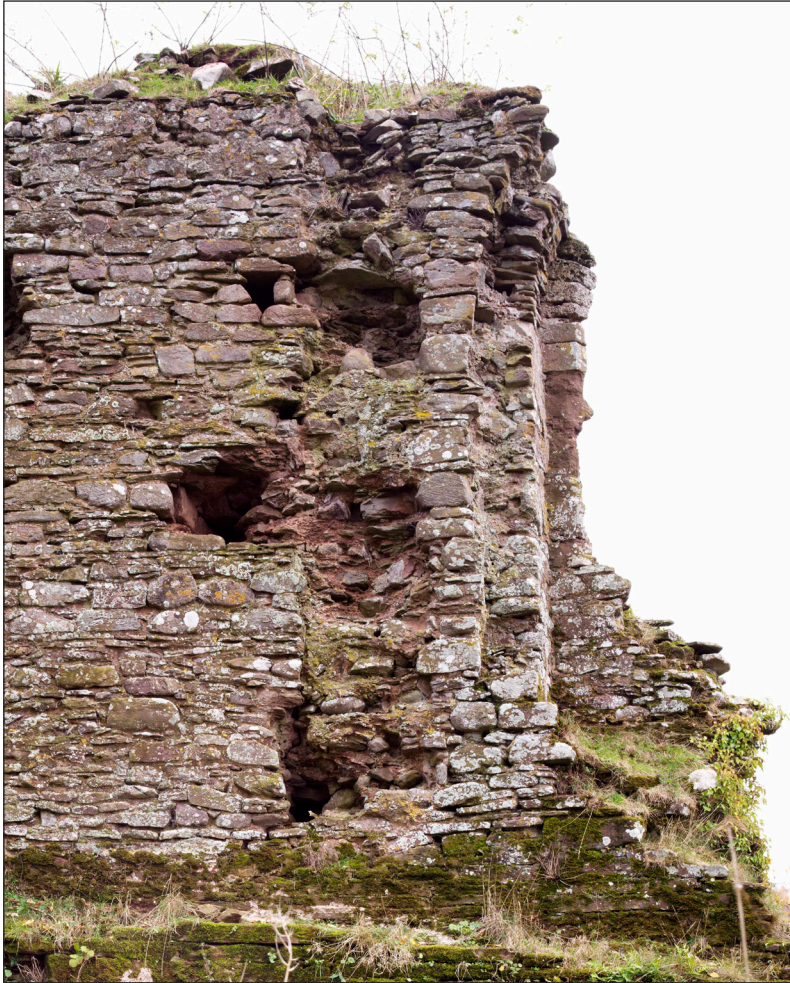
Figure 11 Exposed rubble core, possibly marking the position of a further subdivision in the building (DP195363 cropped).
