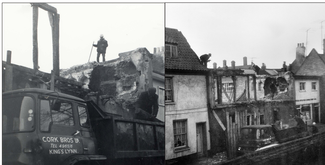
Figure 9: Two images of 47-49 Chapel Street under demolition in January 1967 showing the ogee-headed niches or windows in the north gable-end wall [Source: Norfolk Museums Service (Lynn Museum) KILLM 1992.217.19; Image: HEA DP219386]; [Source: Norfolk Museums Service (Lynn Museum), Image: HEA Red Boxes 4259/52 (4259/130) January 1967]
