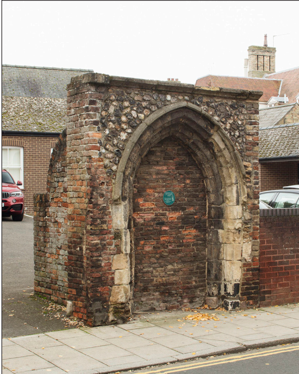
Figure 41: The Grade-II Listed probable 15th-century doorway, former entrance to Bennett's Yard, St Nicholas Street, standing isolated just beyond the north-western corner of the car park. [HEA DP217376 Patricia Payne 20-SEP-2017 ©Historic England]
