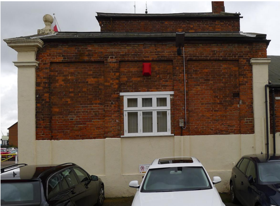
Fig. 81 The south elevation of the front part of the Baths, onto Ferry Street. Photograph: Jonathan Kewley 27-FEB-2017 ©Historic England
