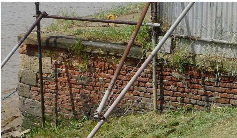
Fig. 21 The south-west corner of the old Common Staithe Quay, brick with stone dressings. Photograph: Jonathan Kewley 3-JUL-2017 ©Historic England
