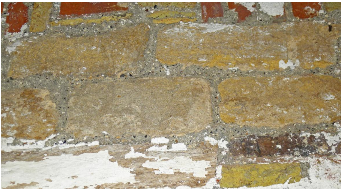
Fig. 76. Close-up of stone at high level on the south interior wall of the Buoy Store. Photograph: Jonathan Kewley 6-JUN-2017 ©Historic England
