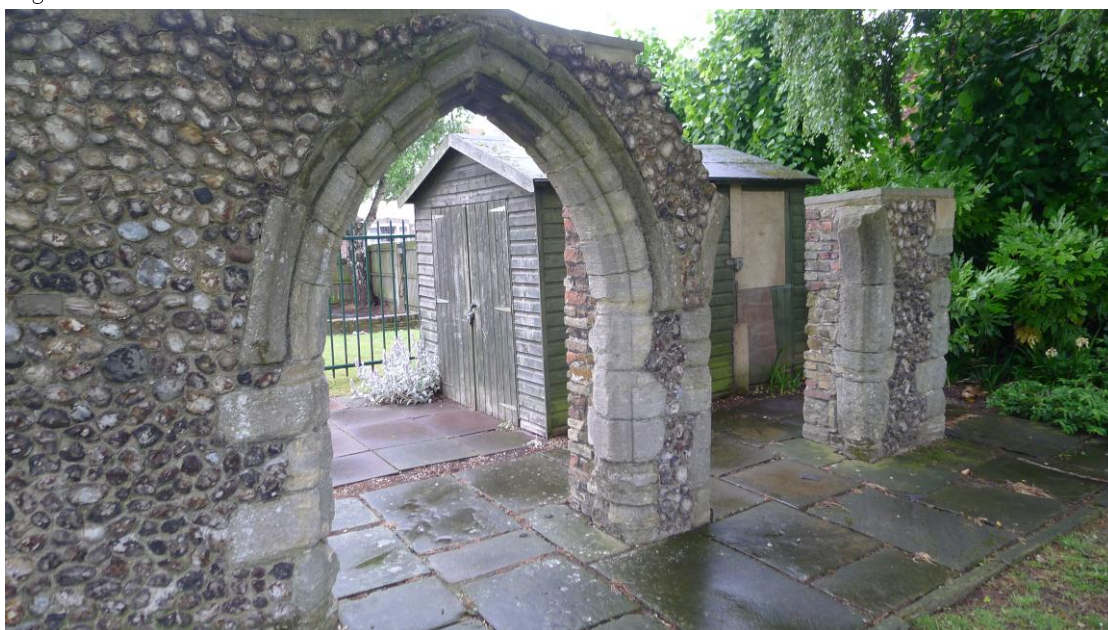
Fig. 111 The other part of the arcade now in Tower Gardens; a view from the north-east. Photograph: Jonathan Kewley 6-JUN-2017 ©Historic England
