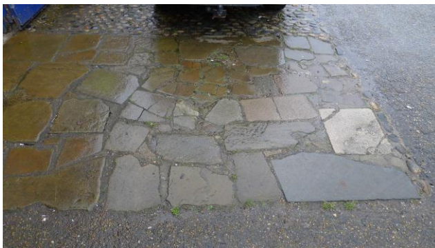
Fig. 72. Paving outside the door to the Engineers' Store. Photograph: Jonathan Kewley 6-JUN-2017 ©Historic England
