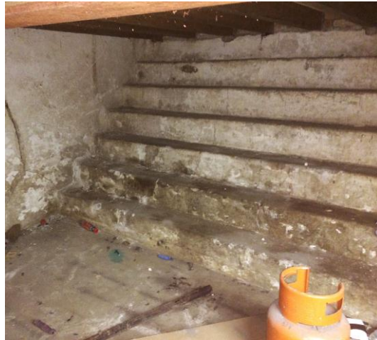
Fig. 94 The steps which run the full width of the west end of the swimming pool.
