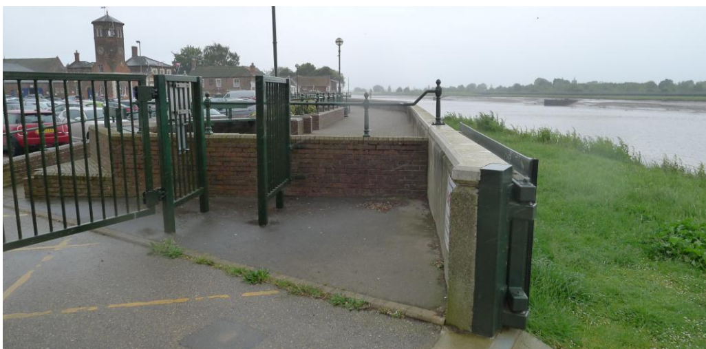
Fig. 123 The raised walkway along the river front of the Common Staithe; note the metal flood gate on the right. Photograph: Jonathan Kewley 6-JUN-2017 ©Historic England
