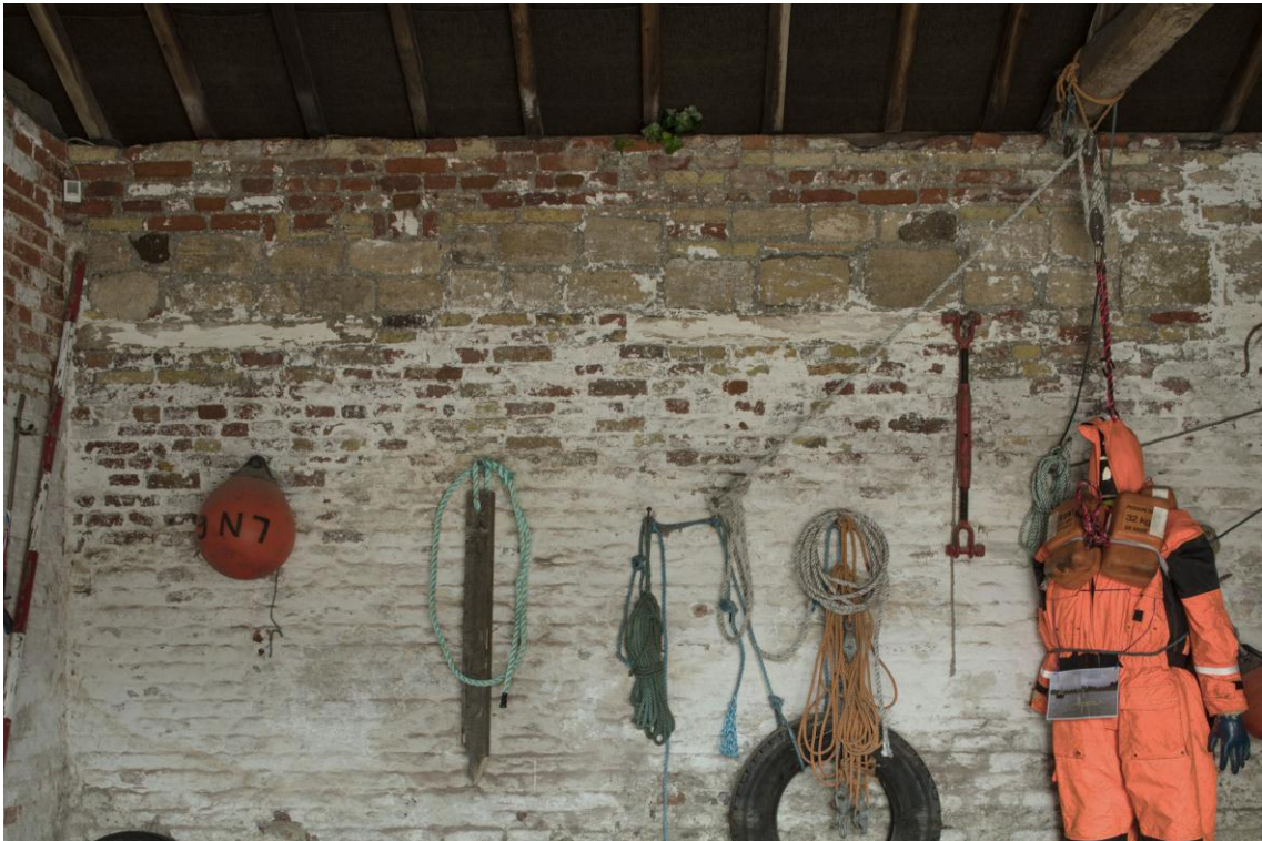
Fig. 75 The south wall of the Buoy Store from inside, showing re-used stone. Detail of HEA Patricia Payne 20-SEP-2017 ©Historic England
