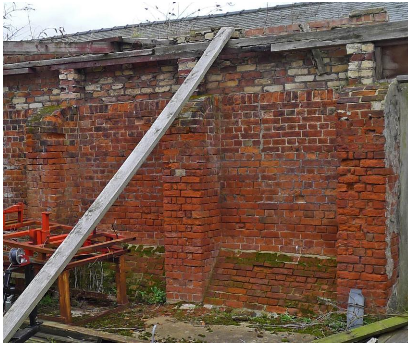
Fig. 100 Buttresses on the outer face of the south wall of the Settling Tank. Photograph: Jonathan Kewley 27-FEB-2017 ©Historic England
