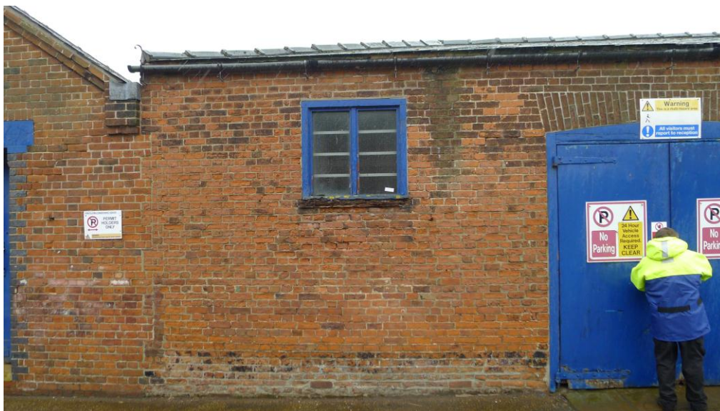
Fig. 70 The Engineers' Store from the north. Photograph: Jonathan Kewley 6-JUN-2017 ©Historic England
