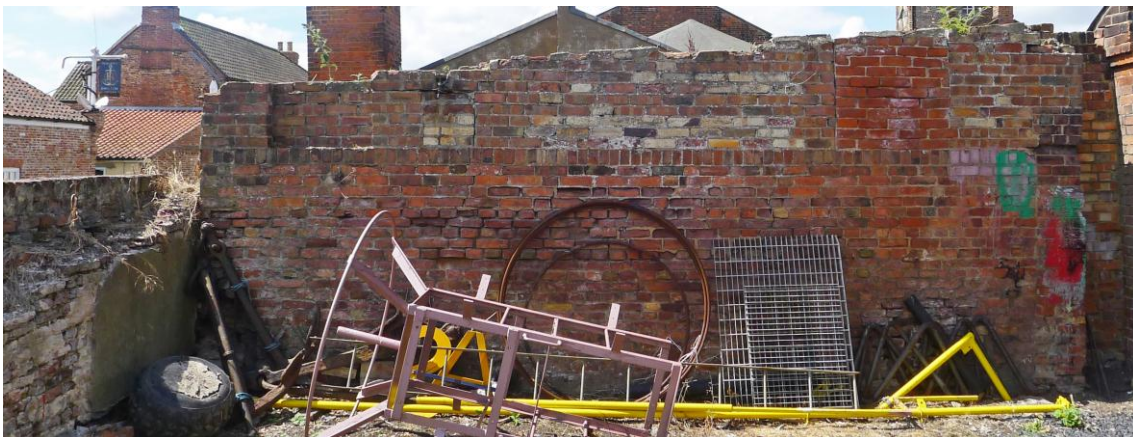
Fig. 117 Looking west from the yard south of the Carpenters' Shop, showing a wall which seems to be a dividing wall between units of the old south range on the Common Staithe, probably much rebuilt. Photograph: Jonathan Kewley 5-JUL-2017 ©Historic England
