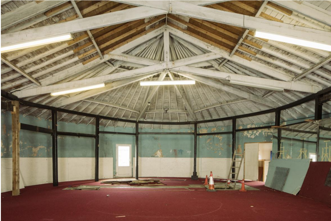
Fig. 91 The Swimming Pool hall looking east. Detail of DP217319 2-AUG-2017 Patricia Payne ©Historic England
