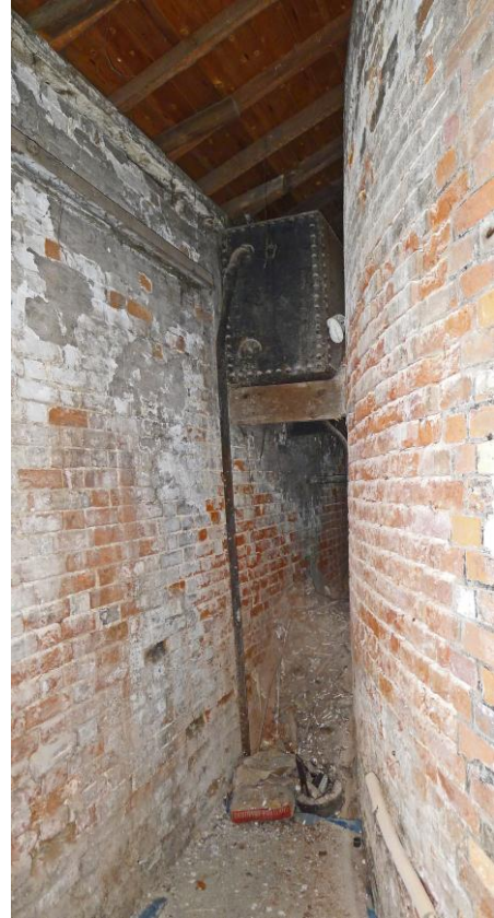
Fig. 90. The space between the south wall of the Baths (on the left) and the cirving south wall of the Swimming Pool Hall (on the right), looking west. Photograph: Jonathan Kewley 6-JUN-2017 ©Historic England
