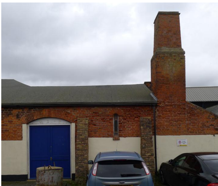
Fig. 89 Buttresses supporting the south wall of the Baths. Photograph: Jonathan Kewley 27-FEB-2017 ©Historic England
