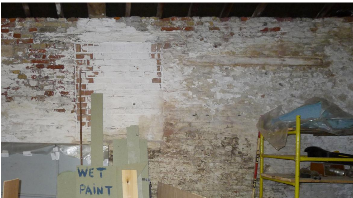
Fig. 65 A blocked-up window in the south wall of the Buoy Store. Photograph: Jonathan Kewley 6-JUN-2017 ©Historic England
