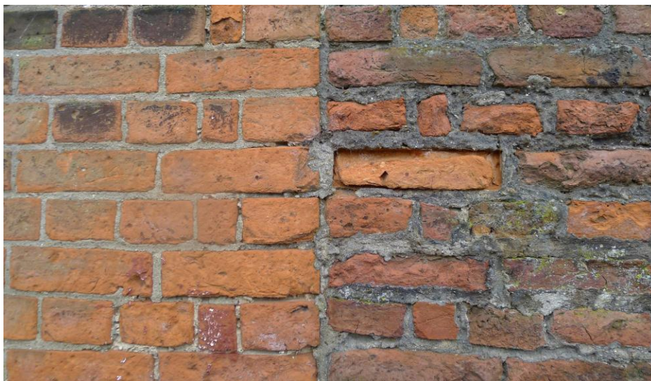
Fig. 36 The break in the brickwork between the 1829 (right) and 1834 (left) warehouses. Photograph: Jonathan Kewley 6-JUN-2017 ©Historic England
