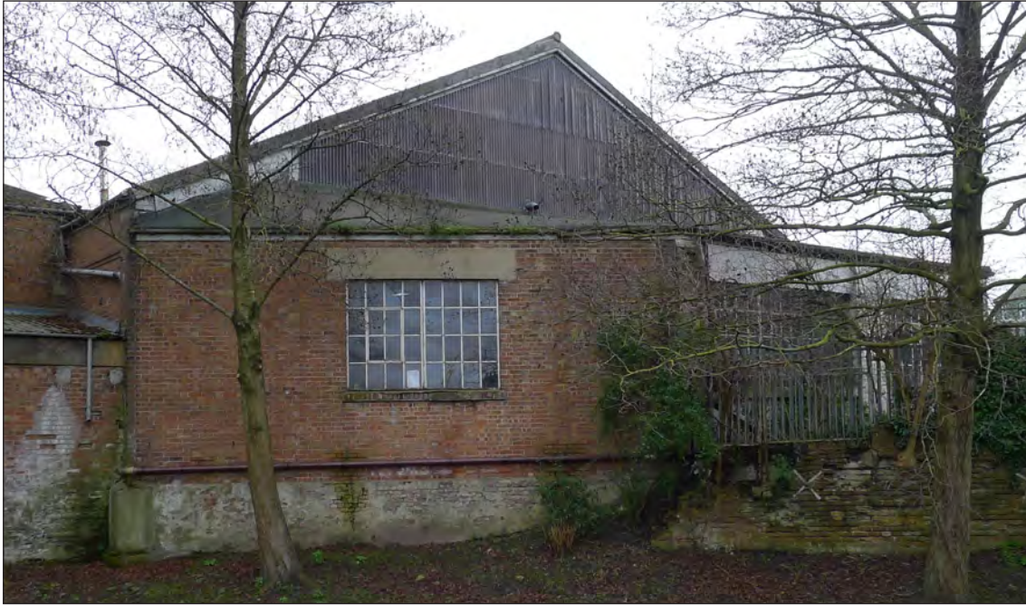
Fig 227 The rear (north) elevation of the earlier part of the Bus Garage, taken from Southgate Park. Photograph Jonathan Kewley 16-JAN-2018 © Historic England
