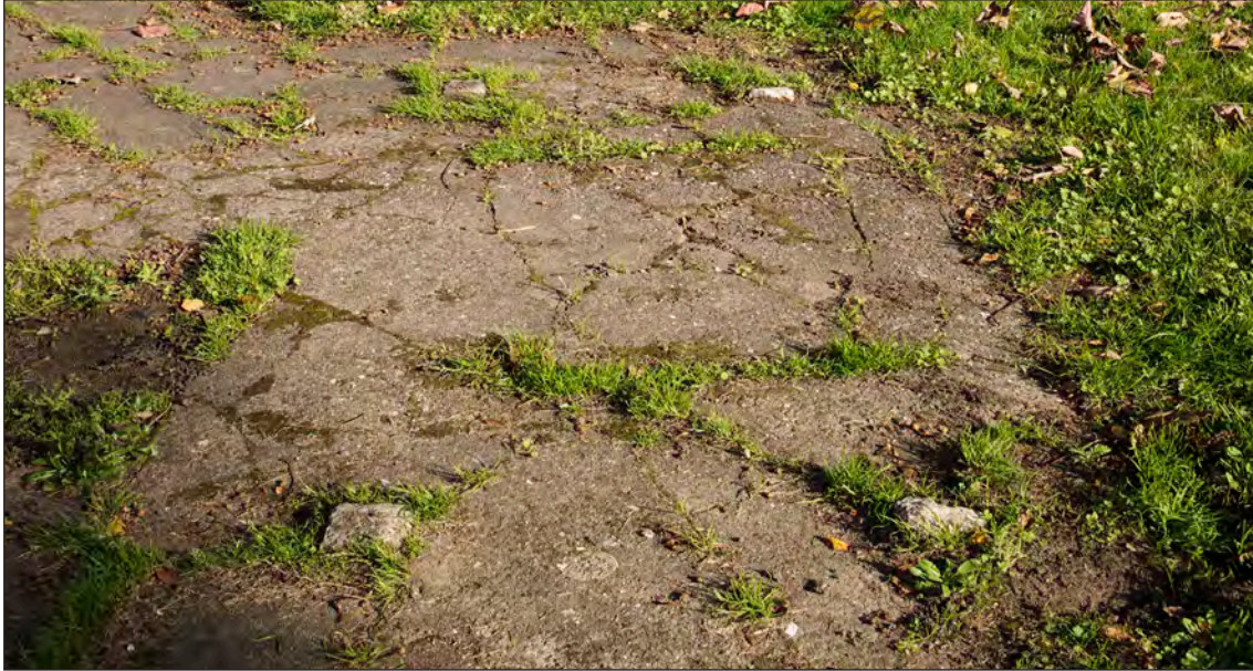
Fig 95: An example of the truncated concrete legs which mark the former locations of concrete benches (HEA DP219112 Patricia Payne 17-OCT-2017 © Historic England)
