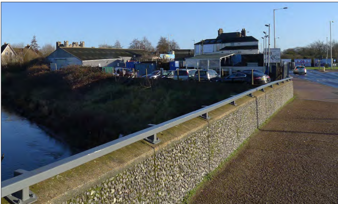
Fig 12. The present Long Bridge over the River Nar, looking east. Note the concrete inlaid with flint. Photograph: Jonathan Kewley 19-FEB-2018, © Historic England
