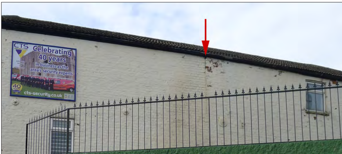
Fig 162 The east wall of the Highland Laddie, showing the break in the brickwork. Photograph Jonathan Kewley 27-FEB-2017 © Historic England
