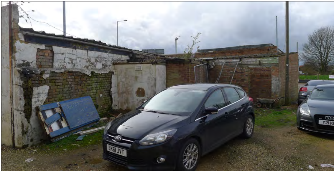
Fig 169 The parade of shops from the rear. Photograph Jonathan Kewley 27-FEB-2017 © Historic England
