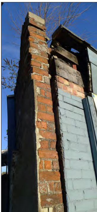
Fig 170 (left) The east (and only surviving) wall of the building west of the shops on the Wisbech Road which was used at one time by the fitters from the Gas Works. Photograph; Jonathan Kewley 16-Jan-2018 © Historic England
