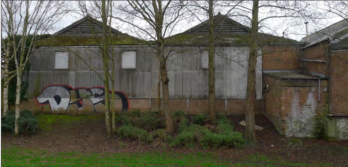
Fig 229 The rear (north) elevation of the 1933 extension to the Bus Garage, from Southgate Park; in the foreground is the now-dry course of the Middleton Stop Drain. Photograph Jonathan Kewley 27-FEB-2017 © Historic England
