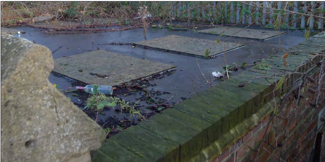
Fig 238 The underground former public lavatories on the east side of Out South Gates. Photograph Jonathan Kewley 16-JAN-2018 © Historic England
