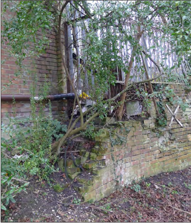
Fig 231 The north-west corner of the Bus Garage, showing its relationship to the older retaining wall on the right. Photograph Jonathan Kewley 27-FEB-2017 © Historic England
