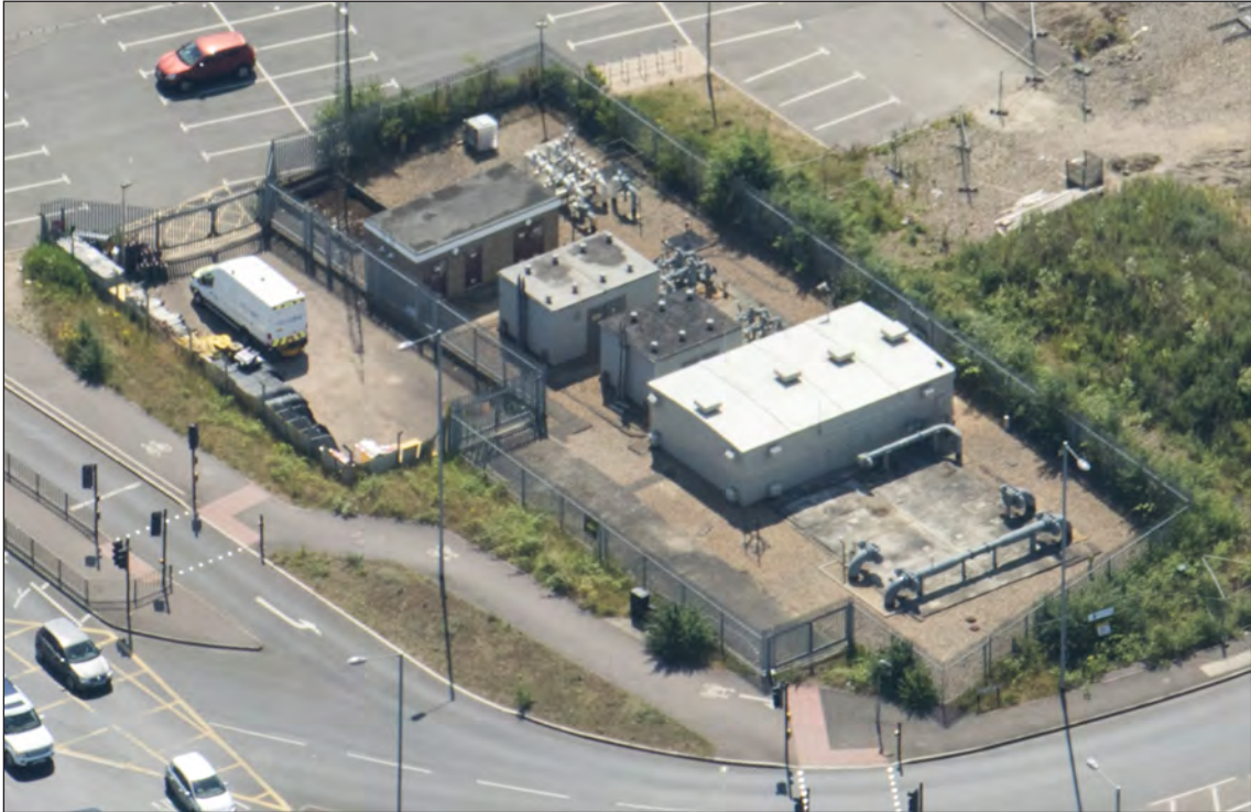
Fig 208 The National Grid Gas Pressure Reduction Station and Depot from the air. Detail of HEA 33197/025 Damian Grady 19-JUN-2017 © Historic England
