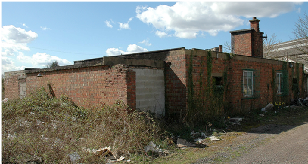
Figure 17: Cleansing (decontamination) and first-aid post (Bldg.48) – a view looking NW, now demolished. [Richard Flagg 07-08-2009]
