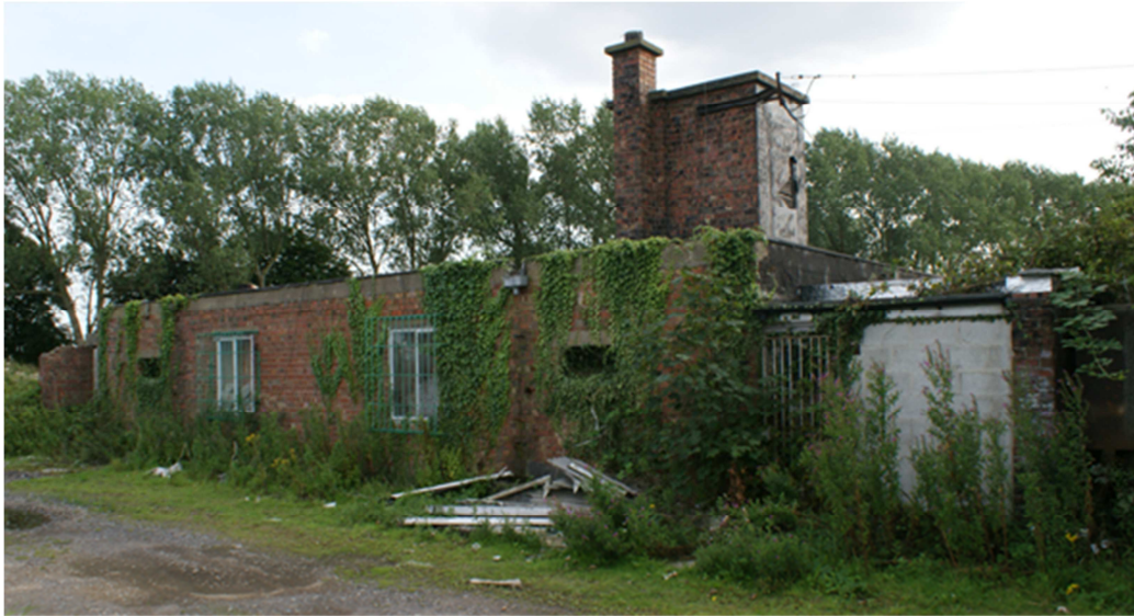
Figure 16: Cleansing (decontamination) and first-aid post (Bldg.48), view looking SE, now demolished. [Paul Francis 07-08-2009]
