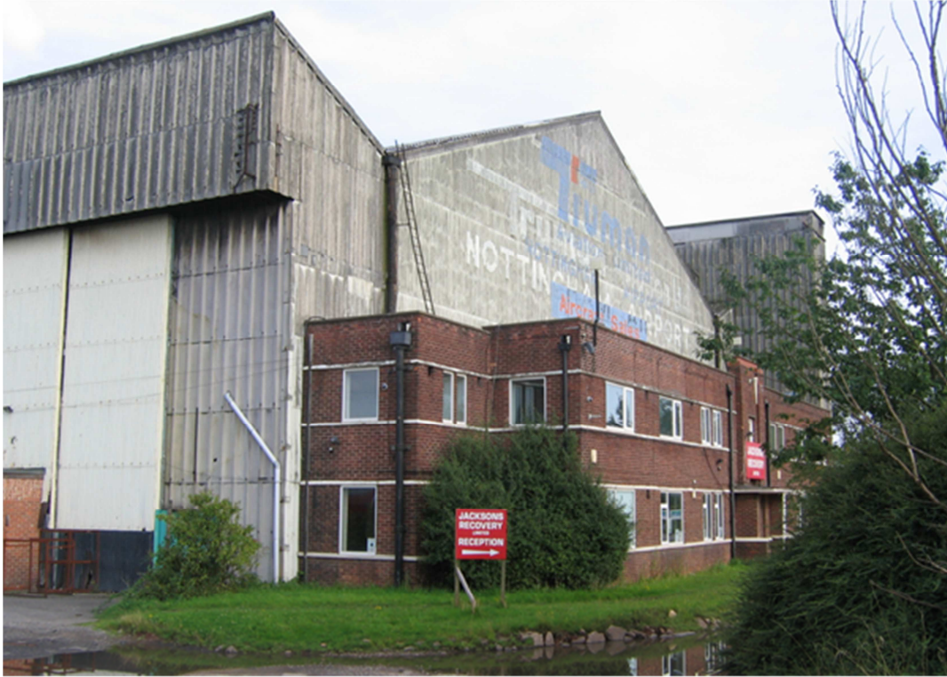
Figure 5: To the left of the rainwater pipe a slightly raised portion of cladding indicates the position of the door that was used by the fire watchers to gain access to the roof. [Milan Petrovic 07-08-2009]
