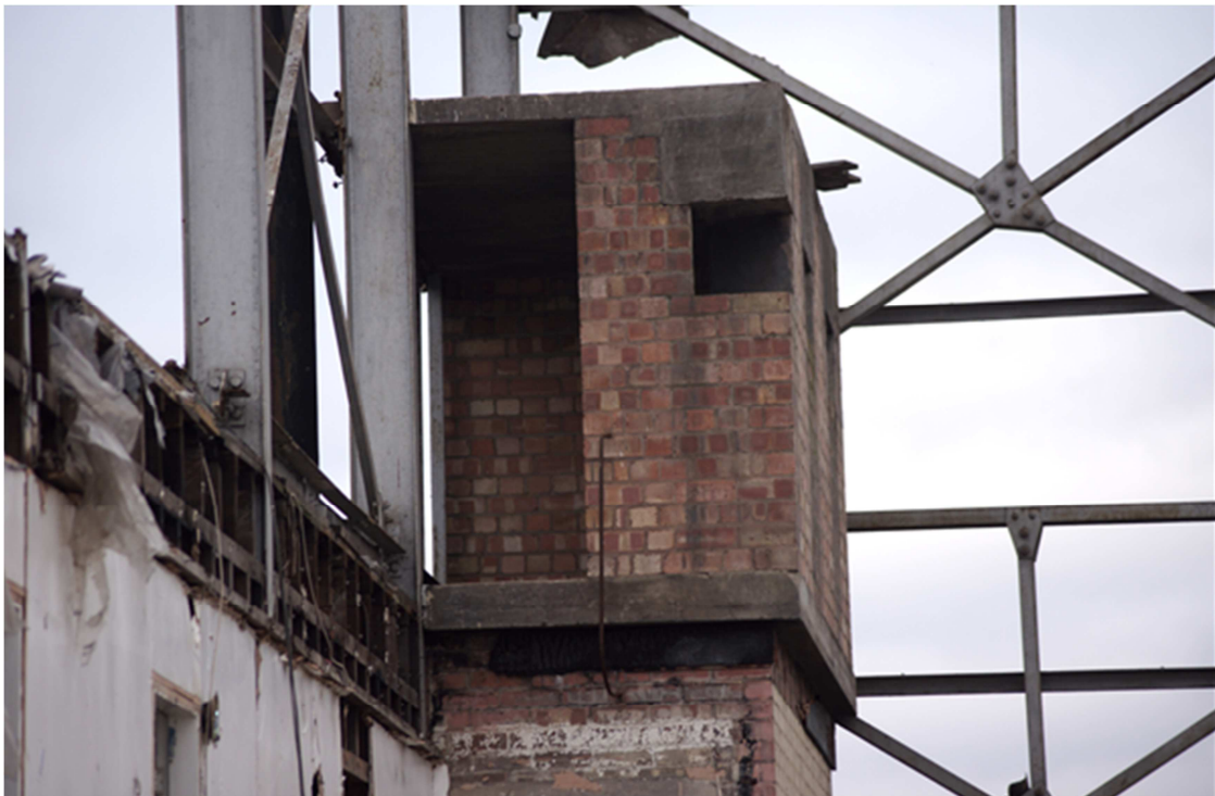
Figure 11: View from the hangar's interior showing entrance side (south) elevation. [Paul Francis 05-12-2017]
