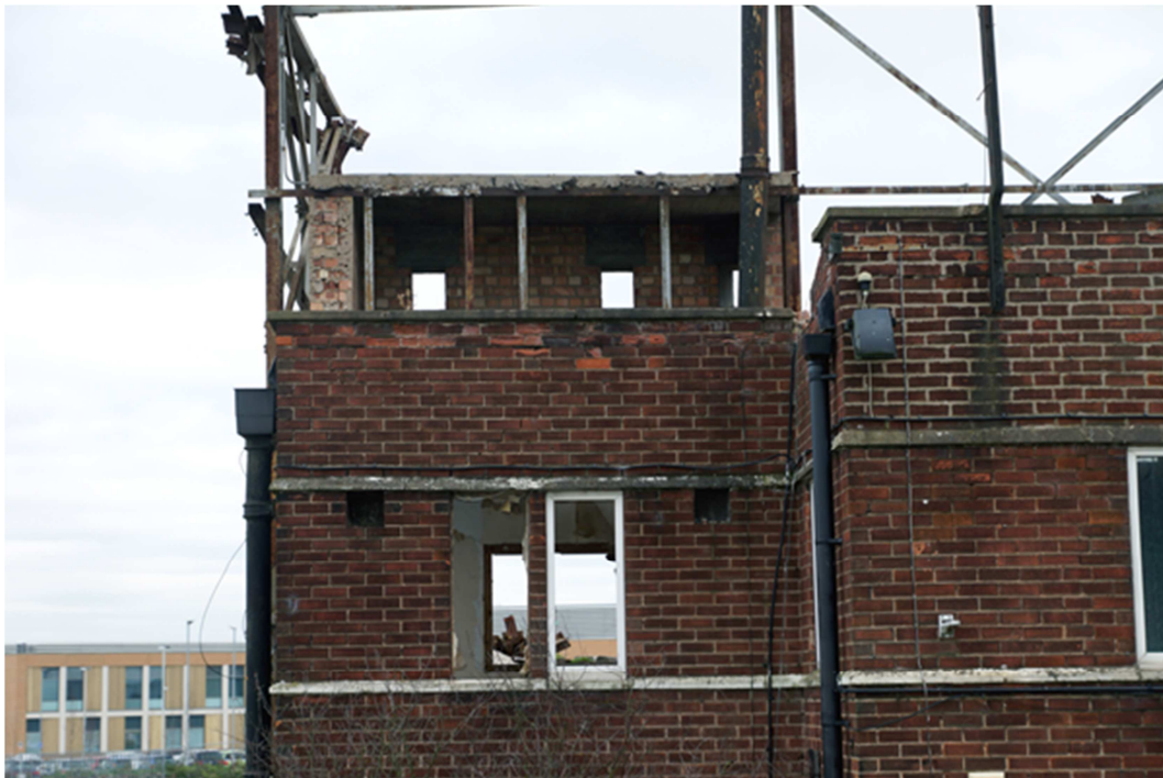
Figure 9: Exterior view looking east, it is partially hidden by the parapet wall of the flat roof. [Paul Francis 05-12-2017]
