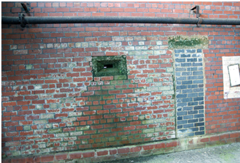
Figure 25: Brick fire watcher's post Royal Ordnance Factory Bishopston – NGR: unknown. [Paul Francis October 2009]
