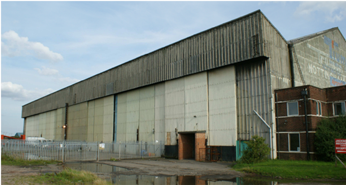
Figure 26: Main hangar, airfield elevation (Bldg.43). Note the roof access ladder positioned close to the fire watcher's shelter (which is hidden behind the wall cladding). [Paul Francis 07-08- 2009]
