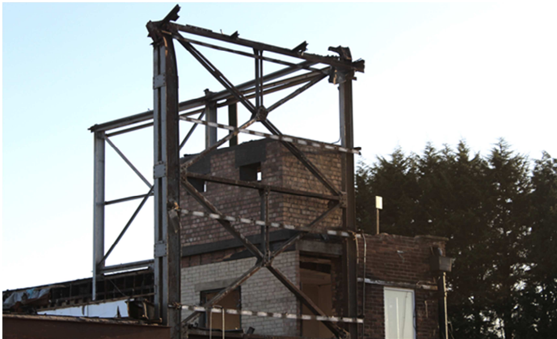
Figure 15: Views showing the metal brackets from the hangar wind girder framework preventing movement of the brick work and roof slab. [Milan Petrovic 15-03-2017]
