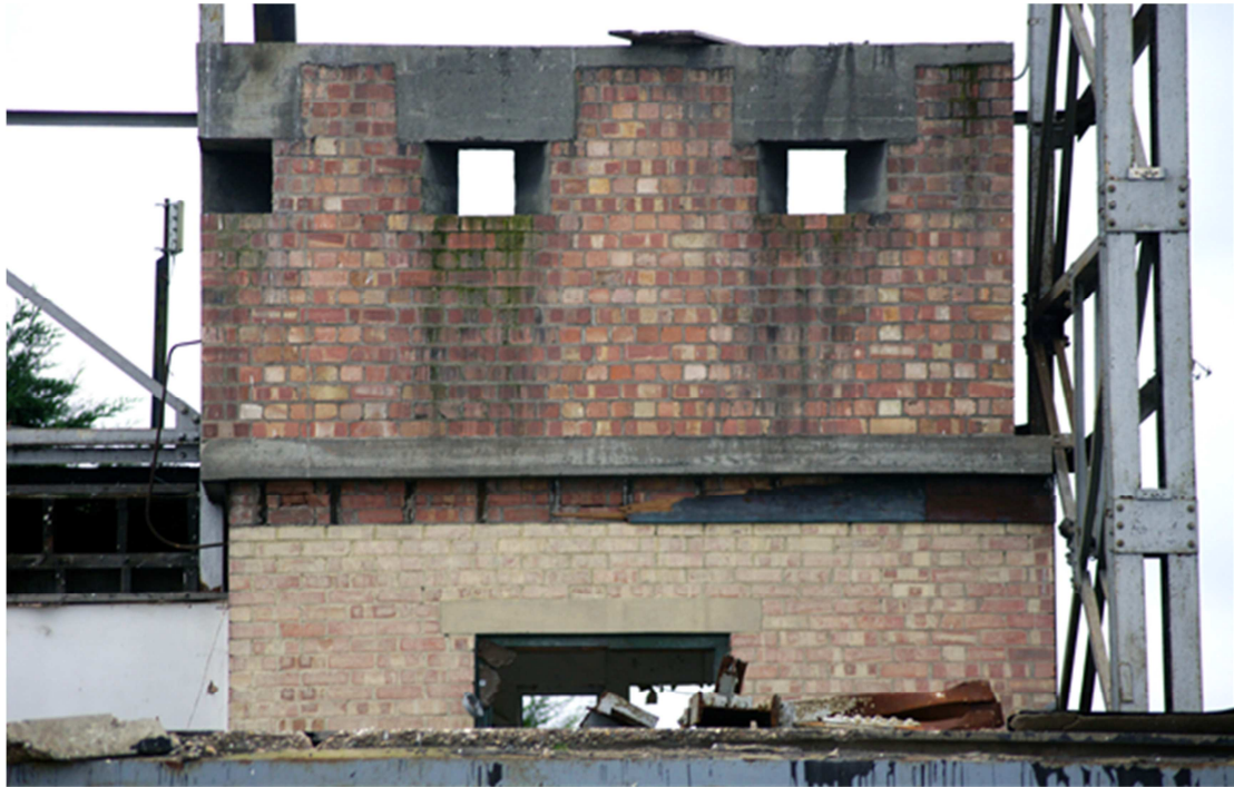
Figure 10: View from the hangar's interior showing the front (east) elevation. Note the row of joists below the floor slab. [Paul Francis 05-12-2017]
