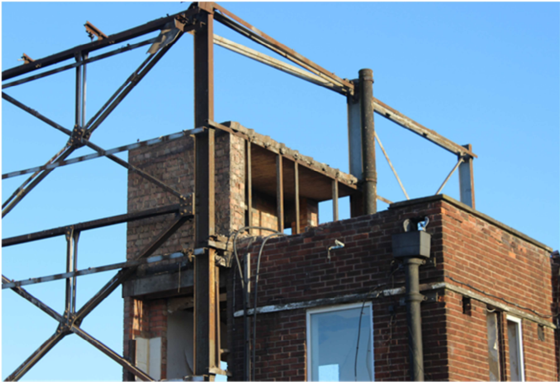
Figure 14: Views showing the metal brackets from the hangar wind girder framework preventing movement of the brick work and roof slab. [Milan Petrovic 15-03-2017]
