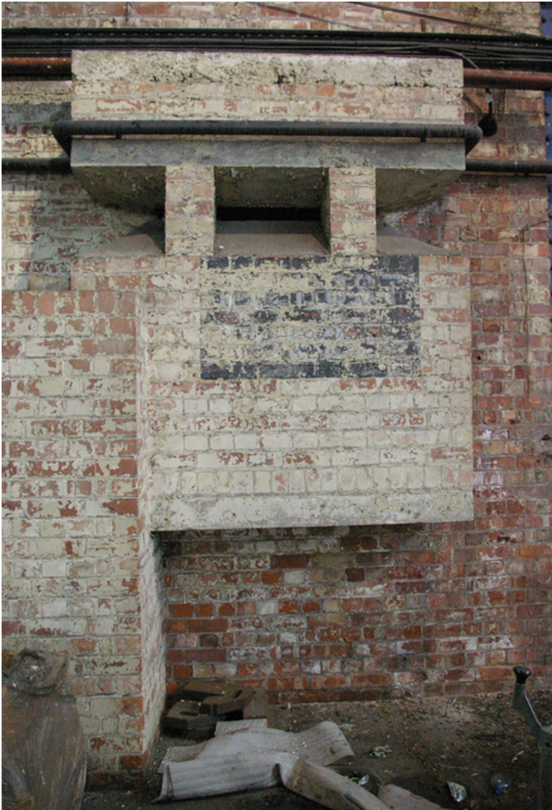
Figure 21: Fire watcher's shelter inside a north-light hangar – NGR: SJ 81013 84727 (hangar) at Ringway (Manchester Airport). [Ian Anderson]
