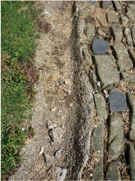
Fig.77. Several of the Tiverton gutters formed in the ground surface adjacent to the path were once lined with asphalt. It is not known whether this lining was primary or an amendment.
