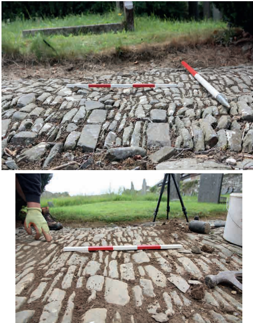
Fig.160, Slumps repaired by relaying (including relaying lost and overturned kerbs) during the trial at Merton, work by Williams and Burrows, supervised John Alexander, funded by the SPAB, associated with discussions with Francis Kelly of Historic England, Simon Cartlidge of the DAC, Jo Cox and John Thorp of Keystone and Ray Harrison.
