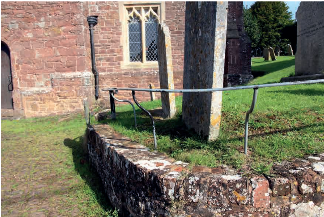
Fig.151. A welcome and serviceable handrail at Sandford on a path that avoids some, but not all, of the steps up to the church. It is need of re-decoration to make it more appealing to use, or abandoning the painted surface altogether.
