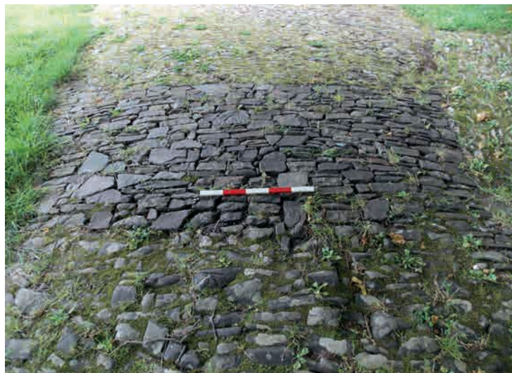
Fig.157. Top. Small repairs to the Exbourne cobbles are visible adjacent to a drain along the front of the porch. Below. A large section of repair to the path at Buckland Brewer. Repairs to this path include replacing tarmac with cobbles. The church has the advantage of a skilled cobblestone-layer living just outside the lychgate who has also repaired a long cobbled footway in the village.
