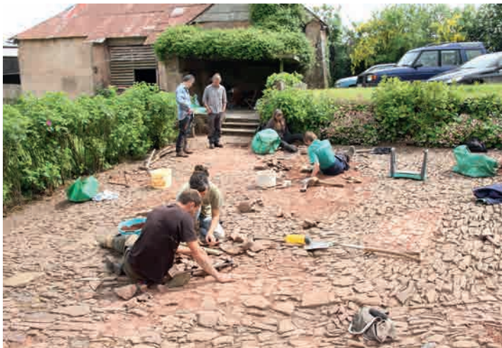
Fig.39. Above and left. Repairing farmyard cobbles in Mid Devon on a one-day cobblestone-laying course tutored by Jennie Goodwin for the Devon Rural Skills Trust. The cobbles were larger than most used for church paths and expectations were for a rougher surface than churchyard cobbles.
