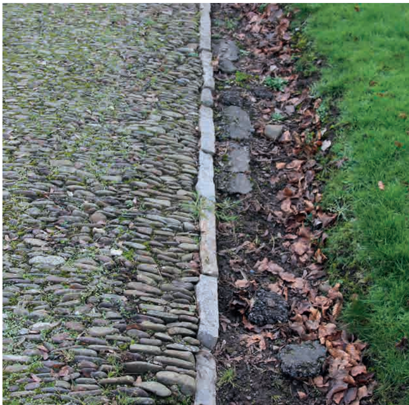
Fig.68. Open gutters either side of one of the paths at Tiverton, St Peter with evidence of disintegrating asphalt lining. The edge restraint of dressed stone kerbs looks substantial but these are overturning into the gutter, probably for a second time as the cobbles adjacent to the kerbs appear to have relaid after an earlier failure.
