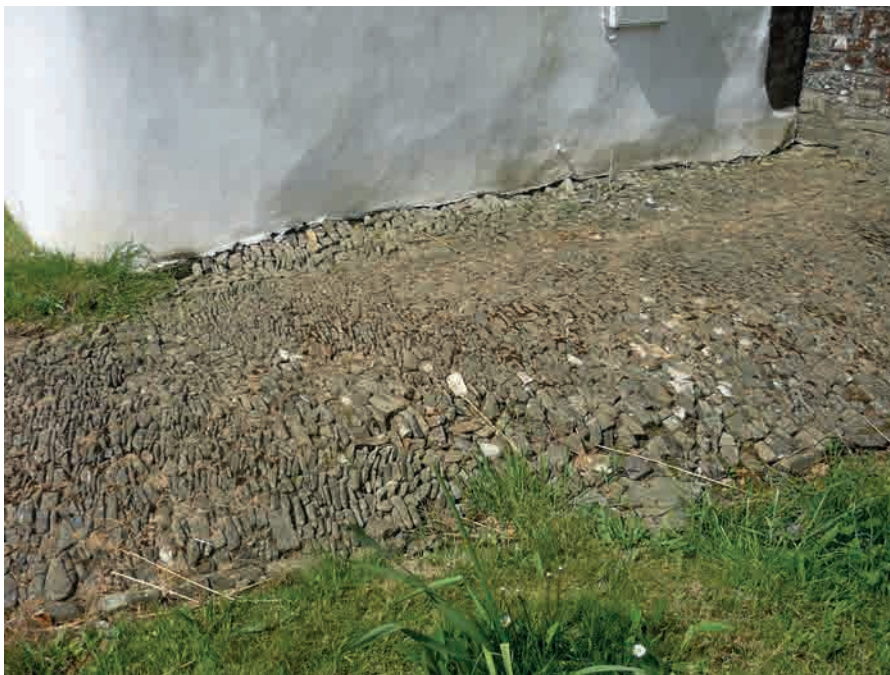
Fig.61. Examples of jointing scour out. This may be localised, e.g. (top) the sloping cobbled apron to the Victorian churchyard wall at Merton has retained most of its earthen jointing except (top right) where water from the lychgate roof has washed it out, some of the cobblestones eventually falling out of the matrix. (Below) a more general washout of jointing with a deposition of silt and clay which has collected in a shallow gutter between two sections of path.
