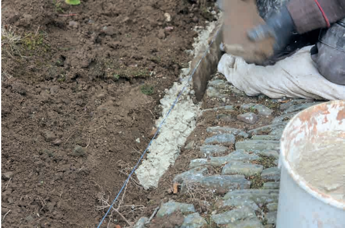
Fig.79. Trial re-laying of kerbs at Merton by Williams and Burrows, trials funded by the SPAB and undertaken under the supervision of John Alexander. On the S side of the path the kerbs were reinstated with haunching using lime. The N side kerbs were relaid using subsoil and some buttressing with small stones.
