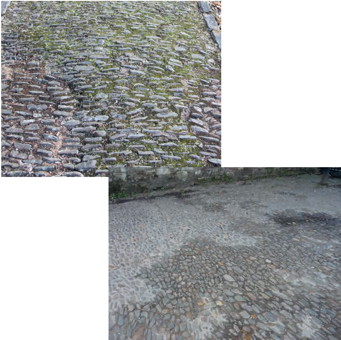
Fig.64. Well-meaning repairs in cement create rigid patches in a flexible pavement, speeding up jointing scour at the junction with the earthen jointing. This is illustrated at Tiverton St Peter (top) and more comprehensively in a semi-secular context at Cathedral Close, Exeter where the extent of cementitious jointing may eventually damage the path down to and beyond the formation level: note the top right slump.
