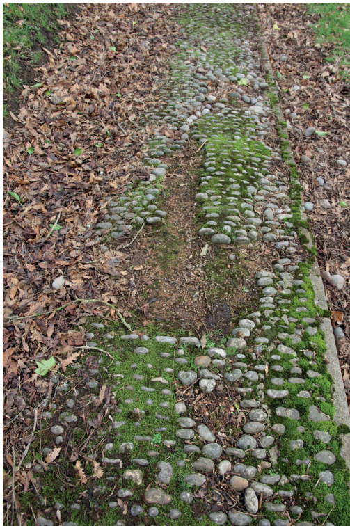
Fig.158. Top, a tiny patch in cement to a patterned section of a path at Alphington is typical of well-meaning work but eventually ineffective work to reinstate dislodged cobbles and keep a path even. Middle, a much larger cement patch to a sub-path at Tiverton St Peter is causing damage to the adjacent earth-jointed cobbles. Bottom, a sub-path at Tiverton, relaid in the 20th century using pebbles laid horizontally, bedded in cement with concrete kerbs has failed. In the opinion of the authors of this report this little-used and, in terms of construction, untraditional path is a lost cause and would be better removed than retained.
