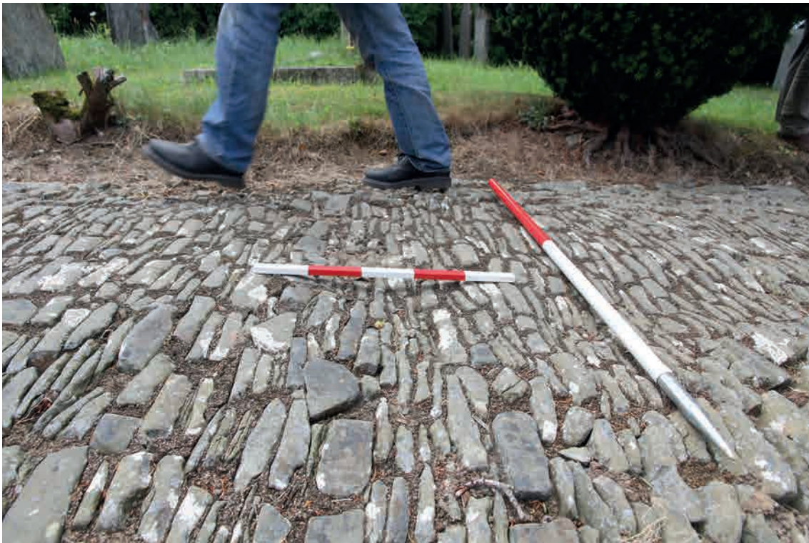
Fig.56. Slumps in the path at Merton have occurred without fracturing the pavement.
