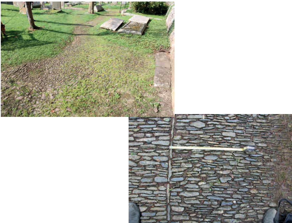
Fig.155. Weed/grass growth. Top, Sandford St Swithun. Below, Exbourne, one of the best-maintained paths seen. Weeds here are killed with a chemical weedkiller whenever they are noticed by a parishioner who regularly walks through the churchyard (pers.comm.) Revetment walls to the path keep it isolated from the churchyard turf: this avoids weedkiller spread.
