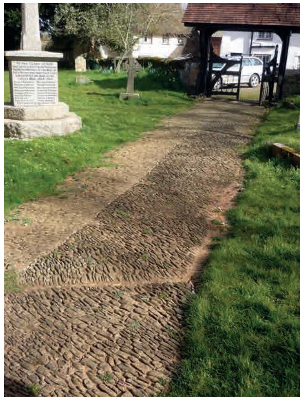
Fig.67. This path (Upton Pyne) has crossfalls from the centre line to each side. Water falling on it is channelled to a diagonal junction in the paving in the foreground. Here and at the junction with the grass, jointing material scoured out from between the cobbles is deposited. We did not investigate the path edge detail, if any.
