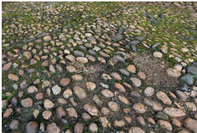
Fig.146. Variations in cobbled surfaces: this page and opposite. Above, lost and loose pebble cobbles at Poltimore. Opposite, clockwise from top right. A relatively level, even and flat path at Exbourne; a water-filled sinking at Petrockstow after rain; a well-preserved path at Hatherleigh between revetment walls. The overshadowed path at Petrockstow illustrates the impact of environmental factors. It does not allow sun to shine on the path or air movement to keep it dry. The narrowing of the width by the foliage is also a barrier to access for people with visual impairment or two people walking side by side (such as a disabled person holding on to a companion or a bride to her husband) or those carrying a coffin.
