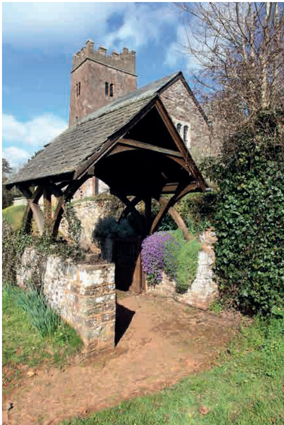
Fig.51. Changing direction. At Newton St Cyres, St Cyriac and St Julitta (top left), the cobbled apron round a vestry of c.1920s date turns a corner of 90 degrees in the form of a fan. At Upton Pyne, Our Lady (right), internal cobblestone kerbs create a junction where a path turns a corner and the cobbles on either side are laid in different directions. At Upton Hellions, St Mary (bottom left), a path turns one right angle before arriving at the lychgate and another as it turns to the church porch. The cobblestones are laid the same way along the whole length of the path, so they lie at right angles across the main section of the path, but on the long axis on the short sections of path before the lychgate and the porch.
