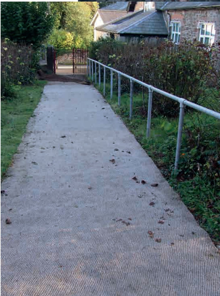
Fig.167. Coir matting (since replaced) used to cover cobbles on a steep path to a busy church at Black Torrington. Photographs supplied by the DAC.
