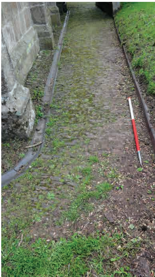
Fig.69. Examples of open gutters which also function as edge restraint. Clockwise from top left: a cobbled gutter at Petrockstow; a stone gutter at Hatherleigh and a ceramic gutter at North Molton.
