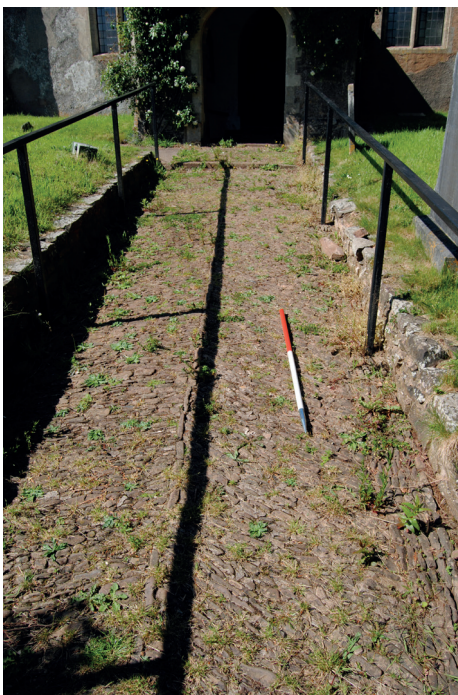
Fig.171. Handrails installed at Coldridge following a 2011 faculty. These are accompanied by a sensible notice on the churchyard entrance. The uprights of the Cadeleigh handrails are fixed into the cobbles. There may have been reasons why a cantilevered arrangement off the churchyard turf was not possible.
