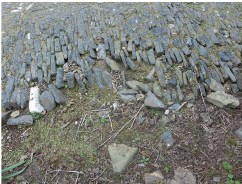
Fig.76. Path kerbs to the churchyard path at Merton have overturned, a common failure and, in this case, dispersed, along with part of the cobbled path surface.
