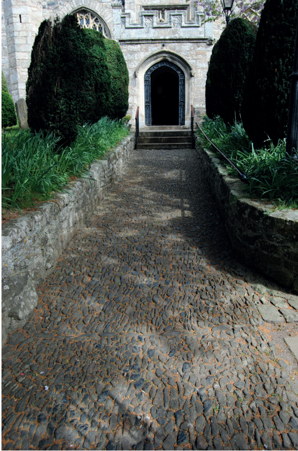
Fig.66. Path drainage here follows the direction of travel of the cobbles making use of a gradient from porch to churchyard boundary.
