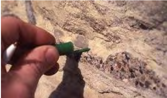
Erosion of exposed historic fabric back beyond previous pointing repair
