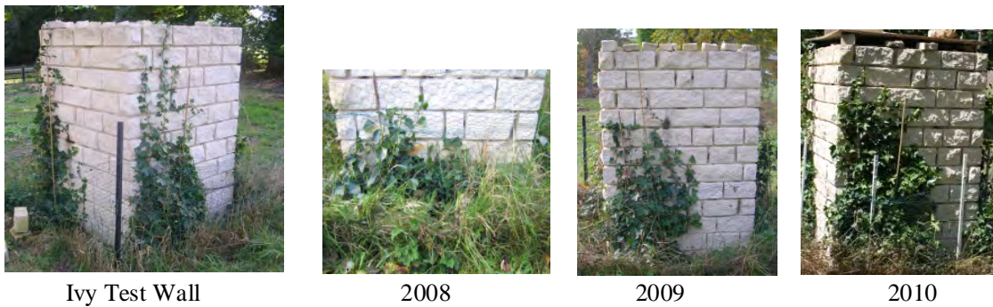
Figure 4.7 Ivy test wall, east face reflecting ivy colonization over time.
