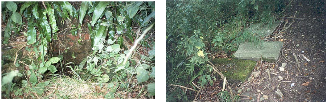
Figure 12: Remains of stone and brick-lined culverts which once took water to the gardens
