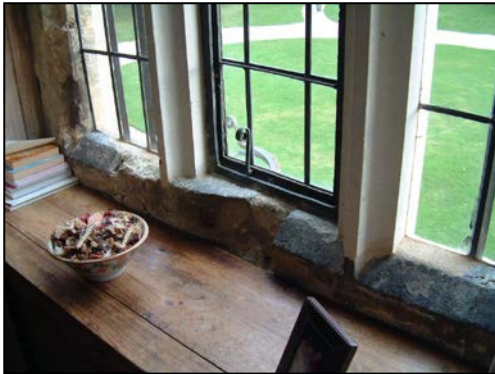
Figure 106. Detail of alterations to window sills and mullions in southern bedroom. (DP004008)
