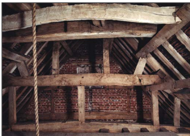
Figure 161. Roof truss on western side of central roof bay. Viewed from east. (AA047430)
