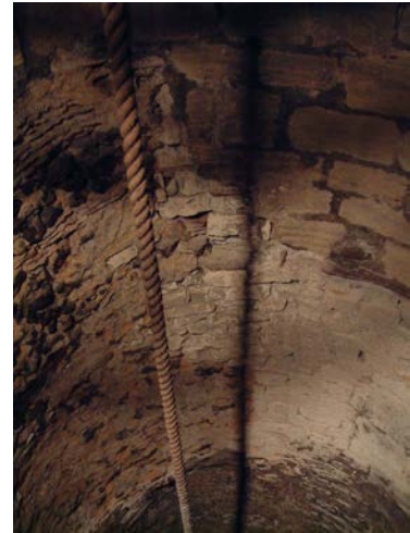
Figure 144. Detail of shaft lining, showing repairs in the masonry, near the head of the well. (DP004014)
