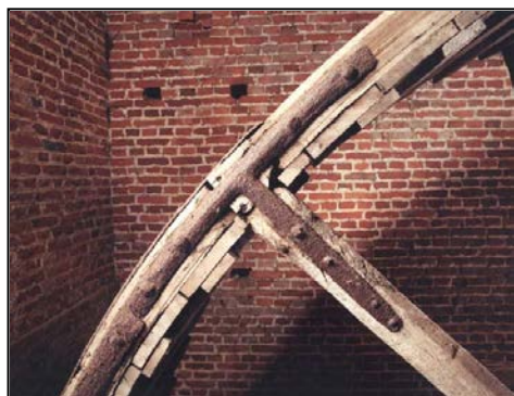
Figure 165. Tread wheel rim. Note spliced timber repairs and later iron straps. (AA047421)
