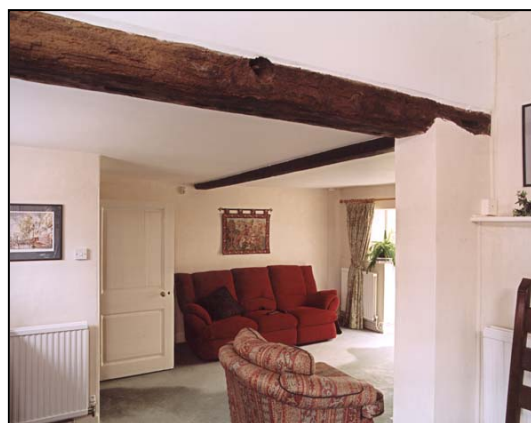
Figure 97. 'The Keep': the living room, viewed from the north east, showing the original beam beneath the central truss. (AA046061)
