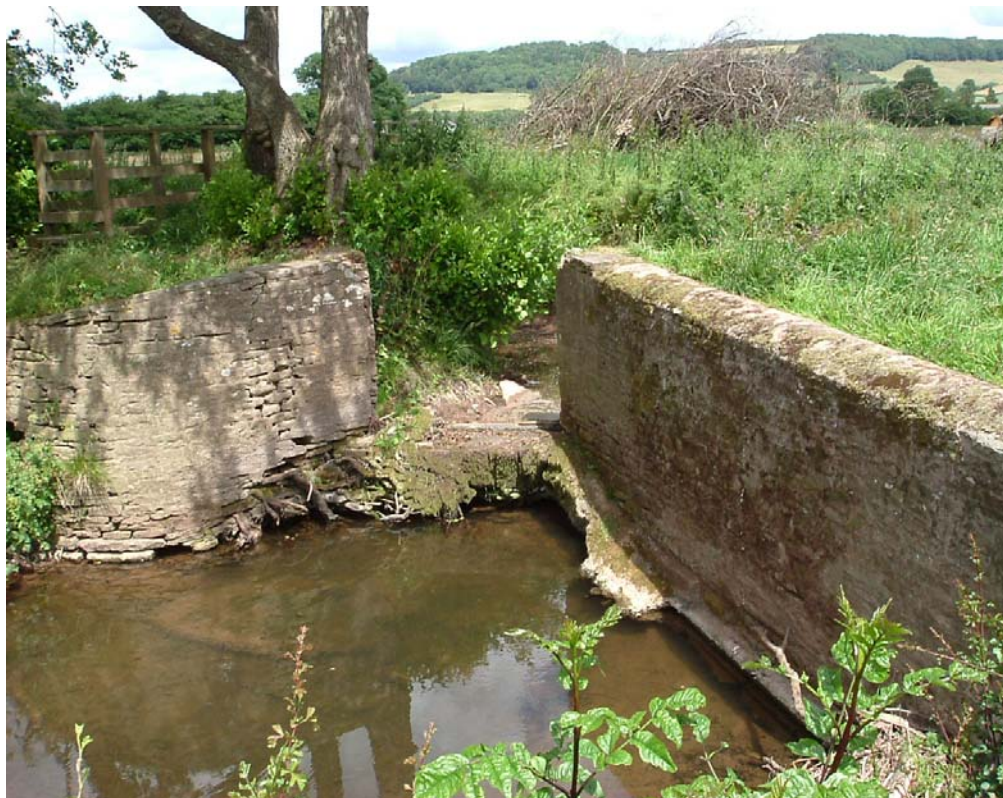
Figure 5: Sluice and weir at (l) on the Slough Brook. Although dry when this photograph was taken, it still carries water for much of the year.
