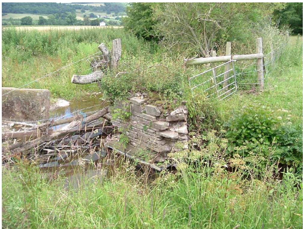
Figure 9: Sluice (q). Remains damaged by tree roots and general decay.
