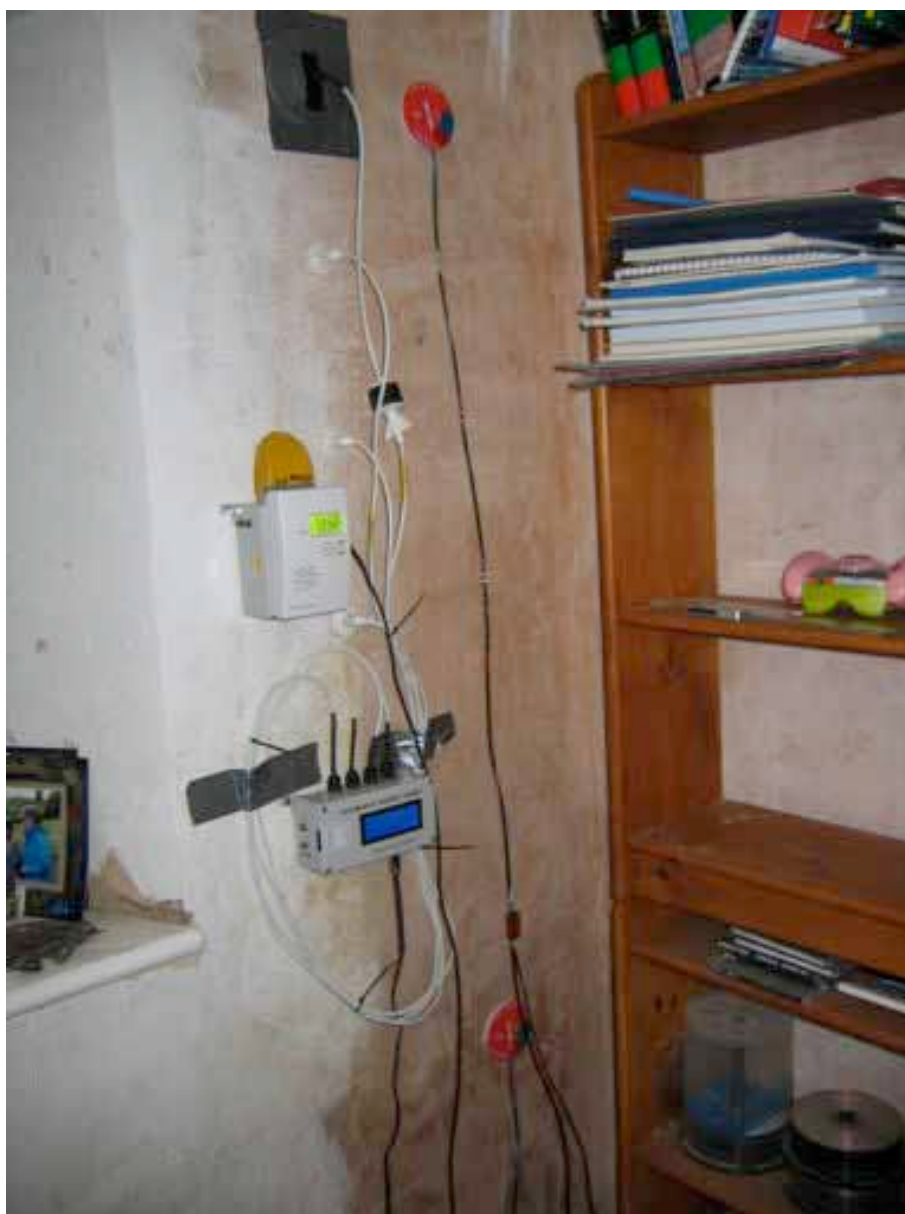
Figure 47. Interstitial, U-value and IAQ monitoring set up at The Firs, Riddlecombe, 2011.
