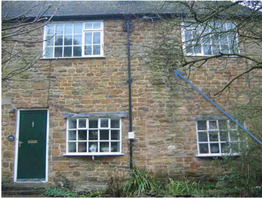
Figure 33. April Cottage, Lower Brailes front elevation showing green staining.
