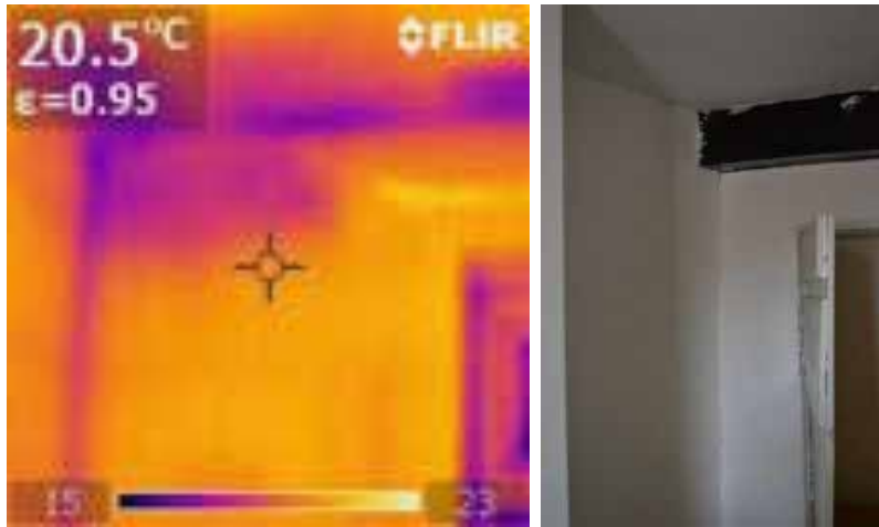
Figure 8. 116 Abbeyforegate, Shrewsbury – second floor, north facing ceiling.
