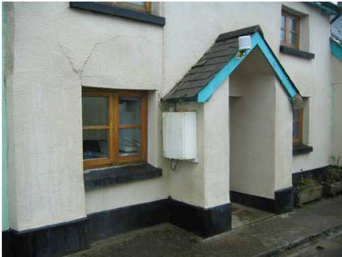
Figure 49. Cracked render at The Firs, Riddlecombe, 2011.
