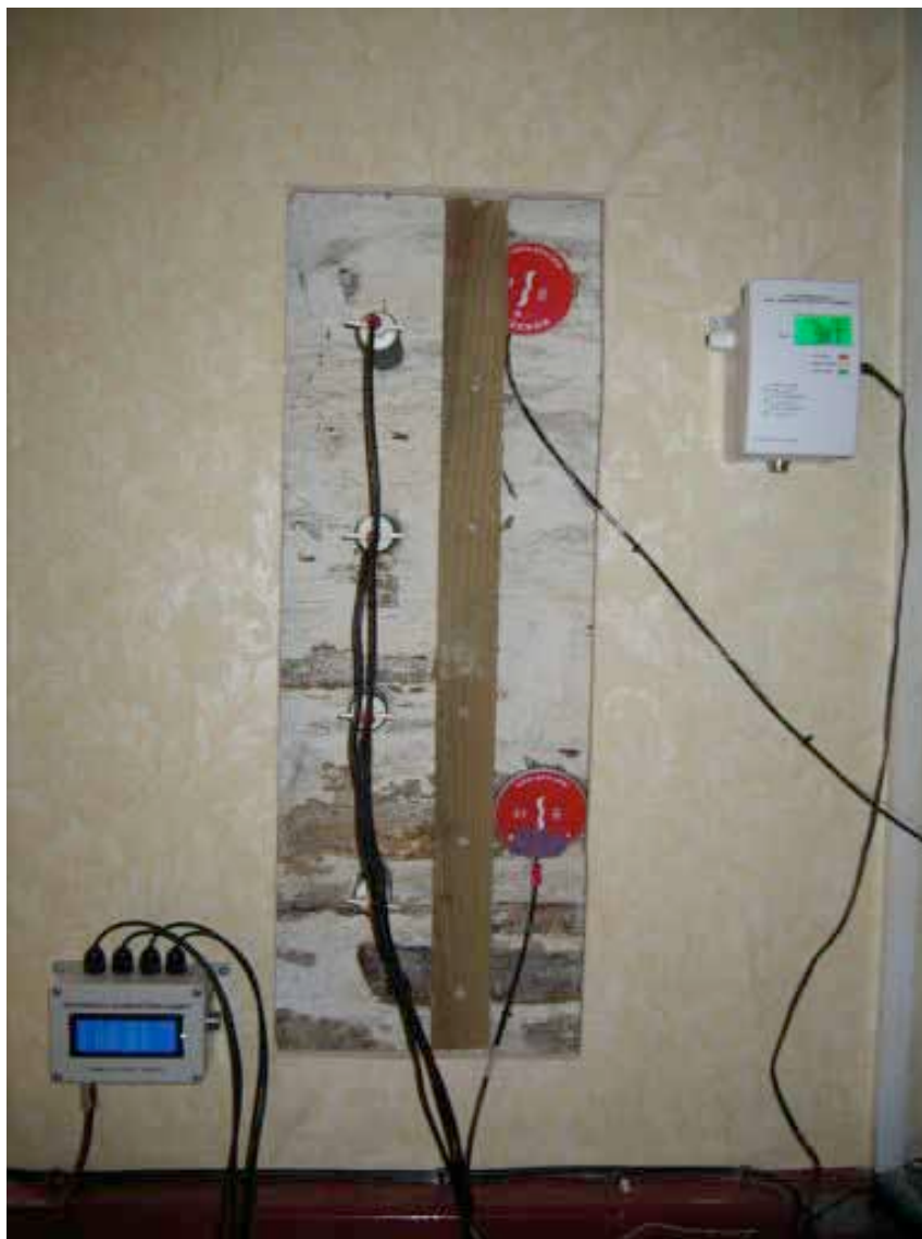
Figure 77. Interstitial, U-value and IAQ monitoring set up at Rock View, Devon Consuls, 2011.
