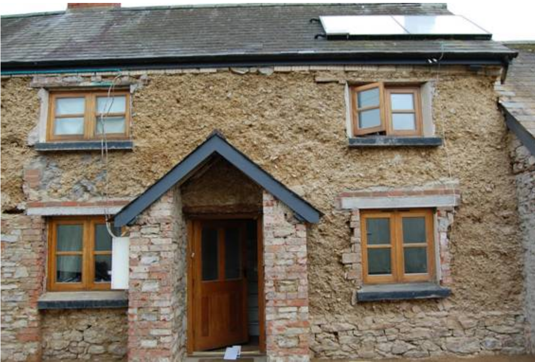
Figure 76. The Firs, Riddlecombe front elevation showing masonry buttress bottom left of frame.
