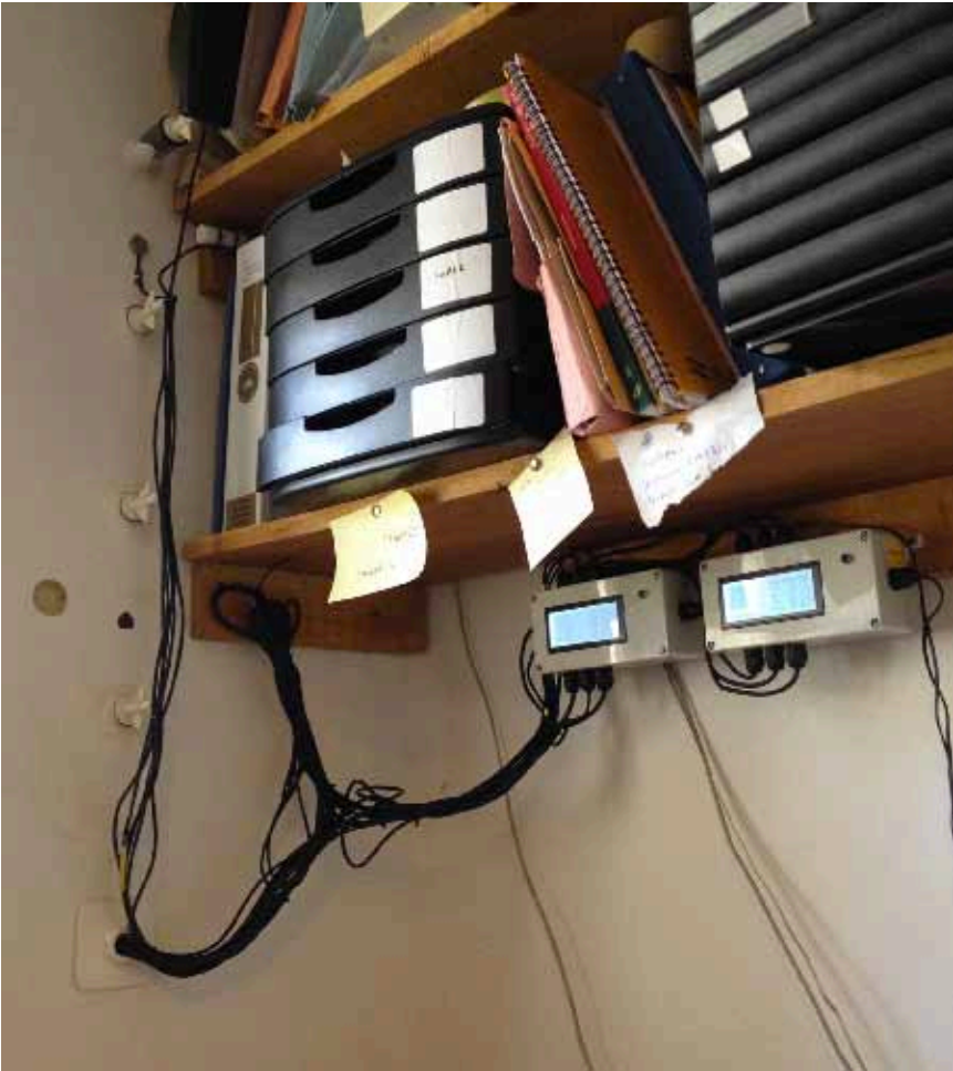
Figure 26. Interstitial Hygrothermal Gradient and Material Moisture Monitoring, Riddlecombe.
