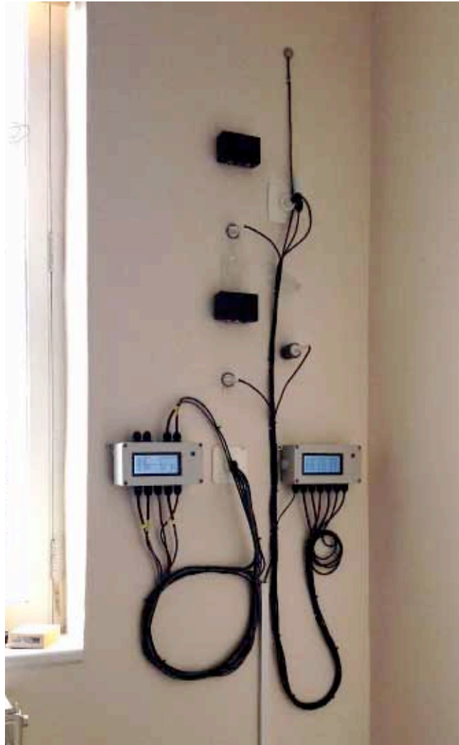
Figure 3. Interstitial hygrothermal gradient and material moisture monitoring, Shrewsbury.
