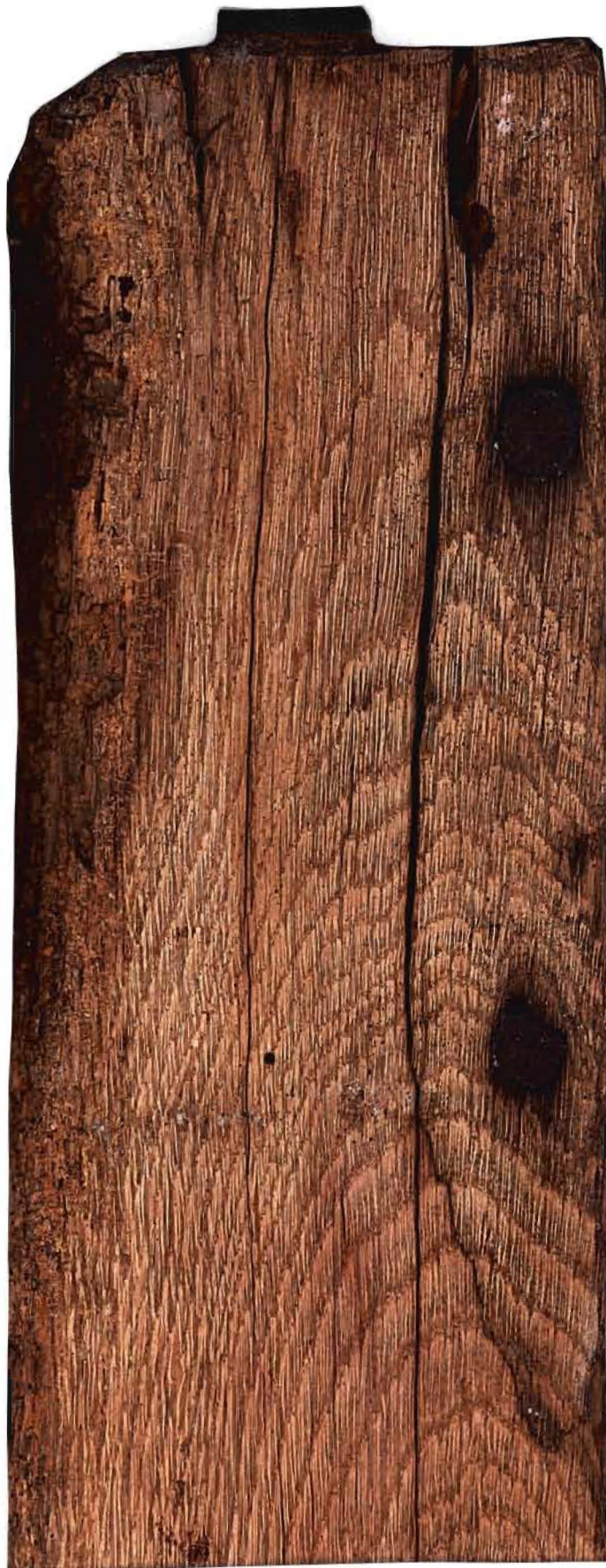
Figure 26: Upper end of south soulace brace of truss 19, St Stephen's (South) Chapel roof, showing two original nails repairing the shoulder damaged during erection (75%)
