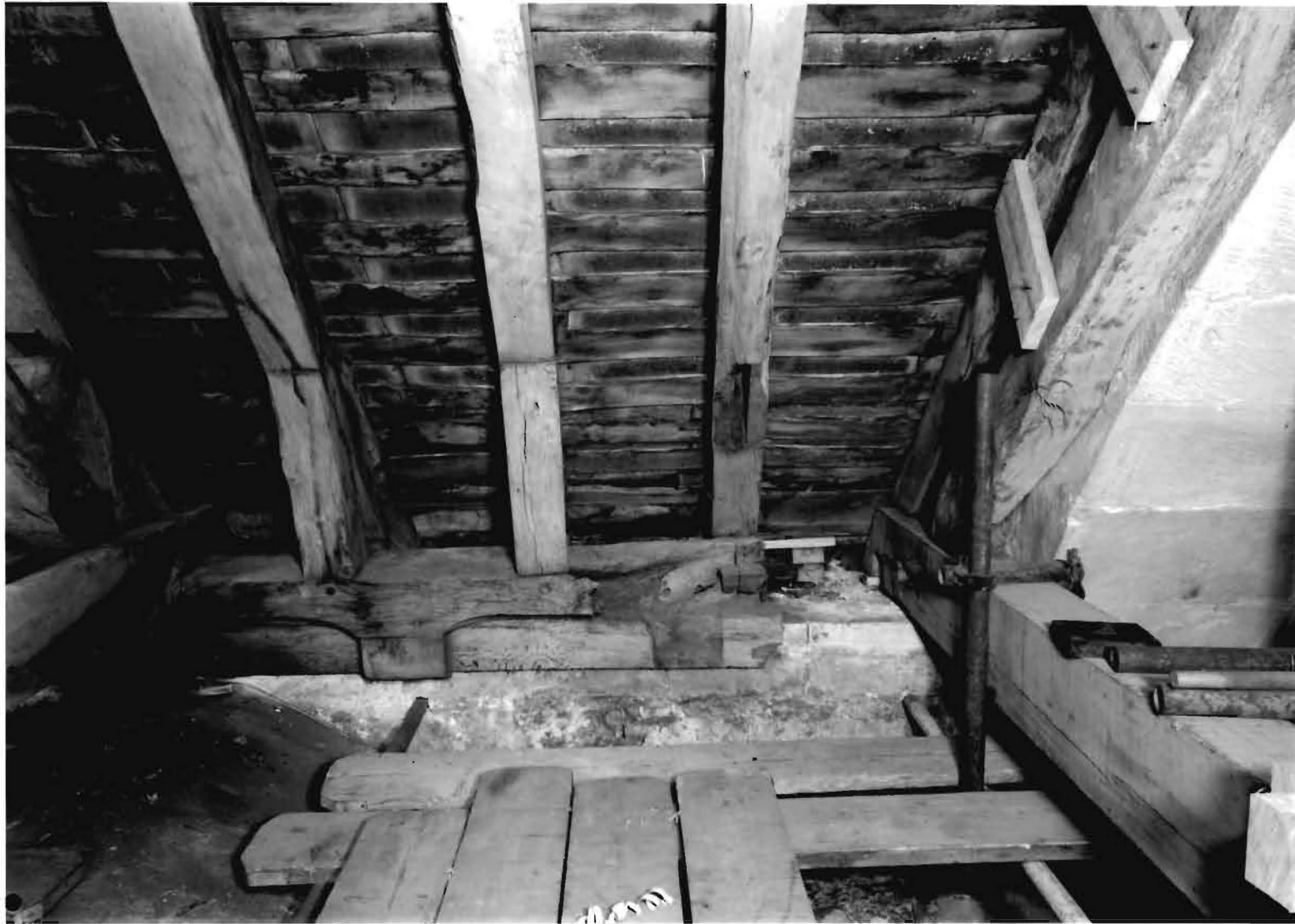
Figure 19: North nave triforium wallplates and roof sarking boards. © Crown copyright. NMR. BB69/4393
