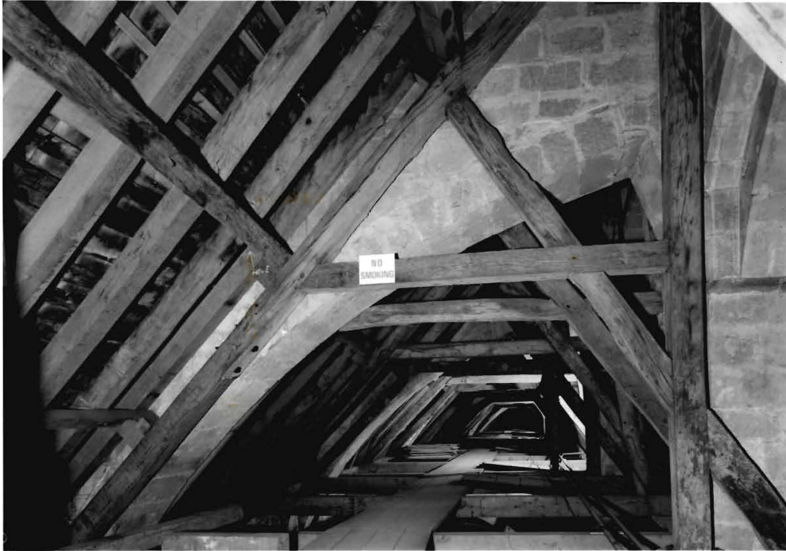
Figure 16: North nave triforium looking east showing truss 2 west. © Crown copyright. NMR. BB71/2660
