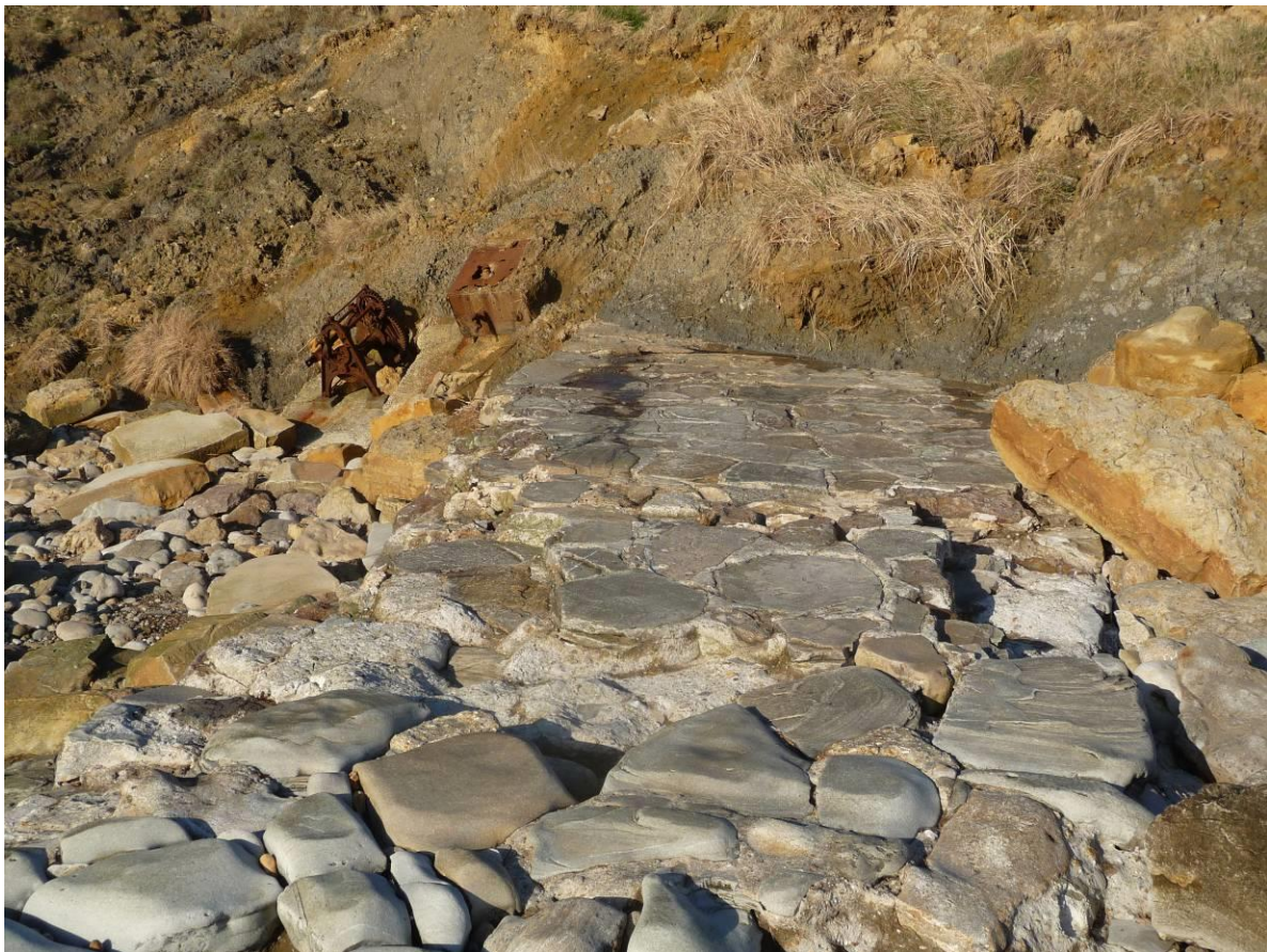
Fig 6.4 A slipway at Osmington, partly covered by coastal collapse (Photograph: Graeme Kirkham).
