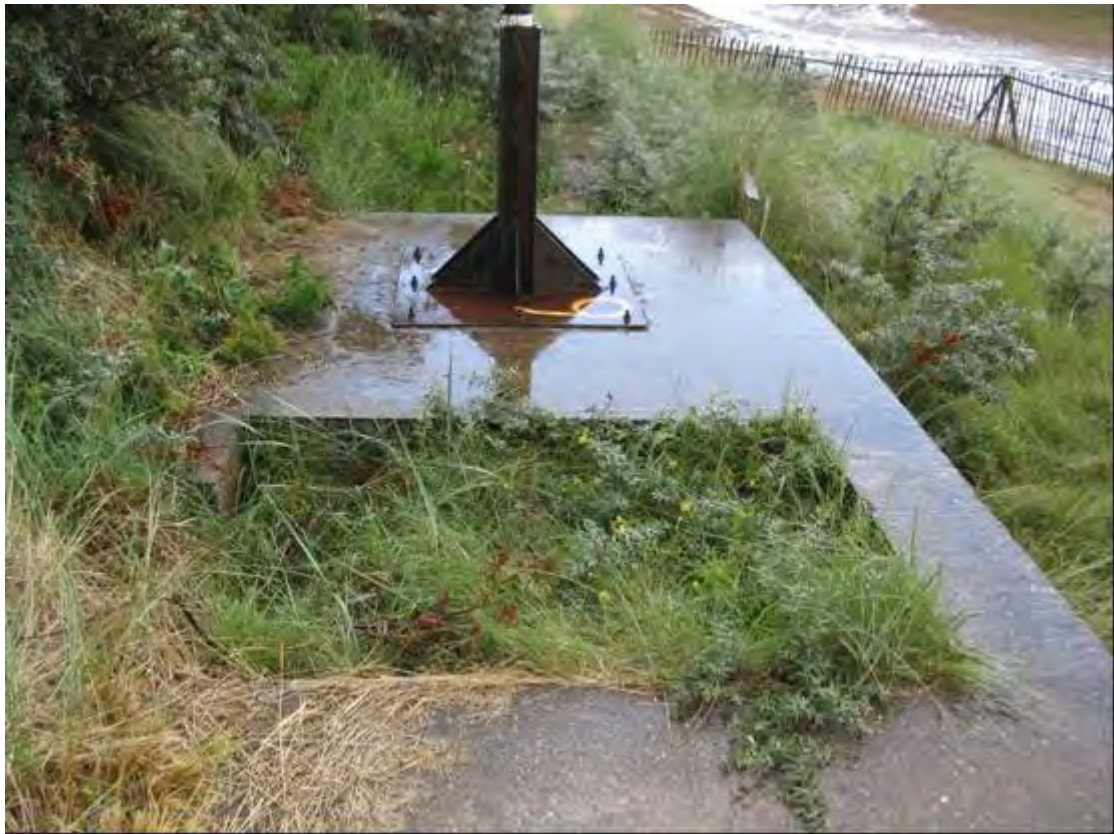
Plate 3 Infilled AA gun pit in roof of WW2 pillbox NS12, North Somercotes
