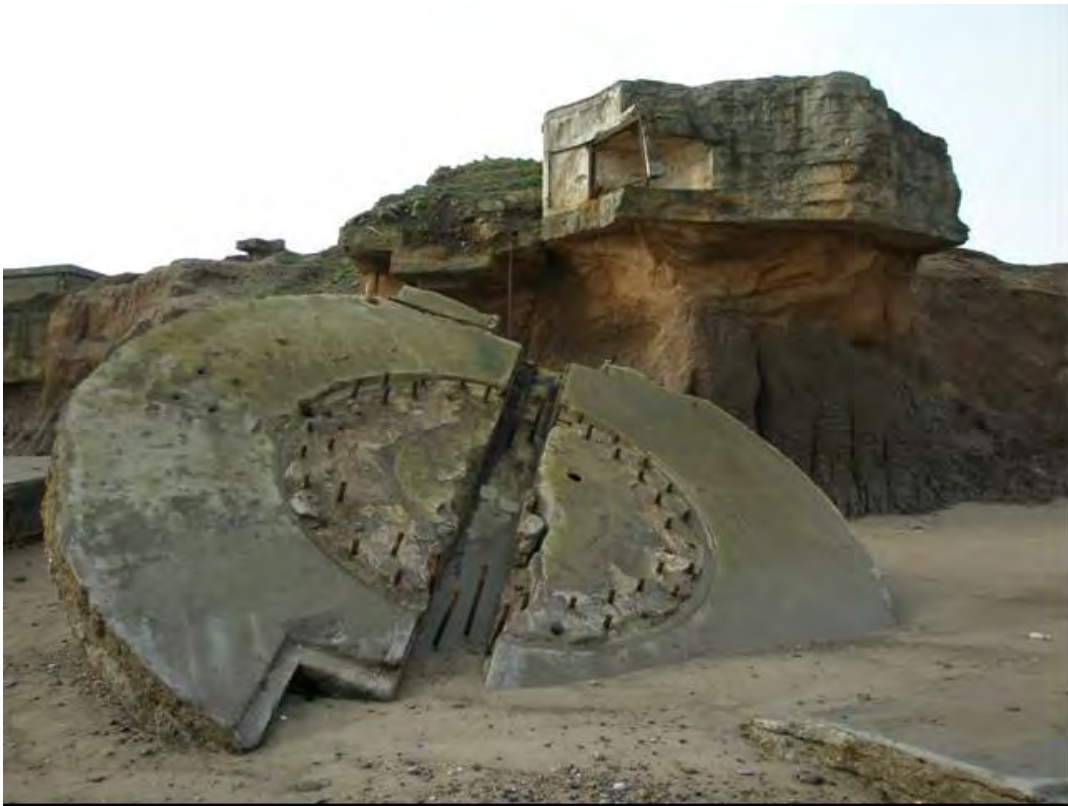
Plate 25 Collapsed 9.2in gun platform and precariously-balanced formerly-adjoining building, Godwin Battery, Easington (EA182), looking west
