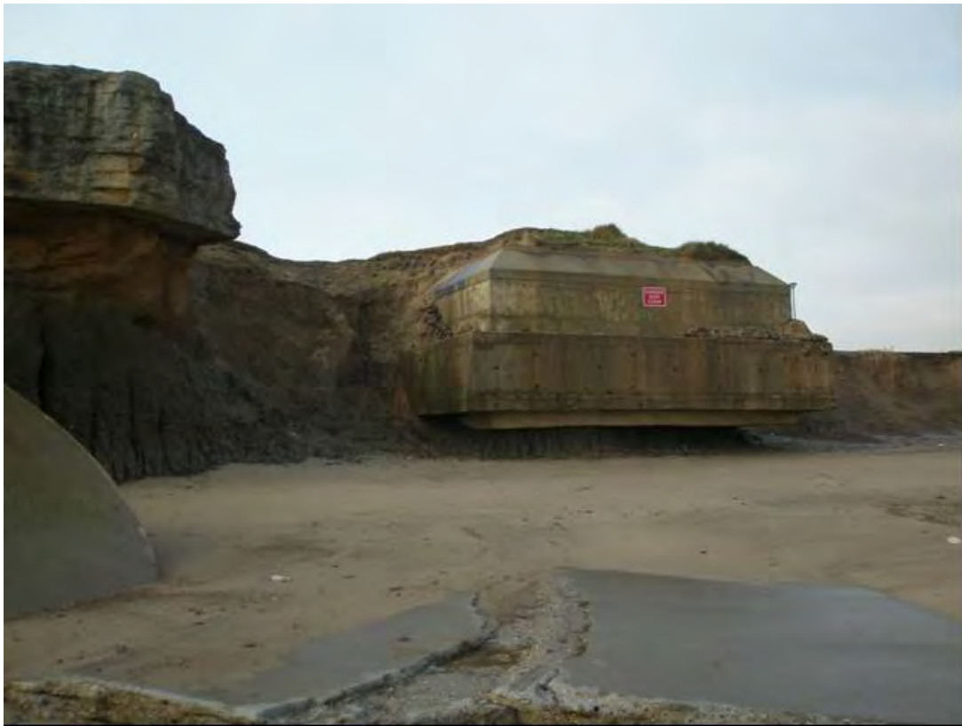
Plate 24 Undermined magazine, Kilnsea Battery, Easington (EA182)
