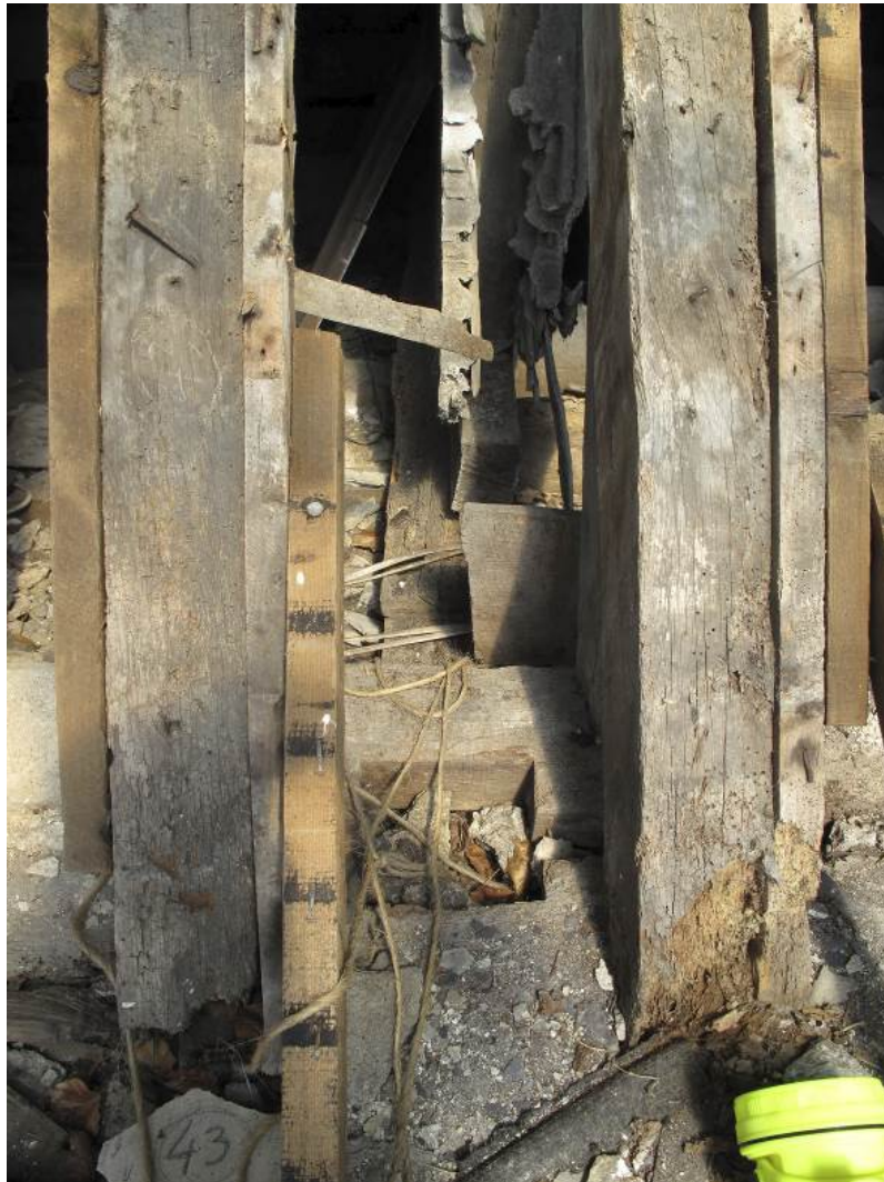
Fig 27 The cuts in the wall plates between trusses 42 (right) and 43 (left) on the south side of the roof. West is to the left. Photo: Rebecca Lane.
