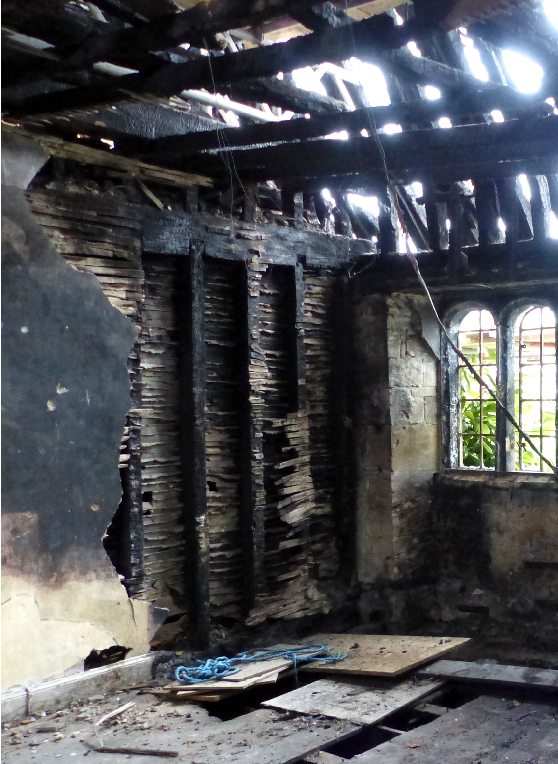
Figure 33 The partition between the two easternmost first-floor rooms (K on Fig 10) viewed from the north west. Photo: Helen Winton
