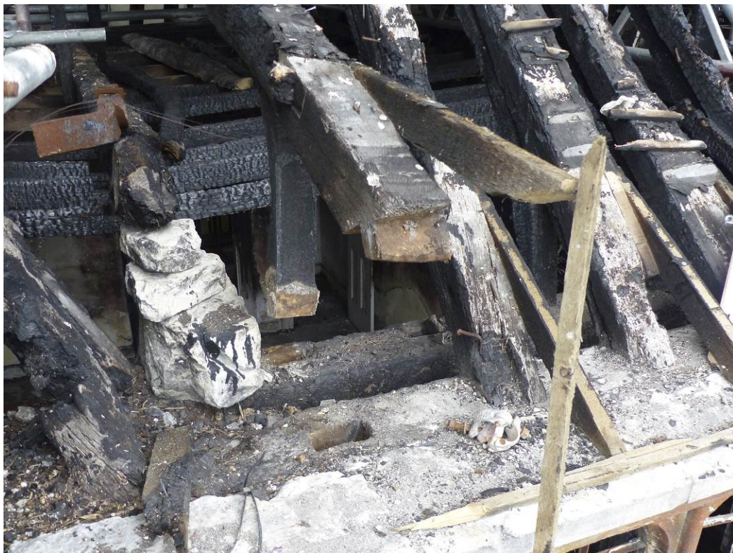
Fig 18 Truss 21 on the south side showing the mortices in the wall-plates and the tenons in the rafter and lower brace. Photo: Helen Winton.
