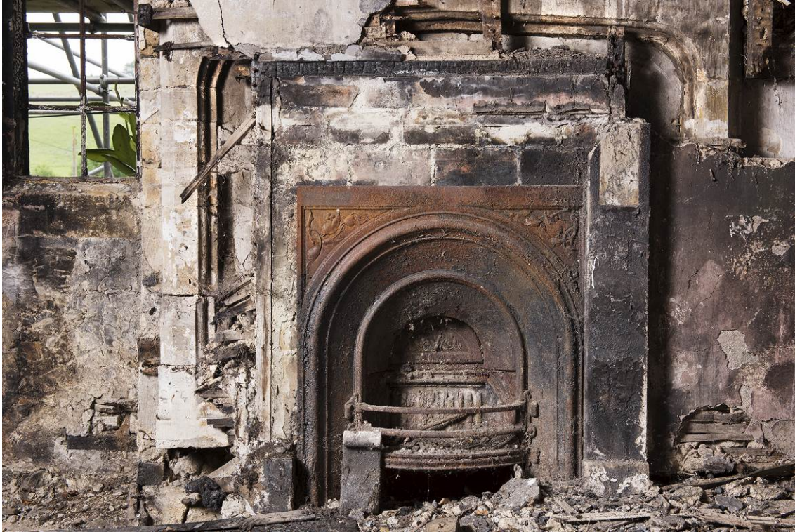
Fig 15 The 16th-century fireplace behind plaster and a 19th-century fire surround on the first floor. HEA DP196753.
