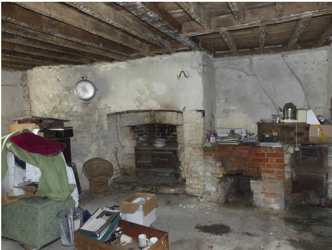
Fig 35 Interior of the ground floor of the south wing, looking south. Photo: Helen Winton.
