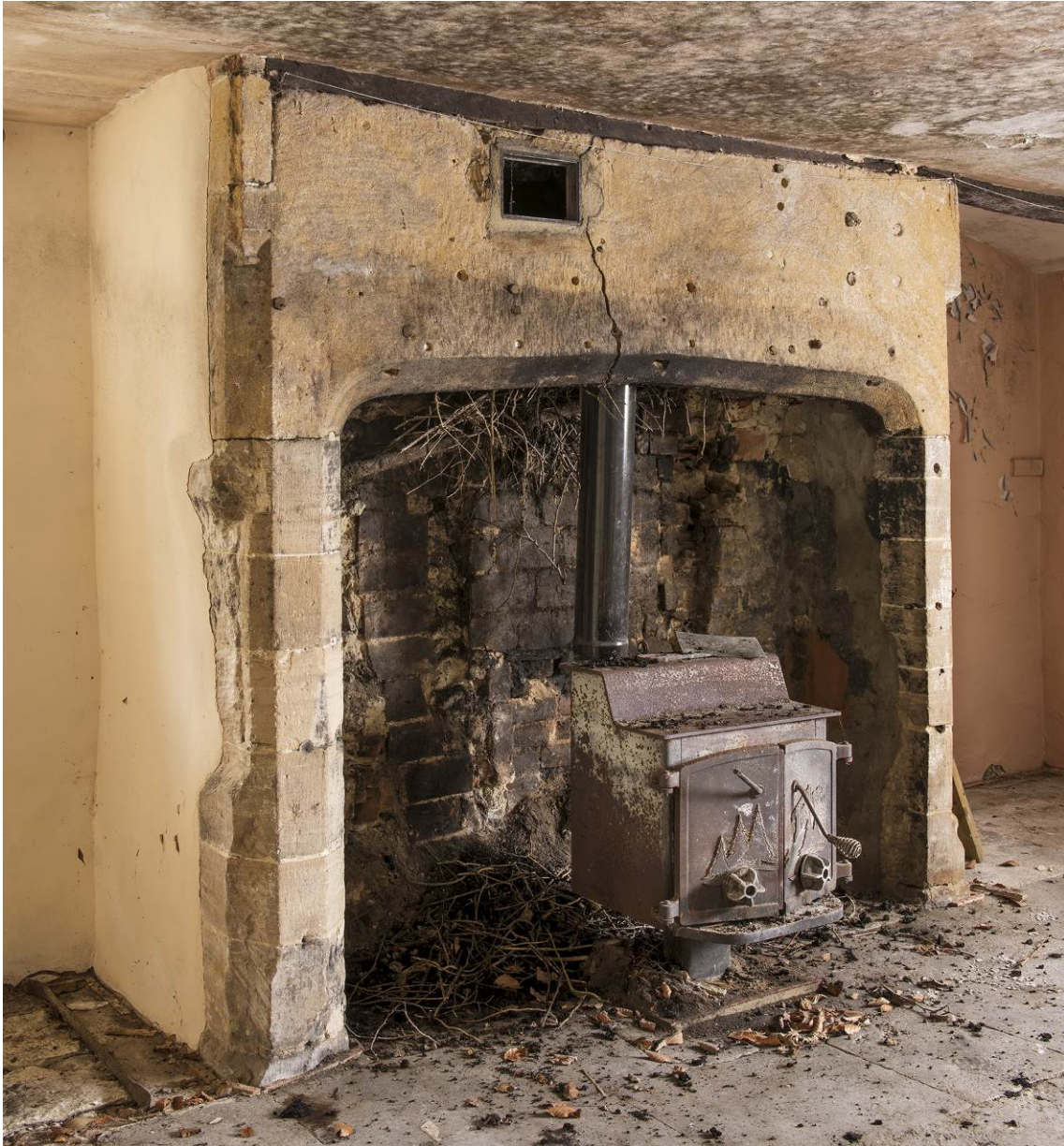
Fig 32 The fireplace on the ground floor at the west end of the house. HEA DP196746.
