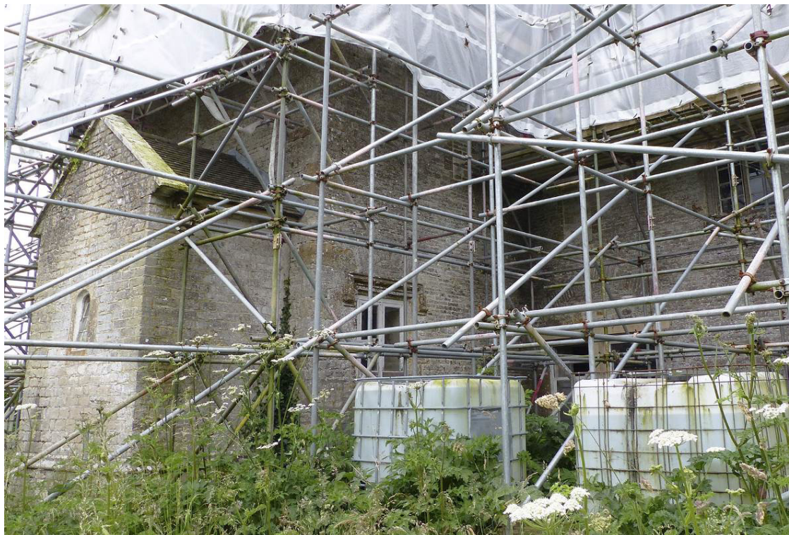
Fig 30 The west elevation of the north wing showing the position of the window between ground and first-floor level. The bottom of the blocked window above first floor level is just visible centre-right near the top of the frame. Photo: Helen Winton.
