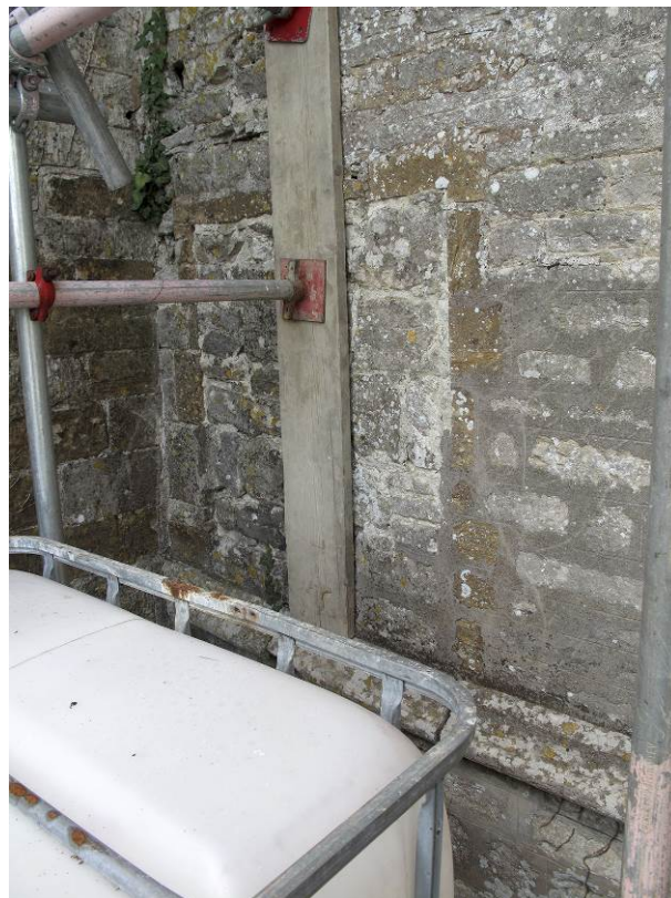
Fig 24 The blocked window on the ground floor where the south elevation of the main range meets the south wing. Photo: Rebecca Lane.
