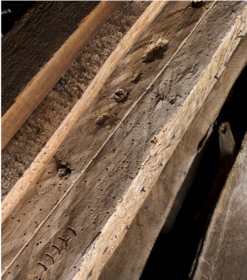
Fig 26 View of the fair (east) side of truss 41 on the south side of the roof over the main range. HEA DP 196787.
