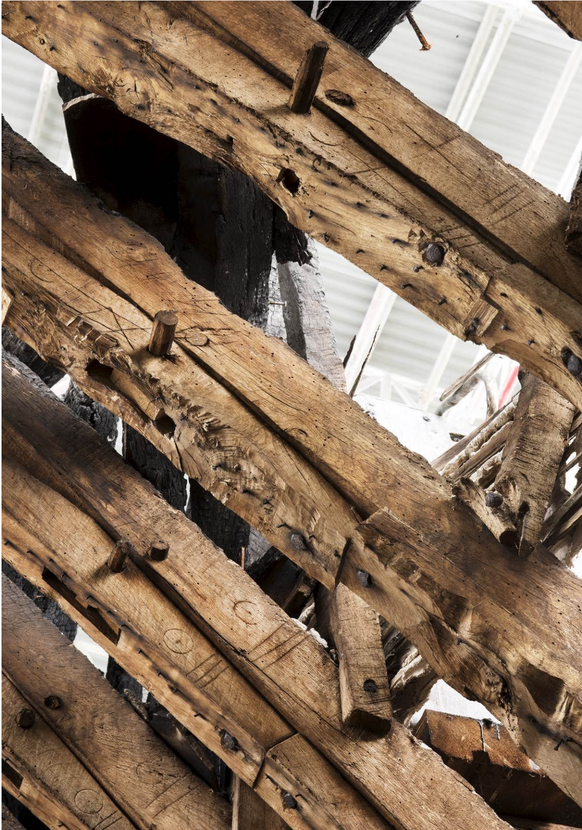
Fig 21 Looking west at the upper braces and rafters on trusses 11 to 14 on the south side of the roof. The underside of the upper braces on trusses 12 and 13 have been cut back, revealing the slip tenon in the joint between the rafter and brace. HEA DP196757.
