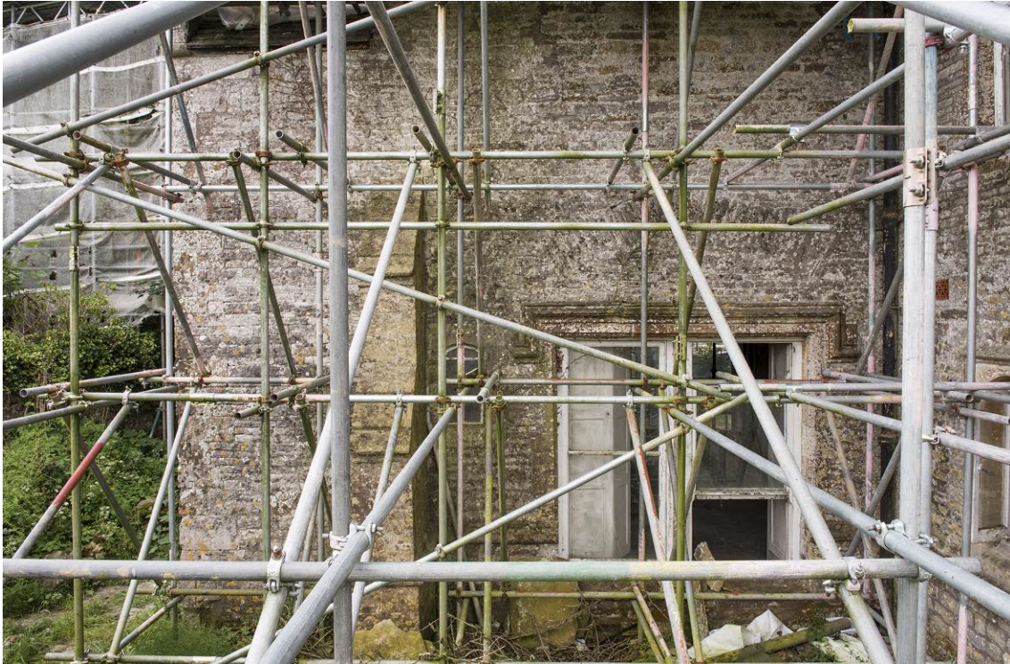
Fig 11 The east end of the north elevation. The roof of the stair tower is just visible top left of frame. The ground-floor window in the main range has been altered but the relieving arch above shows it is an original opening. HEA DP196818.
