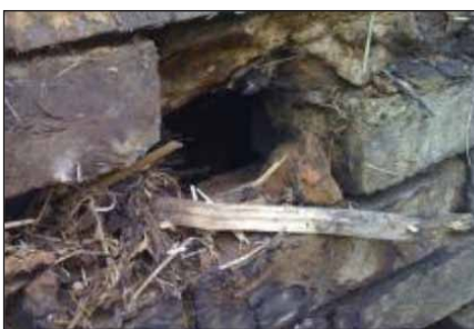
Figure 36. Liner found to be in contact with chimney brickwork.
