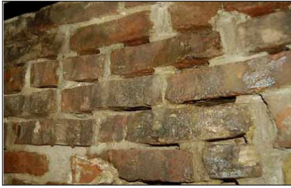
Figure 33. Imperfect mortar in brickwork.
