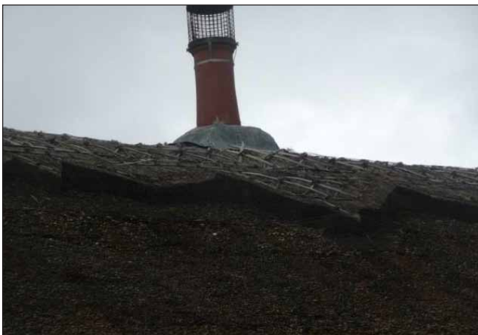
Figure 28. Thatched property with very small pot top to thatch clearance. Figure 29. Long-pot used to increase thatch to pot top clearance.
