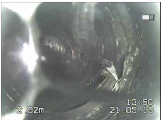
Figure 32. Split chimney liner.
