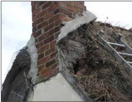
Figure 34. Thatch by imperfect chimney brickwork.
