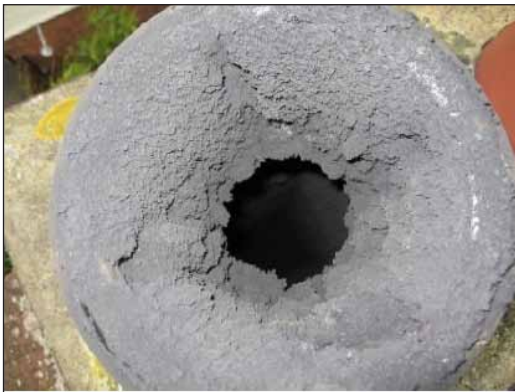
Figure 31. Chimney sweeping annulus.
