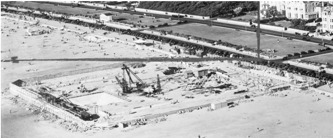
Figure 24 Swimming pool under construction in 1936. Note the deep depression on the left of the crane designed to hold sufficient water for diving. The dark lines across the top were drawn on the original print. Detail of AFL 60897/EPW051725 Aug-1936 © Historic England (Aerofilms Collection)
