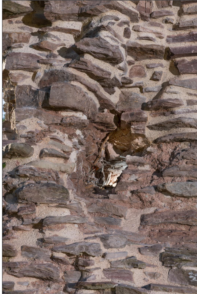
Figure 14 The empty slot in the east wall of the so-called 'hall block' (DP220714).
