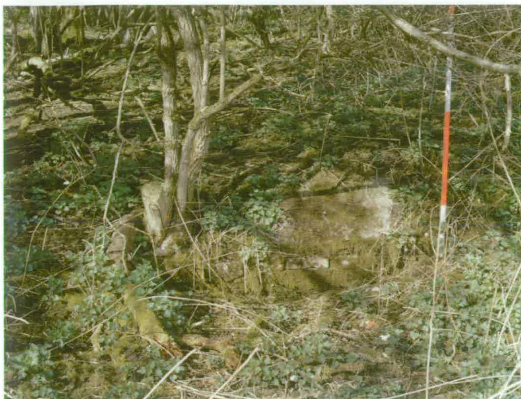
Plate 7: Brick-built and concrete capped drain or culvert on the southern flank of Dovecote Close.
