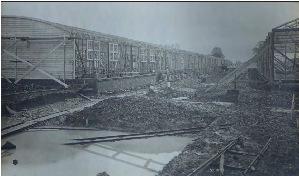
Fig. 4.20. NFF No. 5 Quedgely under construction, 1915. View looking north along the central axis of the site with component stores to the left and assembly huts on the right (TNA MUN5/157).
