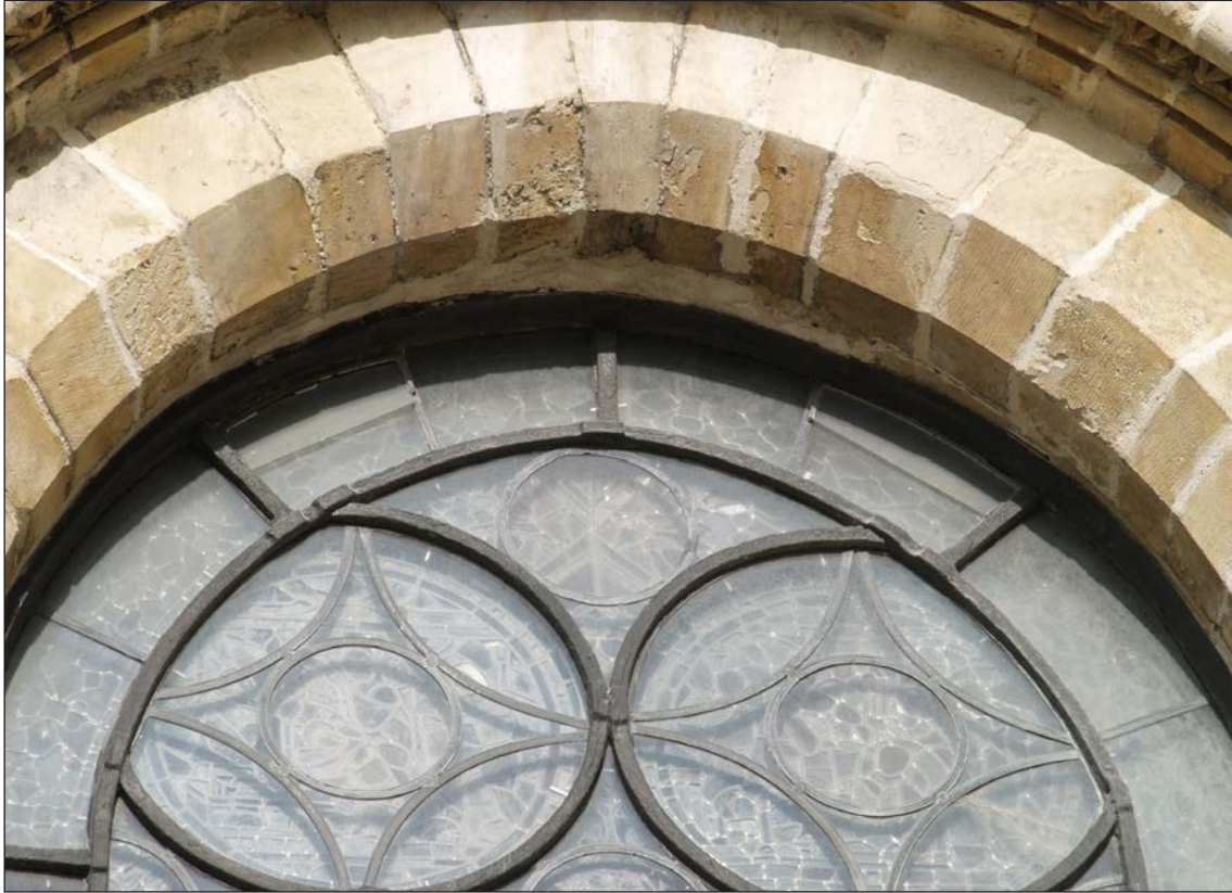
Figure 25. Ventilation openings at the top of an externally vented system installed in 1979 at Canterbury Cathedral.
