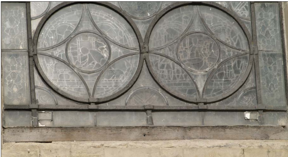
Figure 24. Ventilation openings at the bottom of an externally vented system installed in 1979 at Canterbury Cathedral.
