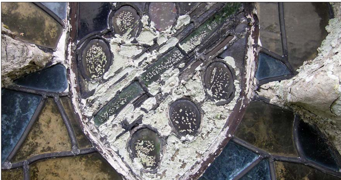
Figures 17, 18. Microbiological attack is both unsightly and can cause chemical deterioration of the glass as well as retaining moisture. Damage can occur internally as at Norbury in Derbyshire (top) or externally as at Boughton Aluph in Kent (bottom, ©Léonie Seliger).
