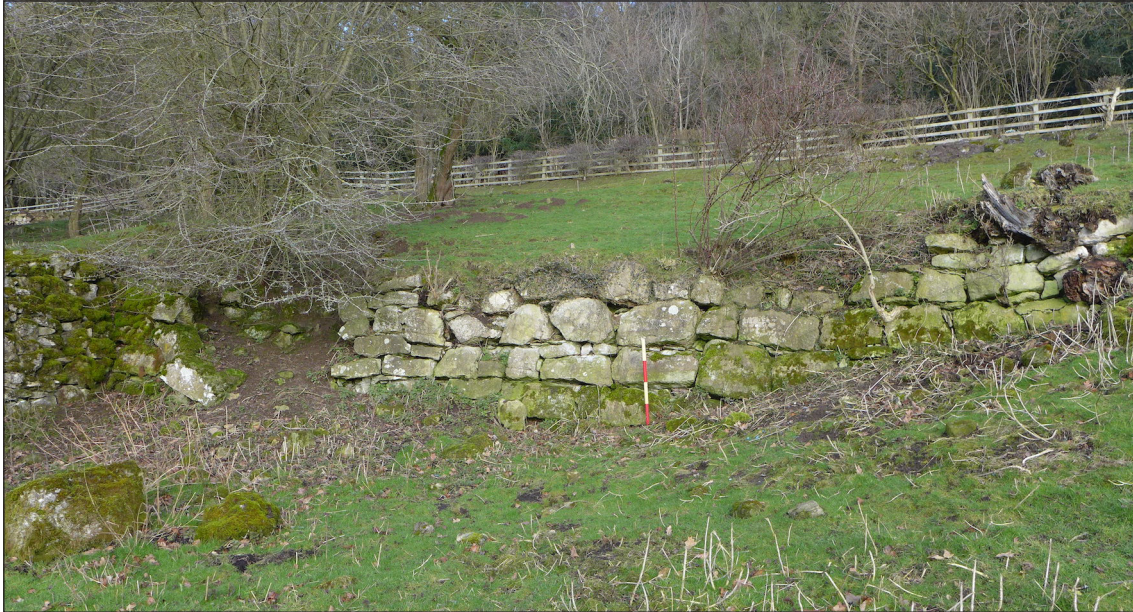
Fig 30. View looking north-east of the stone wall revetting part of the upper terrace, February 2018. © Historic England.
